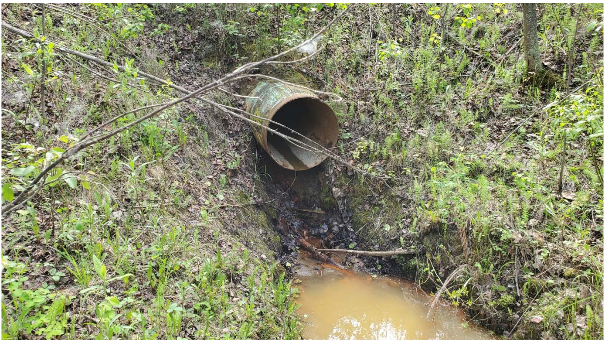
Photo 6 – Hanging culvert outlet.
