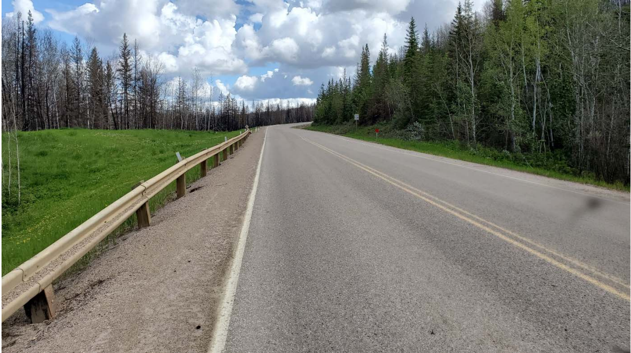
Photo 1 – Looking northeast at hump in the highway.
