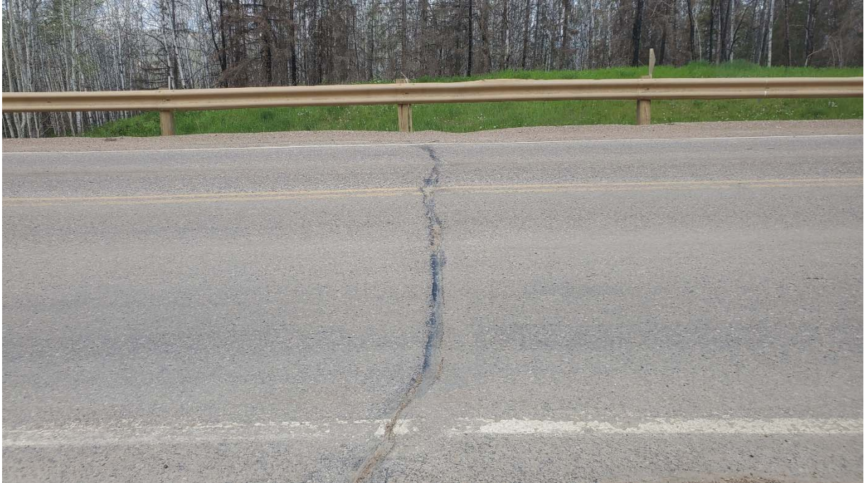
Photo 3 – Looking northwest at crack at northeast end of embankment fill.
