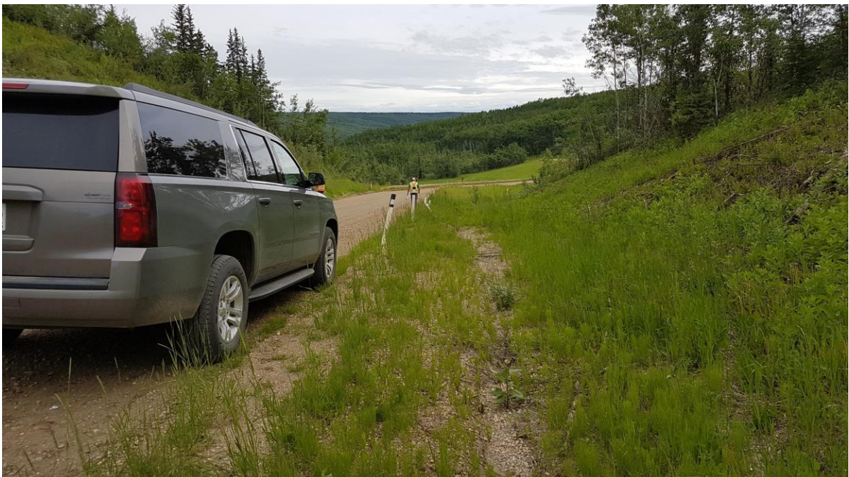
Photo 2 – Looking north at east ditch erosion at the south end of the site (km 42.4).
