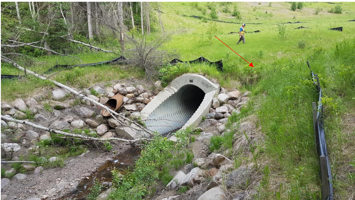
Photo 6 – Looking northwest at culvert inlet. Note erosion to right of culvert above the riprap (red arrow).
