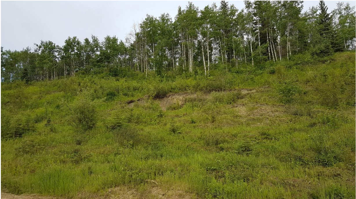
Photo 1 – Looking west at backslope failures at the south end of the site (km 42.4).
