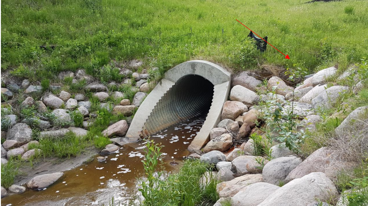
Photo 7 – Looking southeast at culvert outlet. Note erosion below the riprap on the right side of the culvert (red arrow).
