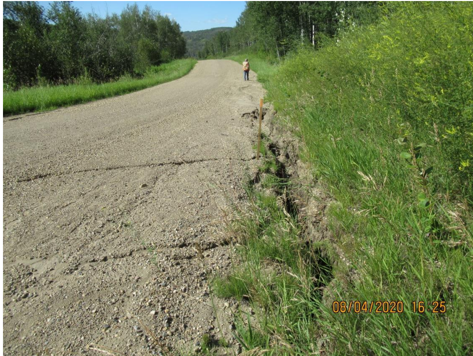
Photo 3 – Looking north along backscarp crack.
