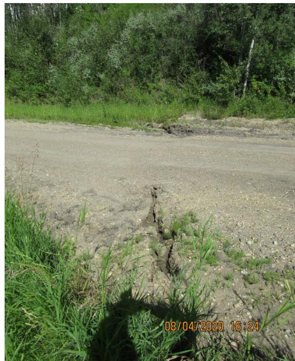
Photo 2 – Scarp crack crossing road
