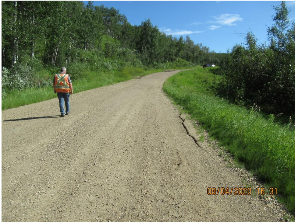
Photo 5 – Looking south toward the landslide.
