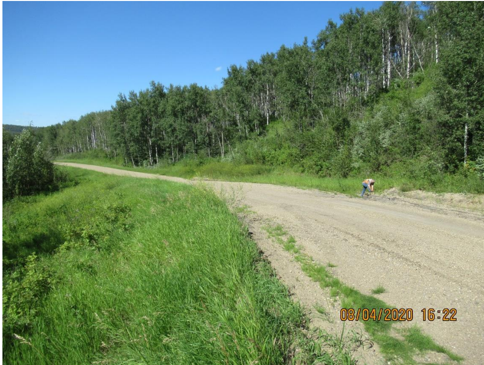
Photo 1 – Looking north at landslide site.
