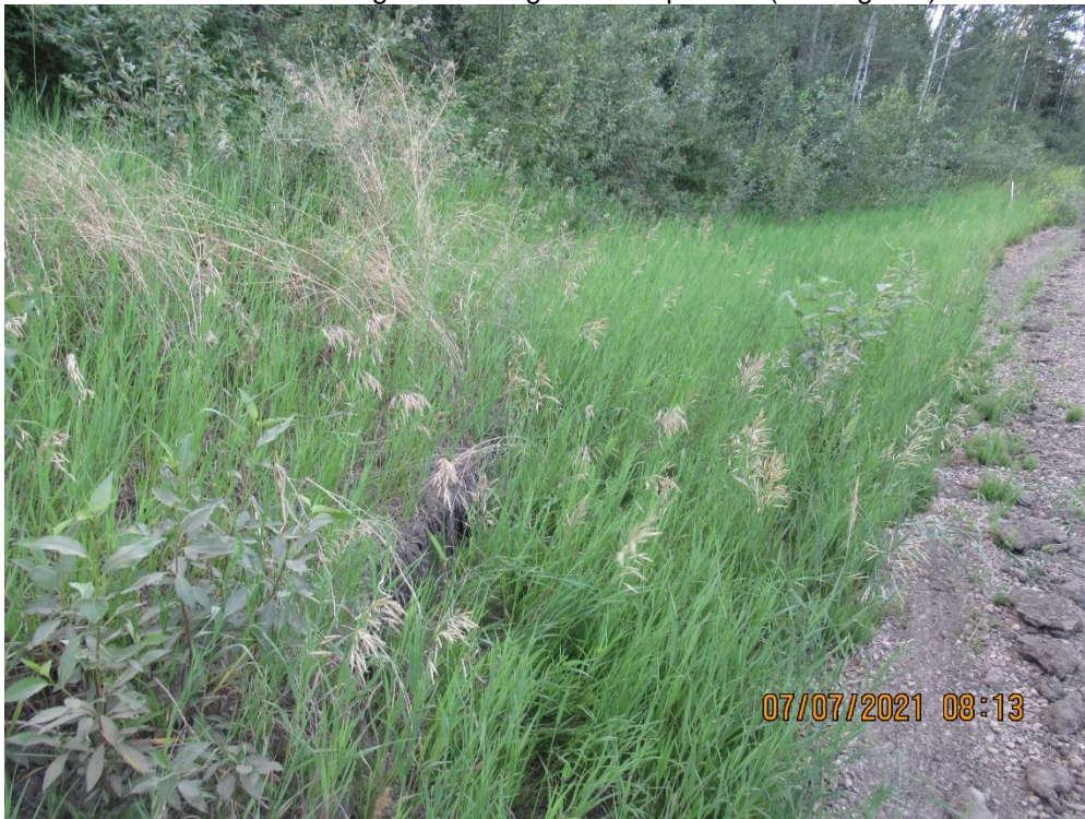
Photo 4 – Looking south at open crack along backscarp of slide at edge of highway.
