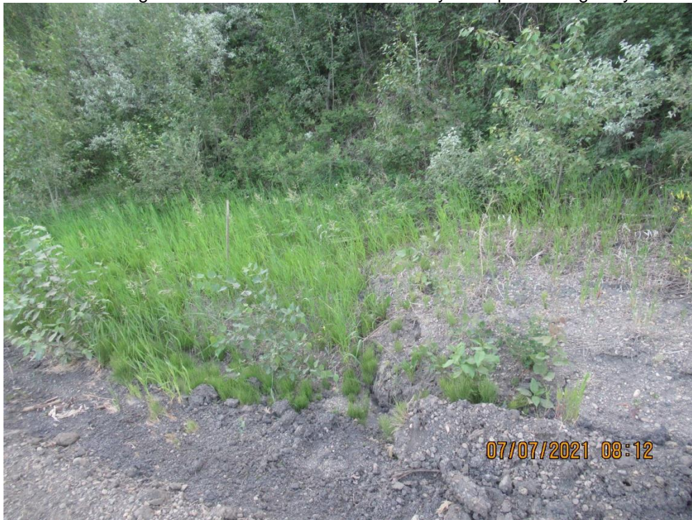
Photo 2 – Scarp crack at the edge of the road
