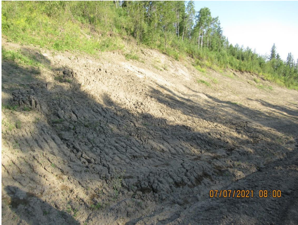
Photo 7 (PH011-1) – Shallow slump forming at south end of the PH011-1 backslope regrading.
