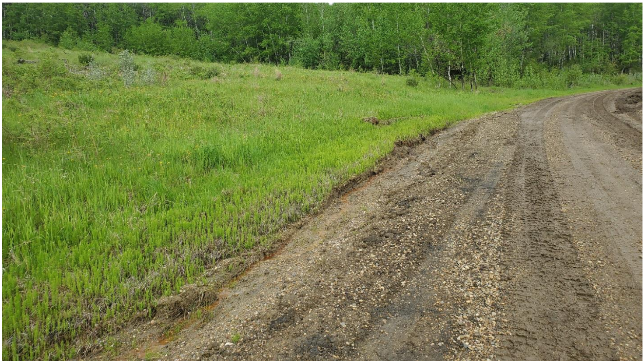
Photo 8 – Looking at seepage along west side of road near the north end of the site.
