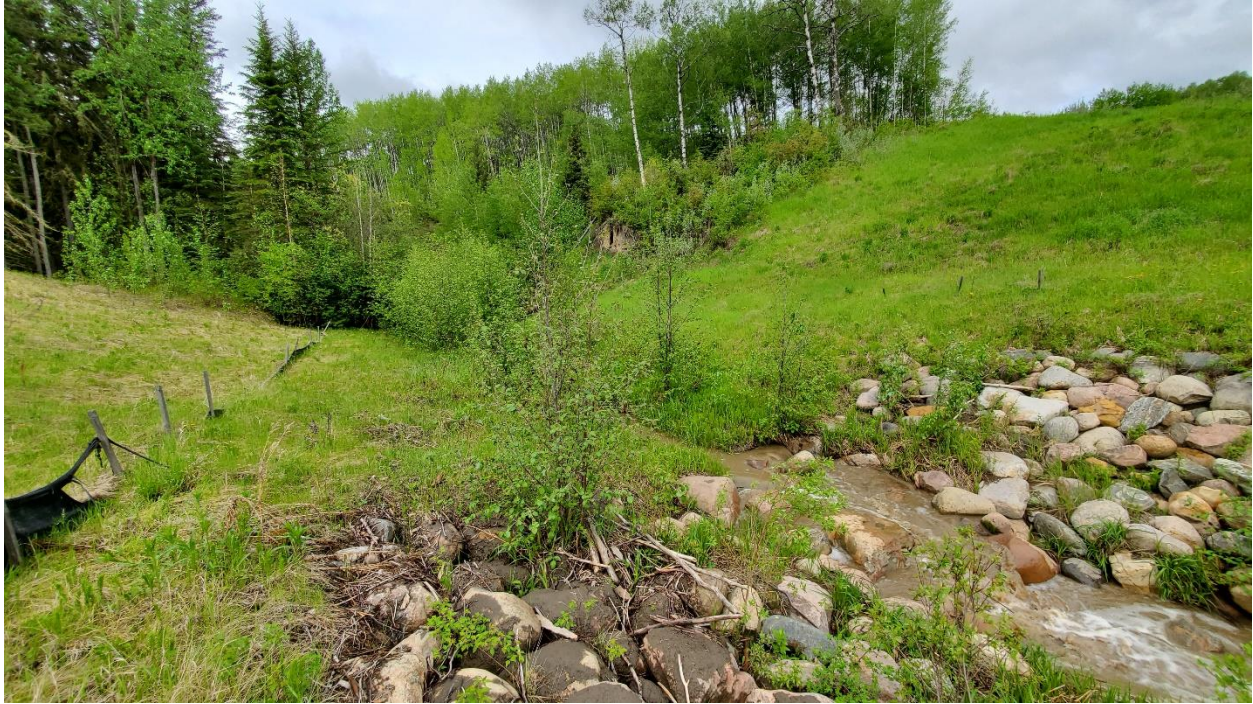
Photo 7 – Looking west at shallow slumps on backslope at culvert inlet.
