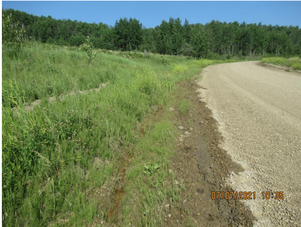
Photo 7 – Looking at seepage along west side of road near the north end of the site.
