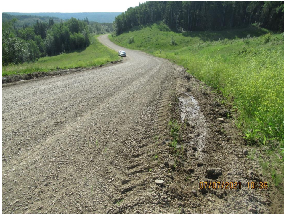
Photo 6 – Looking southeast at road and seepage along south ditch.
