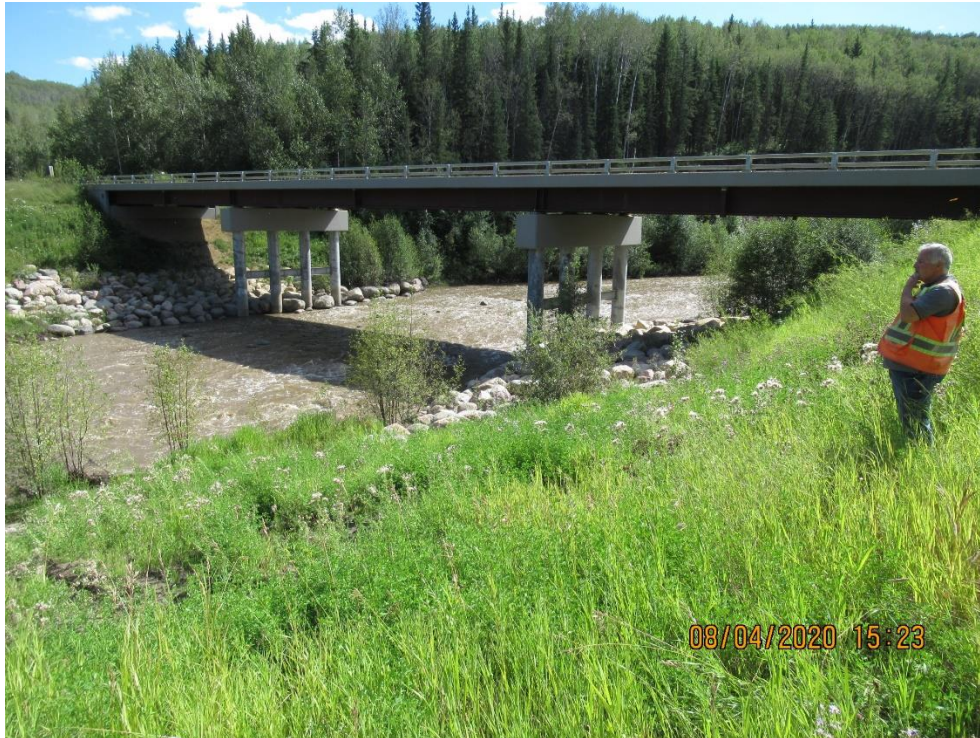
Photo 5 – Run off from ditch erosion went down the riverbank at this location.
