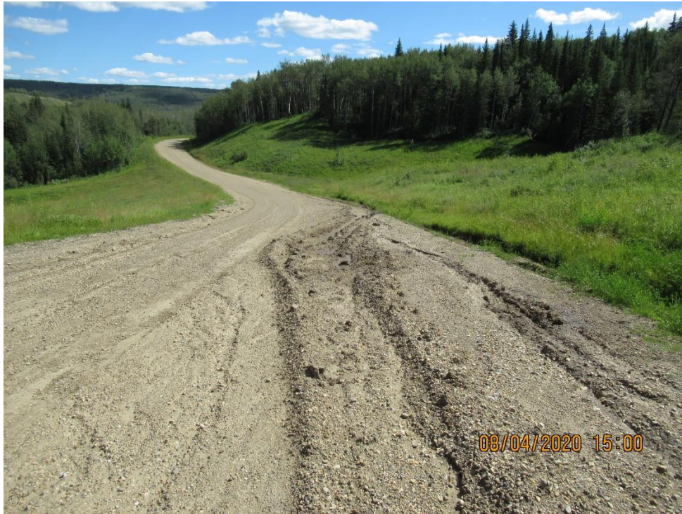
Photo 1 – Looking south at seepage and rutting in road surface at PH038.
