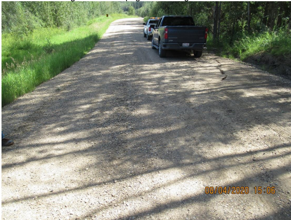
Photo 2 – Looking south at north end of PH075-2 slide
