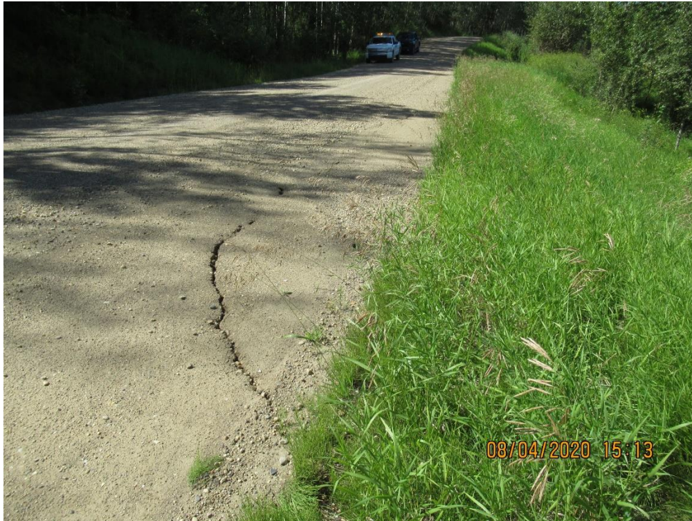
Photo 3 – Looking north along scarp in highway shoulder at south end of PH075-2 Site.
