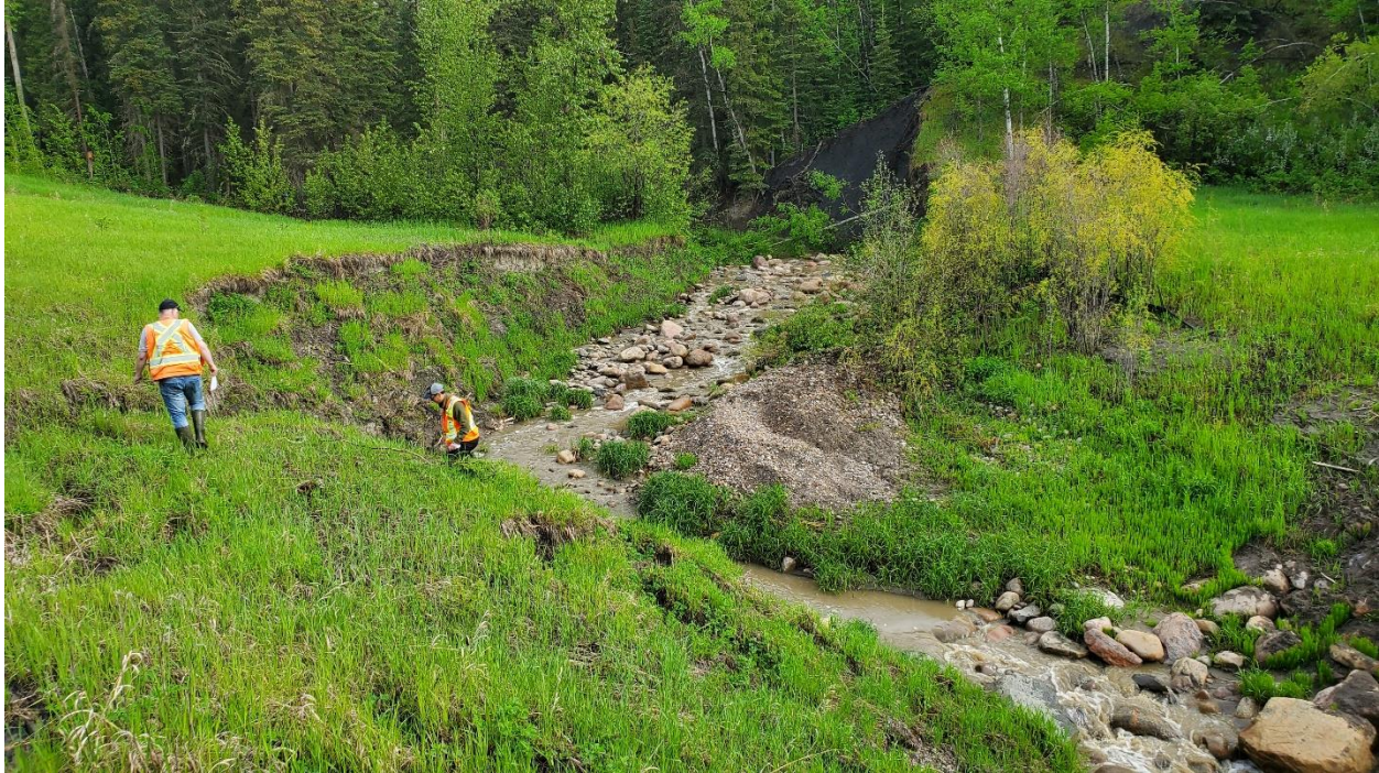
Photo 3 – Looking north at creek bank slumping upstream of the culvert inlet. Note fresh material deposits on the right-hand side of the channel.
