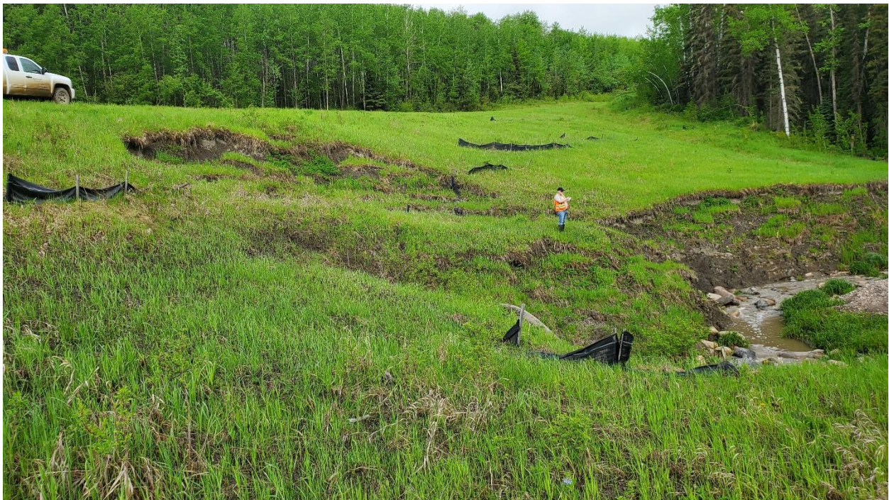
Photo 2 – Looking northwest at creek bank slumping upstream of the culvert inlet.
