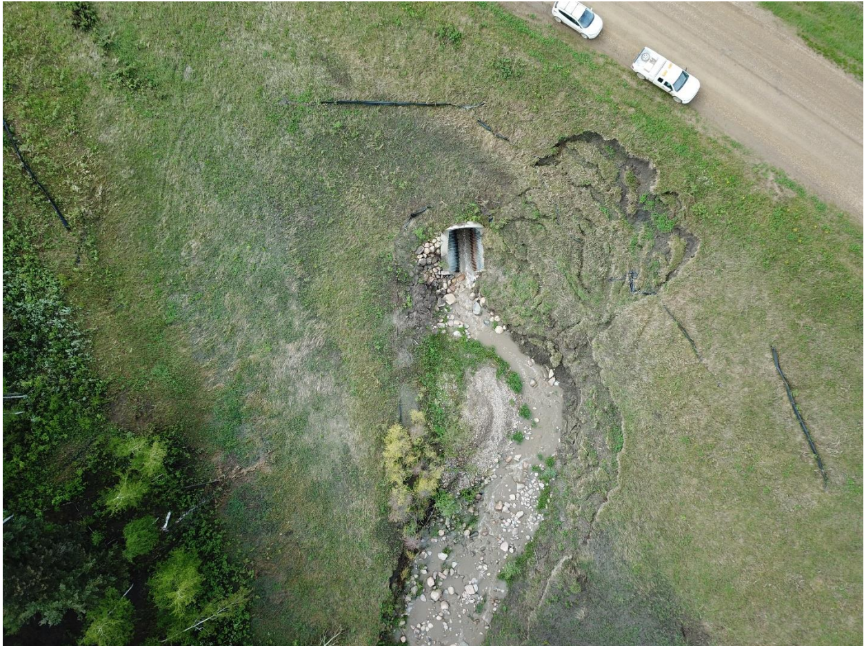
2020 UAV Image of slumping around culvert inlet.
