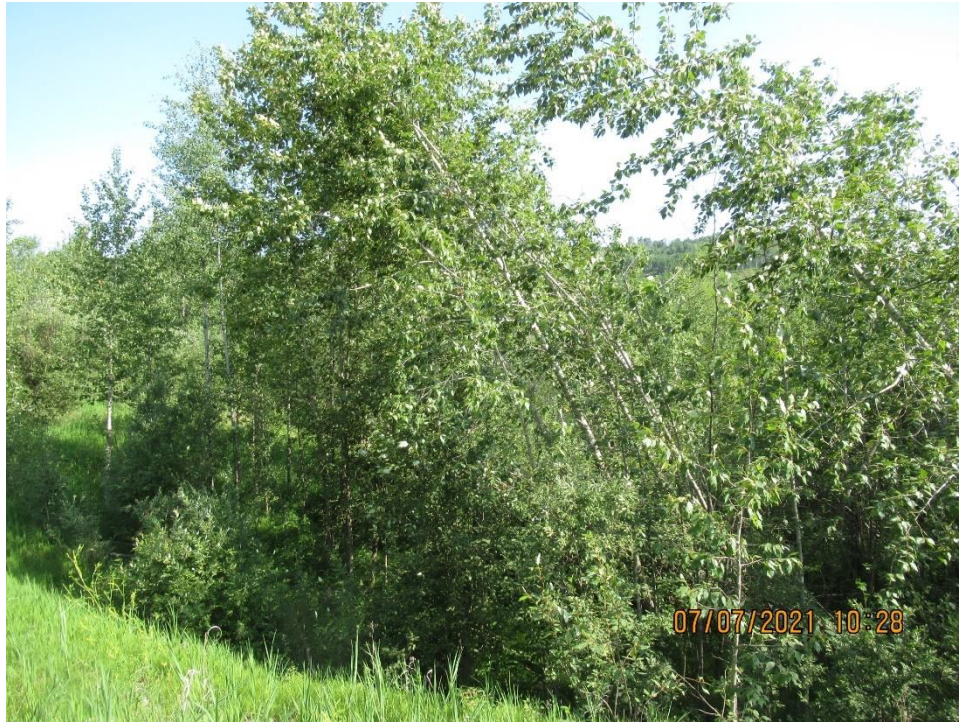
Site 2, Photo 5 – Rotating trees at the toe of the highway embankment.
