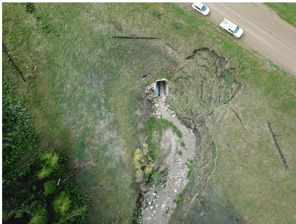
2020 UAV Image of slumping around Site 1 culvert inlet.
