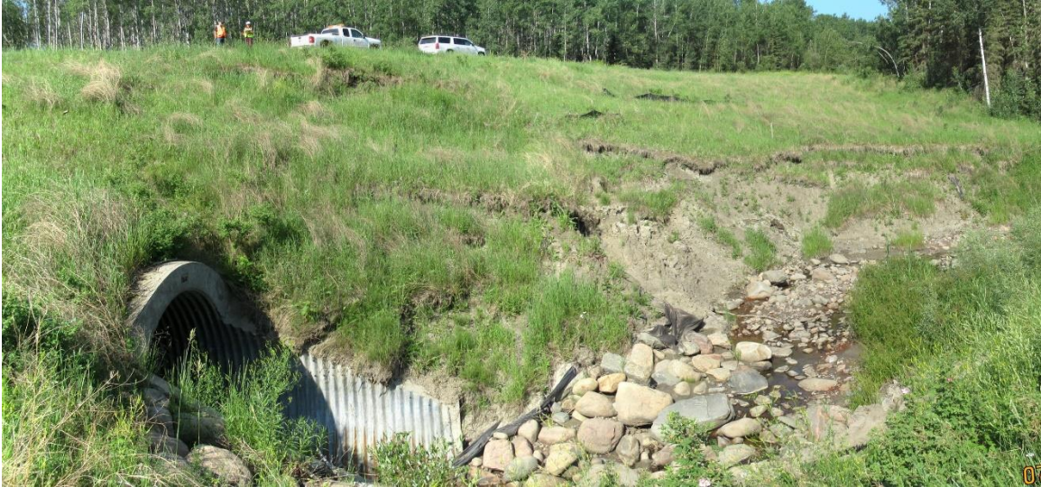
Site 1, Photo 1 – Looking west at north sideslope.
