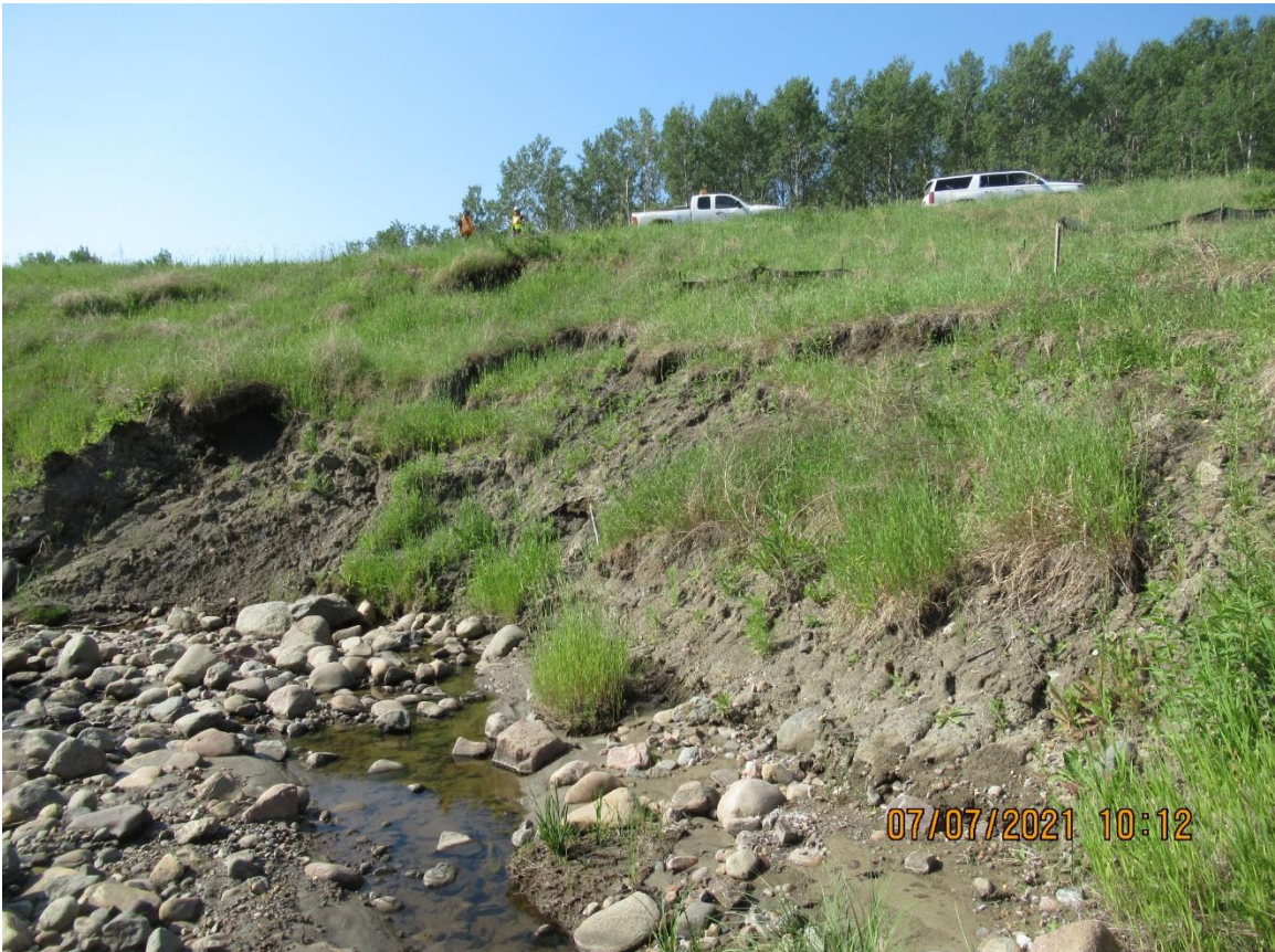
Site 1, Photo 2 – Looking southeast at creek bank slumping upstream of the culvert inlet.
