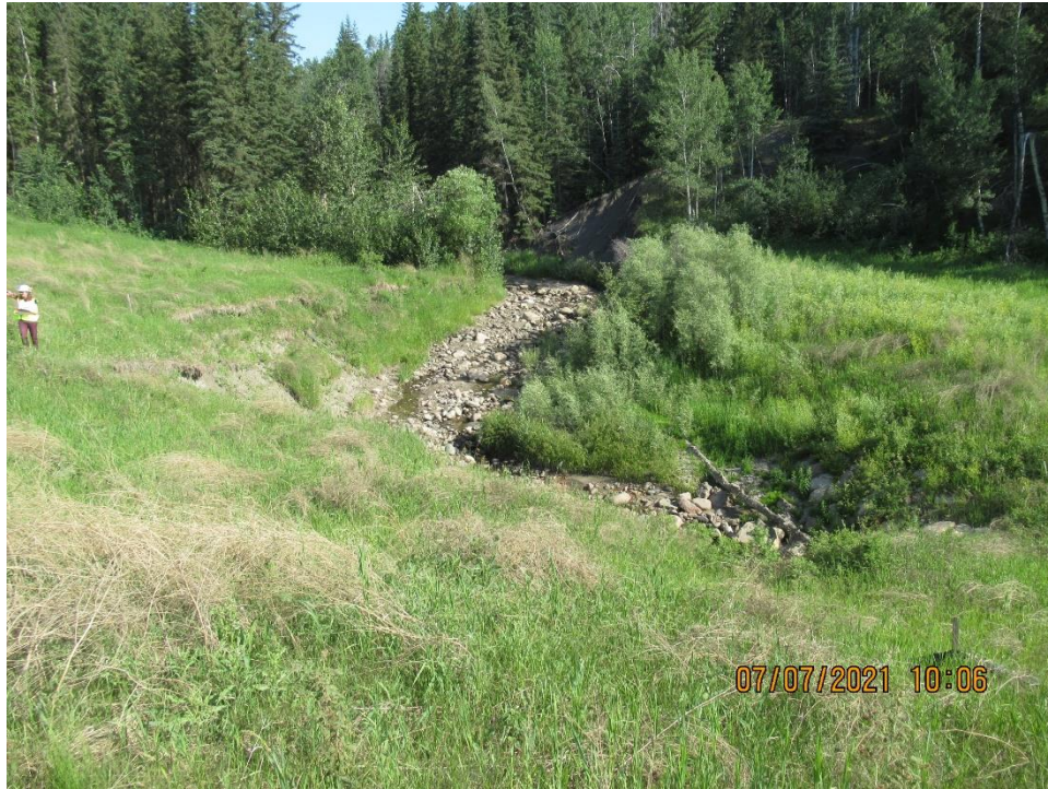
Site 1, Photo 3 – Looking north at creek bank slumping upstream of the culvert inlet. Note fresh material deposits on the right-hand side of the channel.
