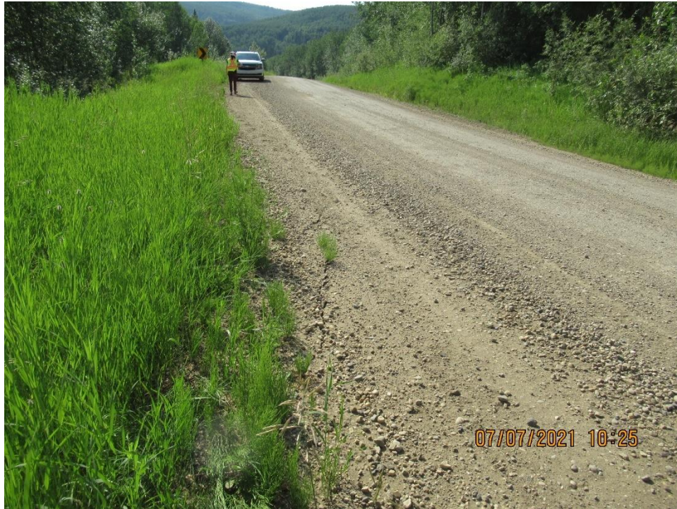
Site 2, Photo 3 – Looking at north end of cracks.
