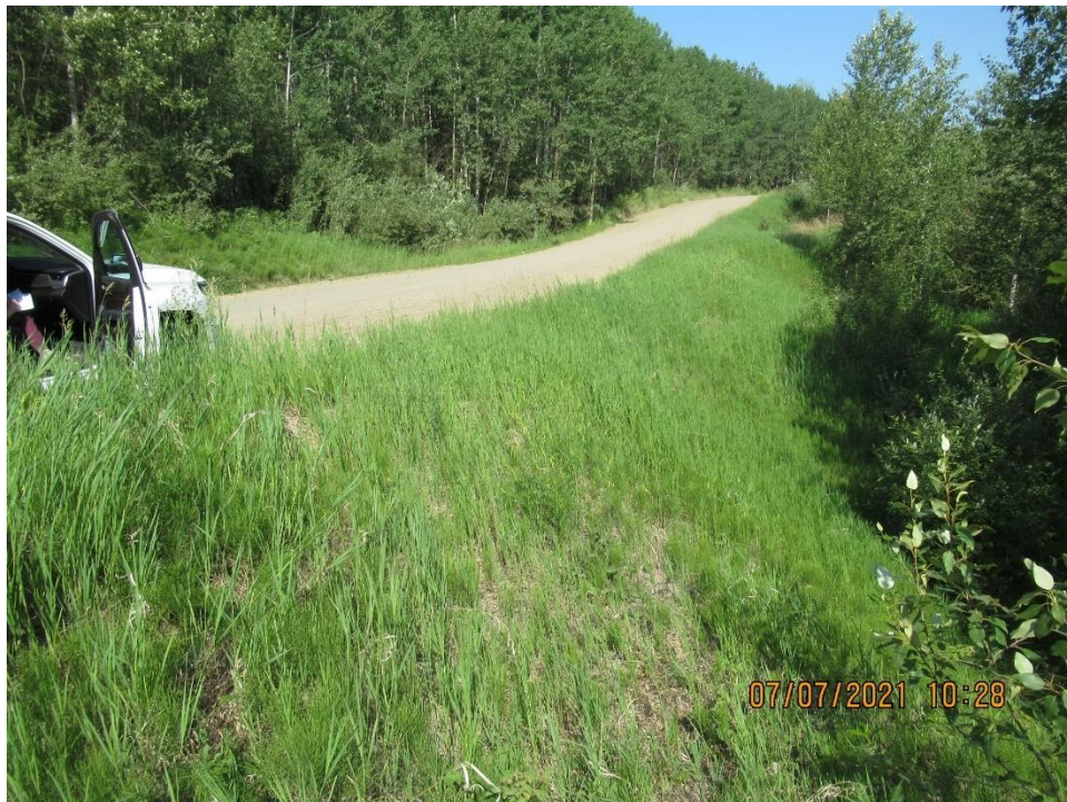
Site 2, Photo 4 – Looking at dip in highway surface over the slide.
