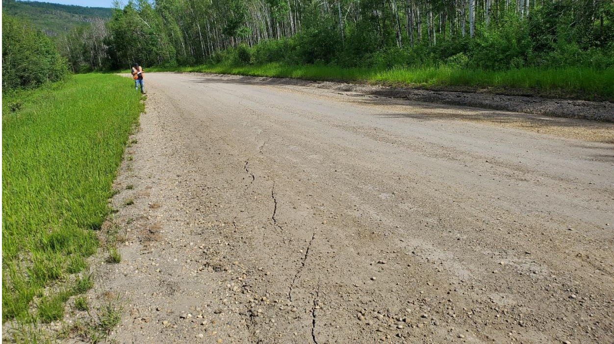
Photo 7 – Looking north at tension cracks on the west side of the roadway.
