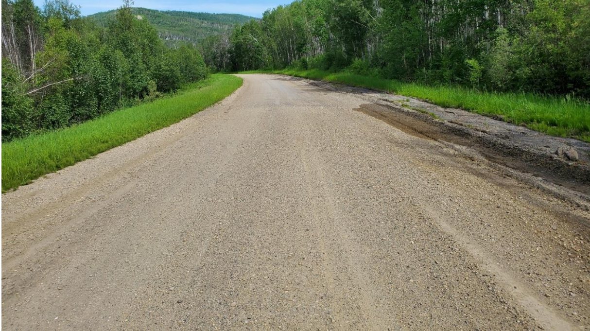
Photo 3 – Looking north at the slide located just beyond (north) of the seepage in the east ditch. There was no obvious vertical distortion of the roadway surface at the time of the callout inspection.
