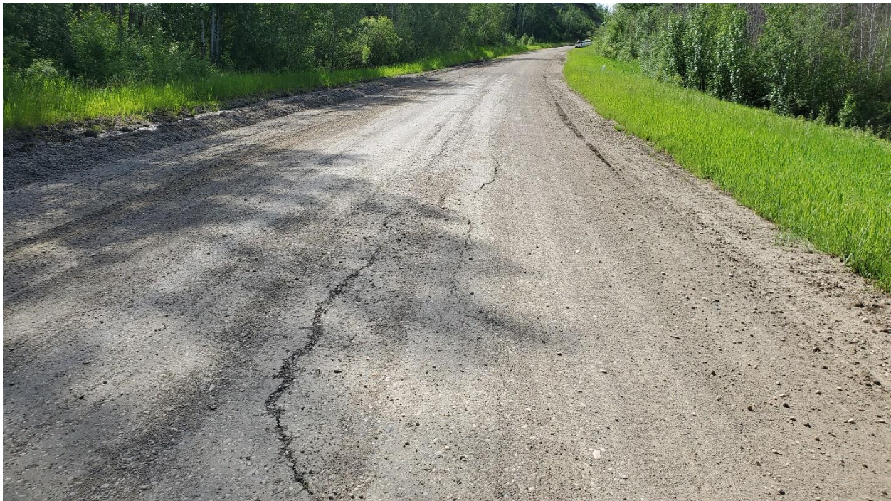
Photo 8 – Looking south at tension cracks on the west side of the roadway.
