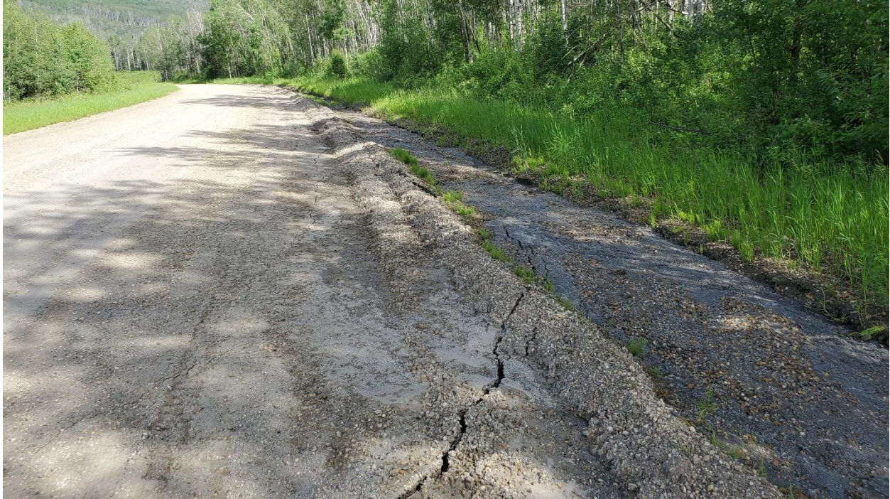
Photo 5 – Looking north at the main scarp crack cutting through the low graded berm. Note the wet material accumulated behind the berm from seepage further south.
