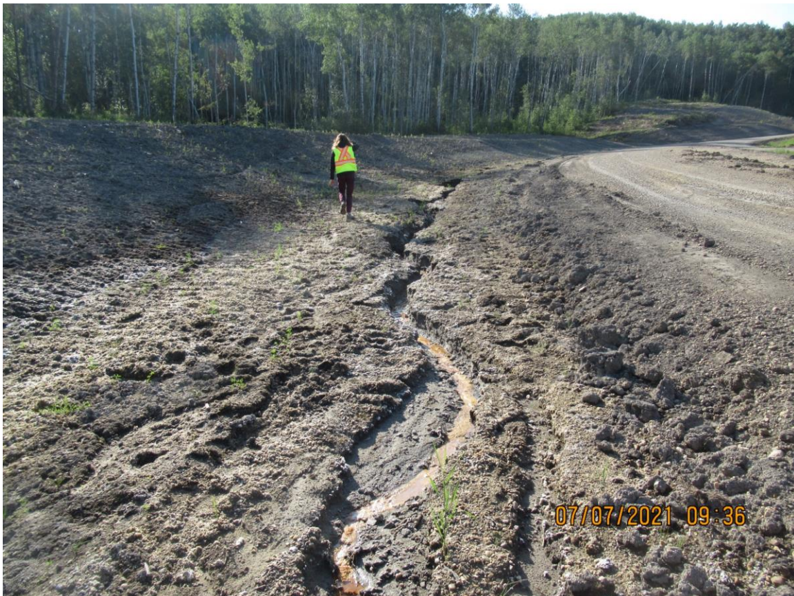
Photo 6 – Looking at erosion at north end of the ditch at the toe of the new backslope.
