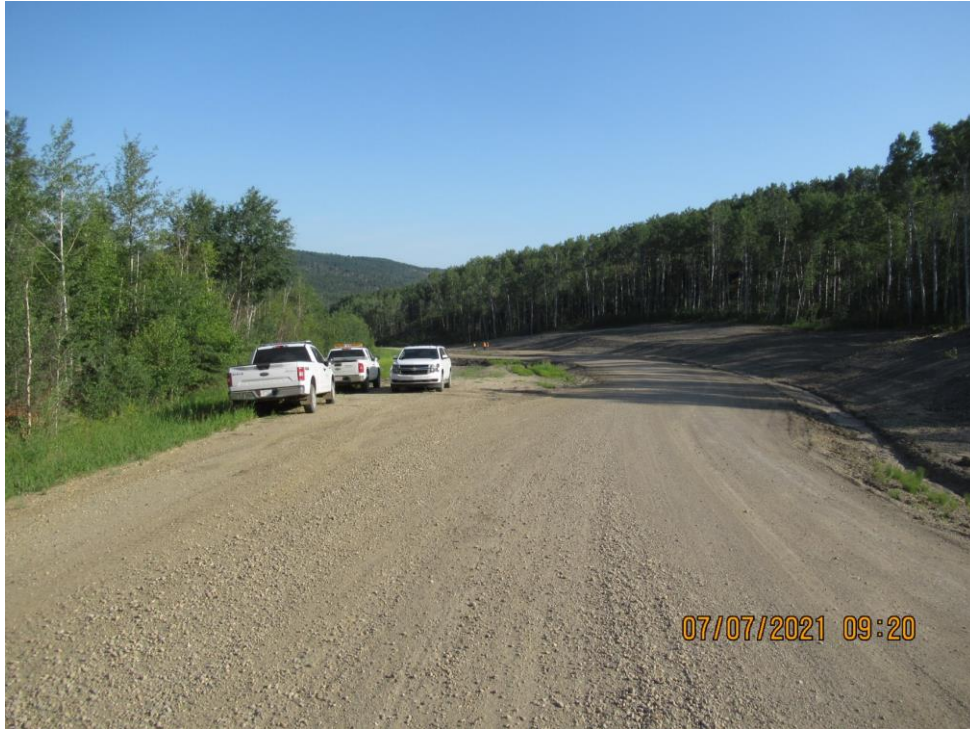
Photo 1 – Looking north at the landslide area. Trucks are parked along the old alignment with the temporary detour on the right. Note erosion in ditch at toe of backslope.
