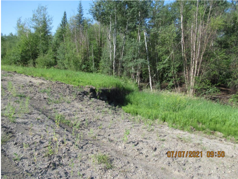
Photo 3 – Looking southwest at the south side of the landslide scarp.
