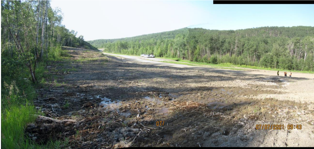
Photo 5 – Looking south at seepage accumulating at top of new backslope.
