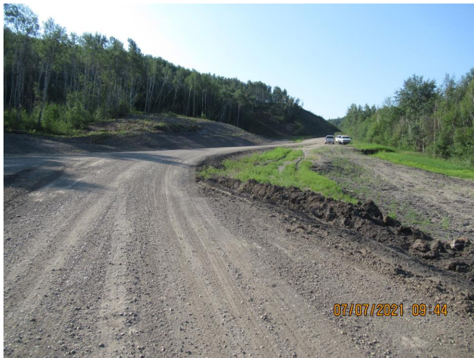
Photo 2 – Looking south along the alignment. Scarp through the old road visible in front of the trucks.
