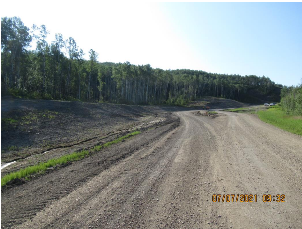
Photo 4 – Looking south at the north end of the detour where it splits around a soft area.
