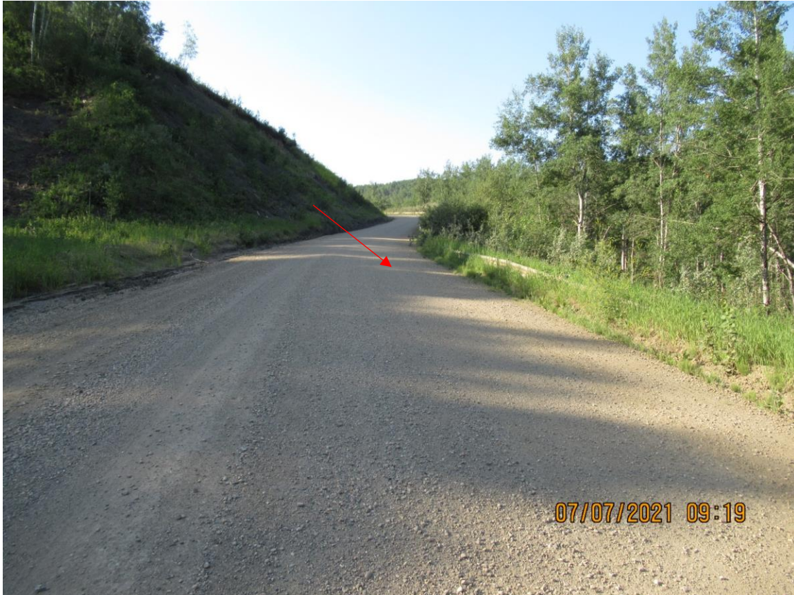
Photo 7 – Looking south towards the south landslide lobe and high shale backslope (PH011-2) on left. The cracks are at the guardrail but had been graded out at the time of the photo.
