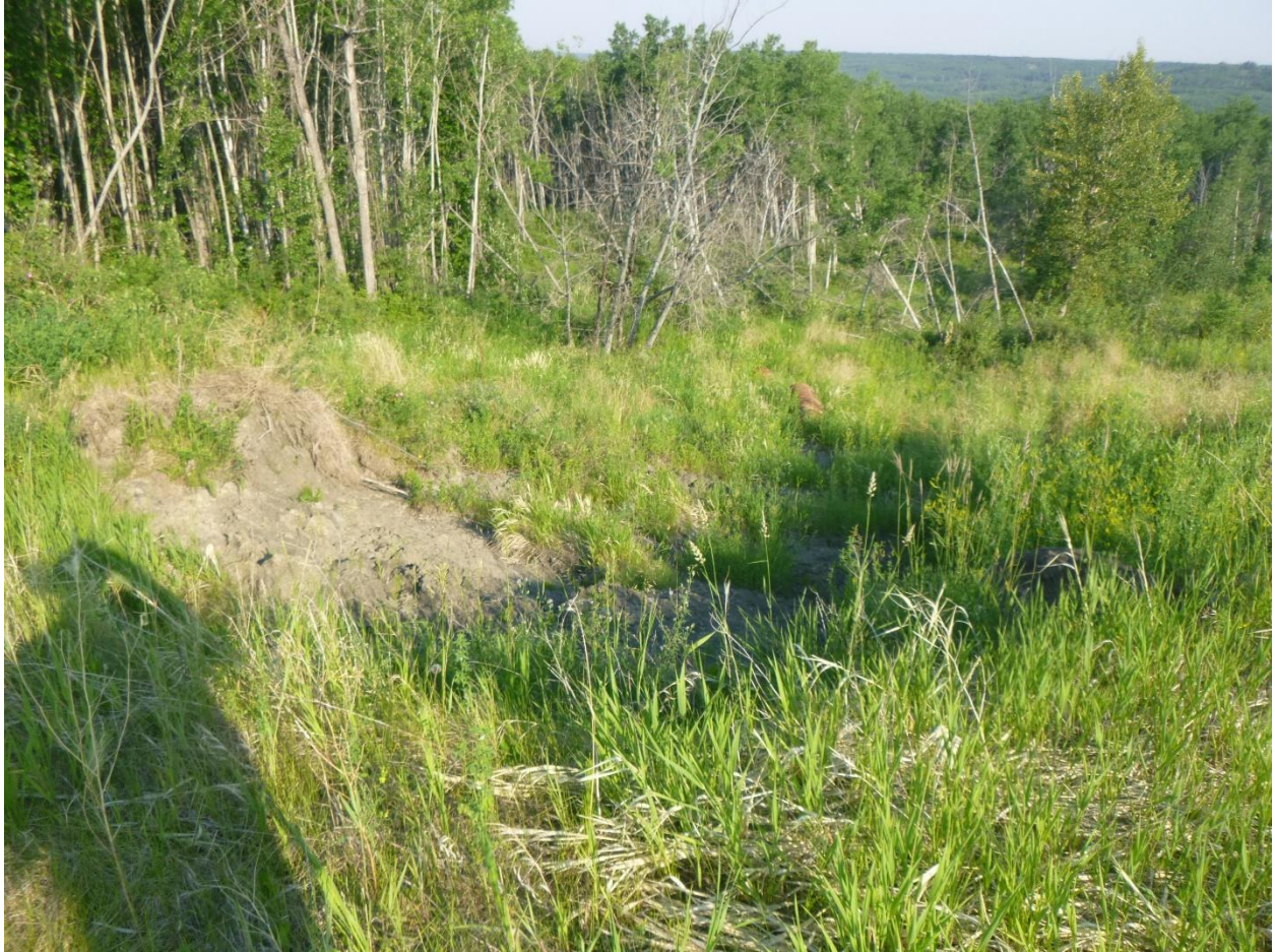
Photo 4 – Looking west at slide at km 14.45 located adjacent to south gabion basket swale.
