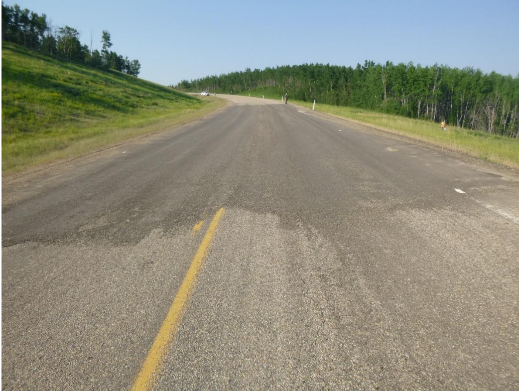
Photo 3 – Looking south at patched pavement area.
