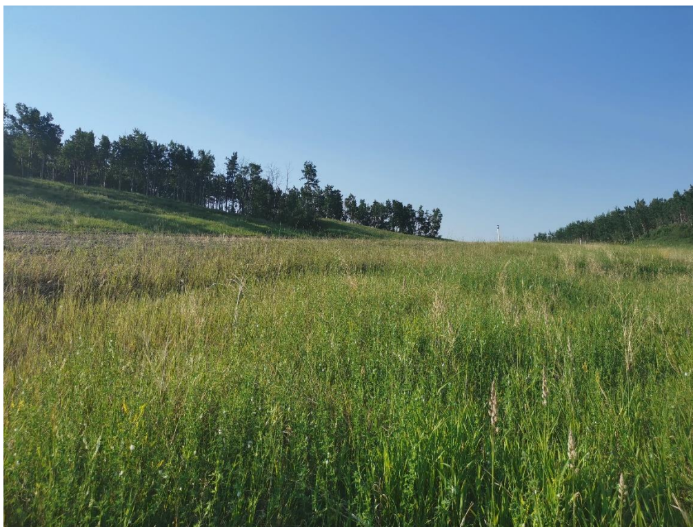
Photo 5 – Looking southeast at scarps forming close to the highway at about km 14.48
