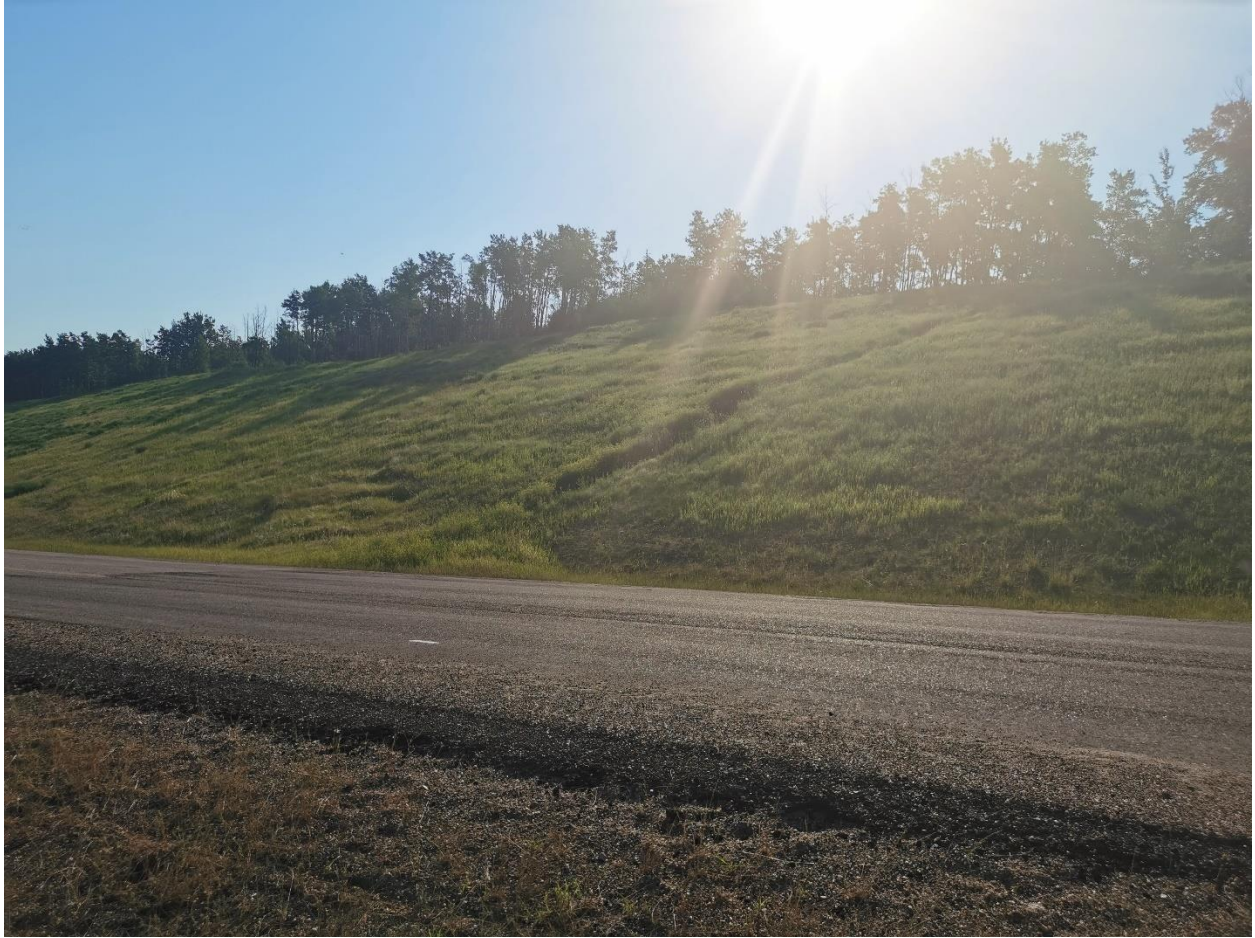
Photo 1 – North gully; note slump to left of gully on lower part of slope.
