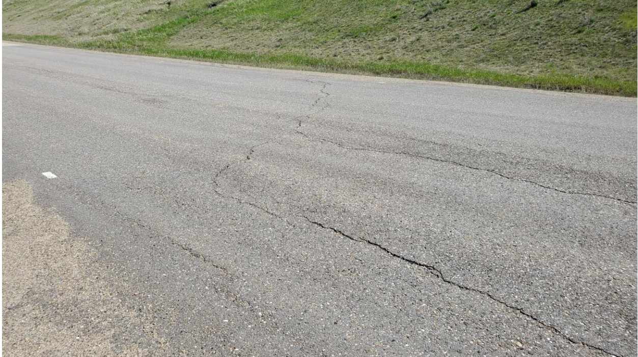
Photo 3 – Looking northeast at crack pattern reflecting through recent patch on highway above scarps shown in Photo 7.
