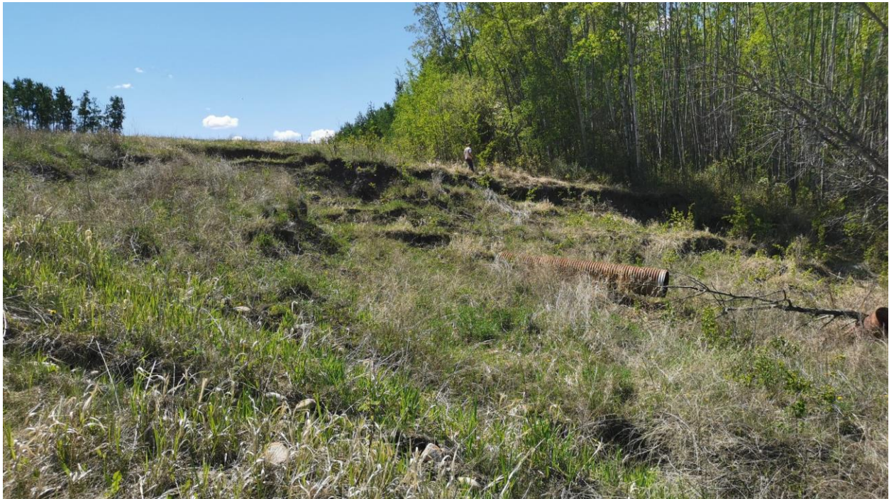
Photo 4 – Looking south at fresh slide at km 14.45 located adjacent to south gabion basket swale. The culvert may be from the previous highway alignment.
