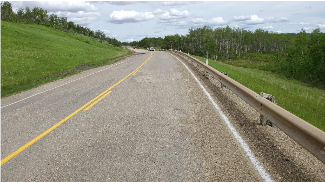
Photo 6, Site 4 – Looking east at transverse crack and patch at ~km 18.820.
