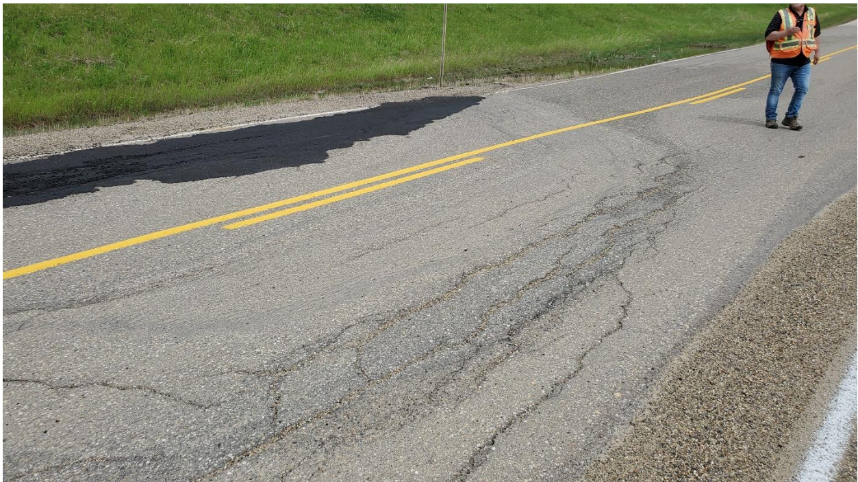
Photo 8 – Looking northeast of a portion of the patch at km 18.84.
