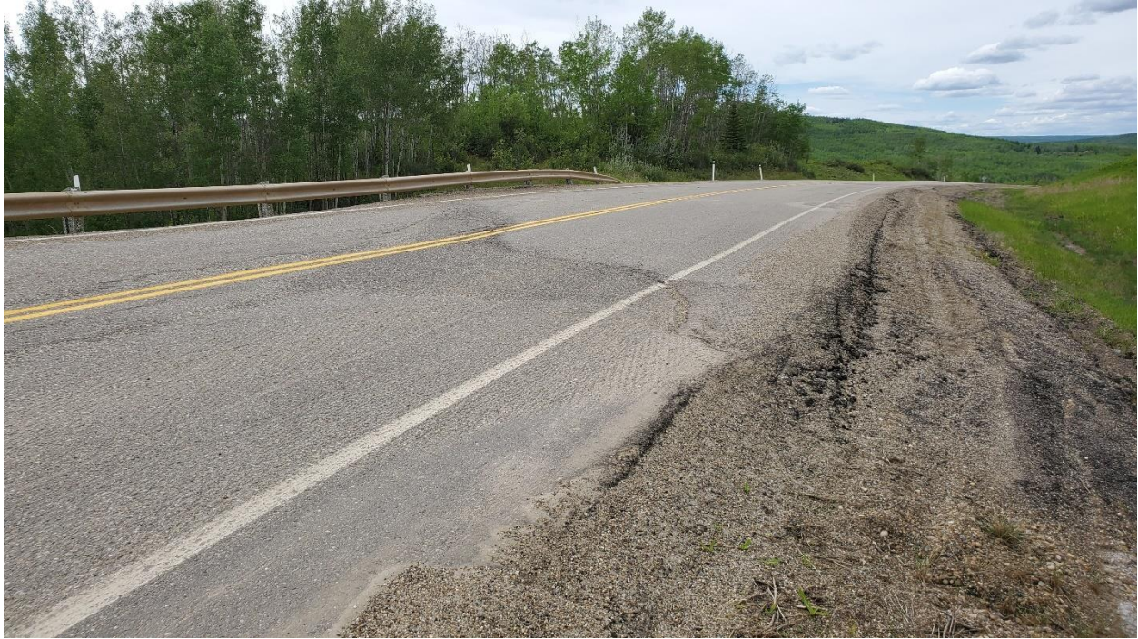
Photo 7, Site 4 – Looking southwest at dip in highway surface at ~km 18.840.
