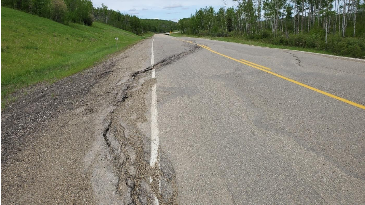
Photo 3, Site 9: Looking northeast at braided crack in highway surface over main slide scarp.
