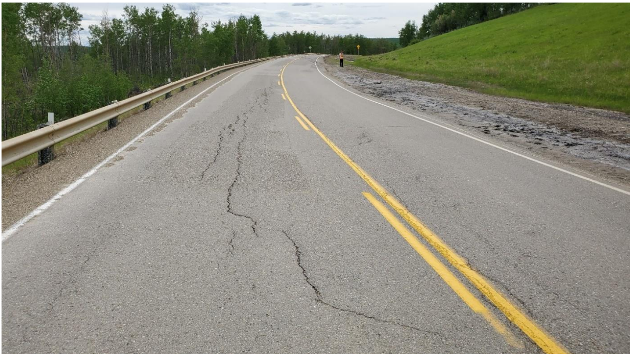
Photo 2, Site 8 – Looking southwest from the northeast end of Site SH012-8. Note main scarp crack has reflected through the new patch.
