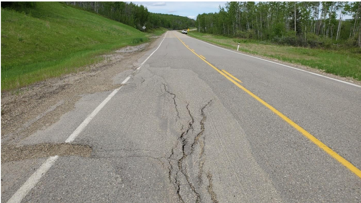
Photo 6, Site 9: Looking northeast near northeast end of site where main slide scarp moves north of highway.
