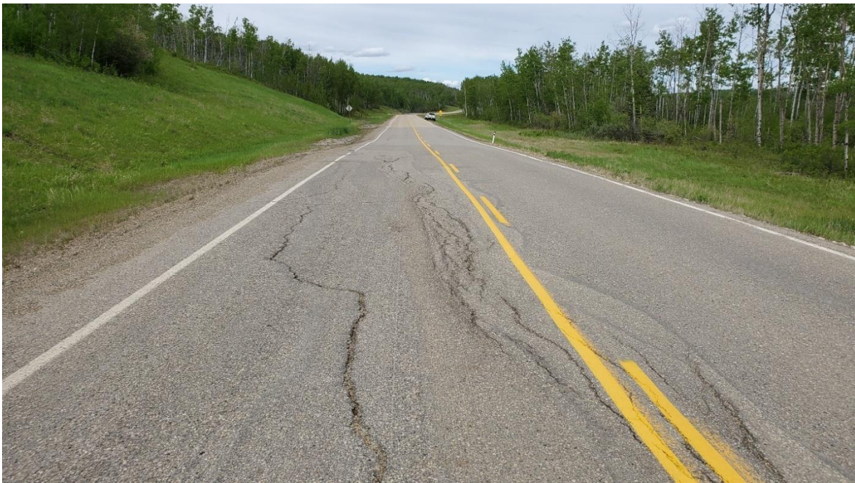
Photo 4, Site 9: Looking northeast at cracking and milling near northeast end of site.
