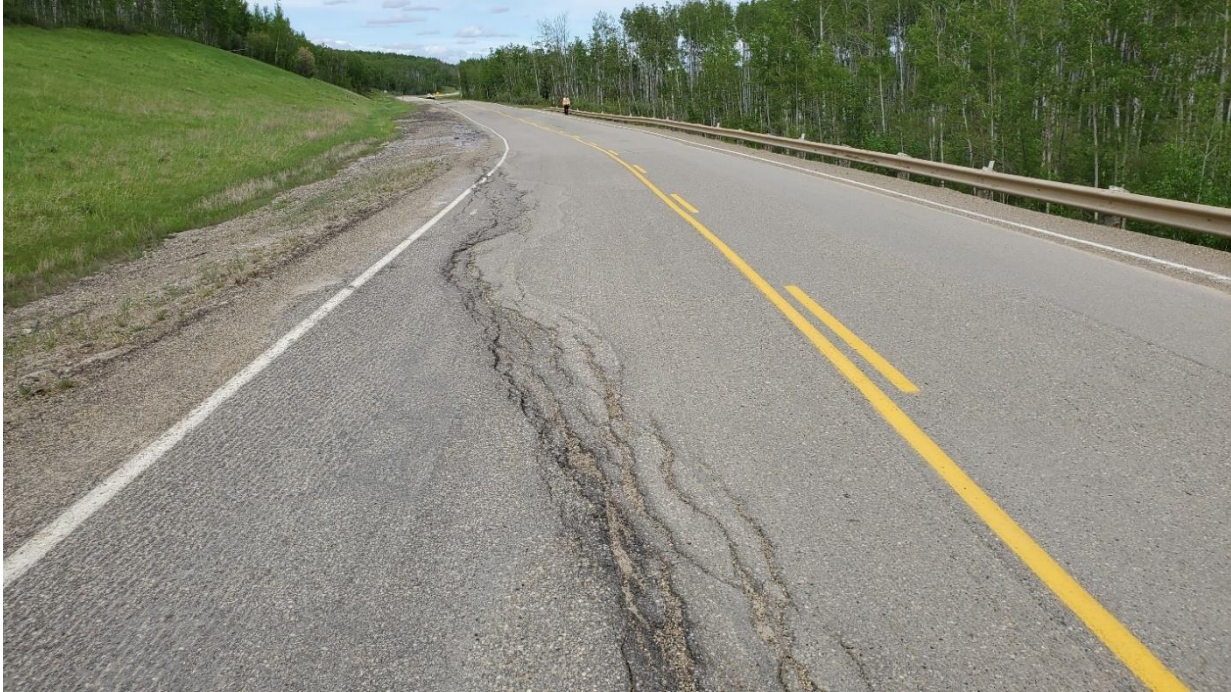
Photo 1, Site 8 – Looking northeast from the southwest end of the Site along a major scarp crack.
