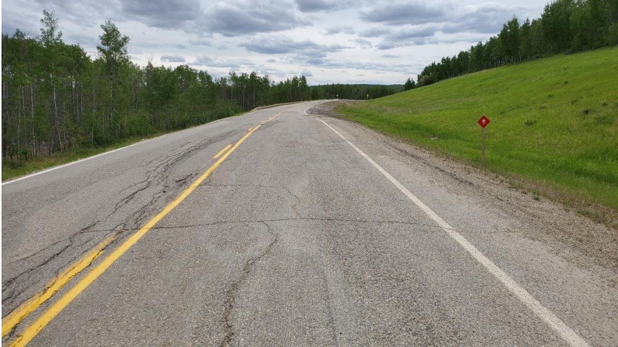
Photo 5, Site 9: Looking southwest at braided crack along main slide scarp. Note milling material used to regrade sideslope and ditch.
