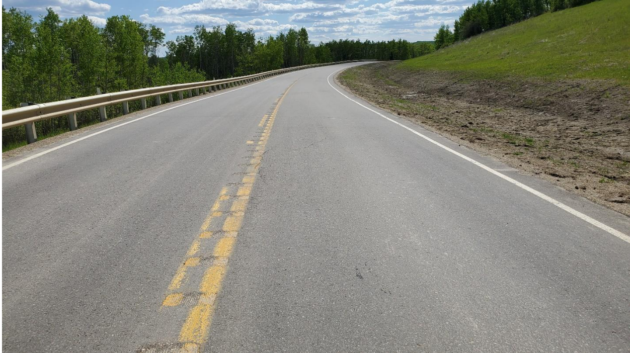
Photo 1, Site 8 – Looking southwest from the northeast end of Site SH012-8. Previous main scarp crack not clearly visible during inspection.
