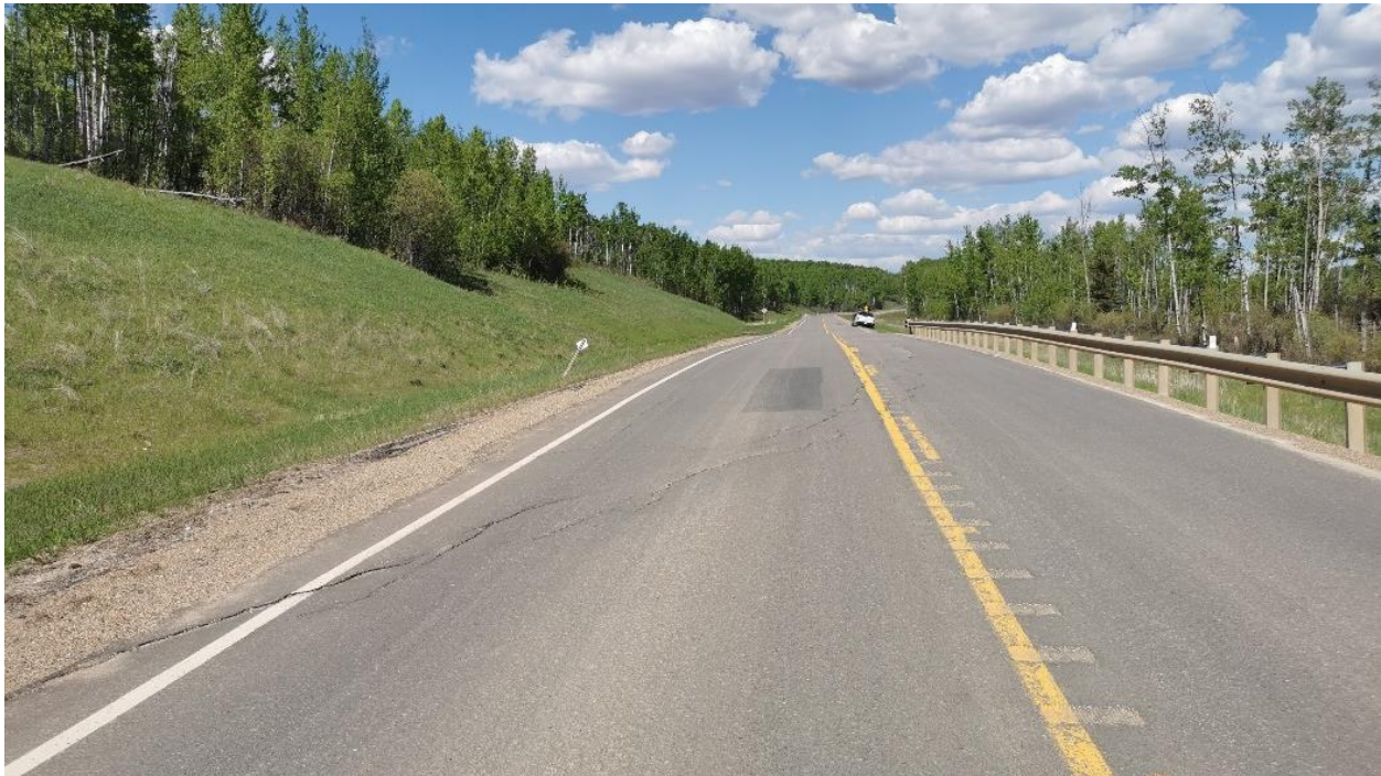
Photo 2, Site 9: Looking northeast at crack in highway surface over main slide scarp that is reflecting through the recent highway overlay.
