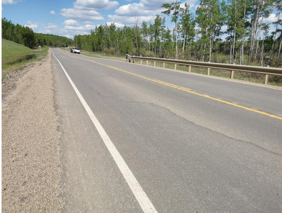
Photo 3, Site 9: Looking northeast at cracking near northeast end of site.
