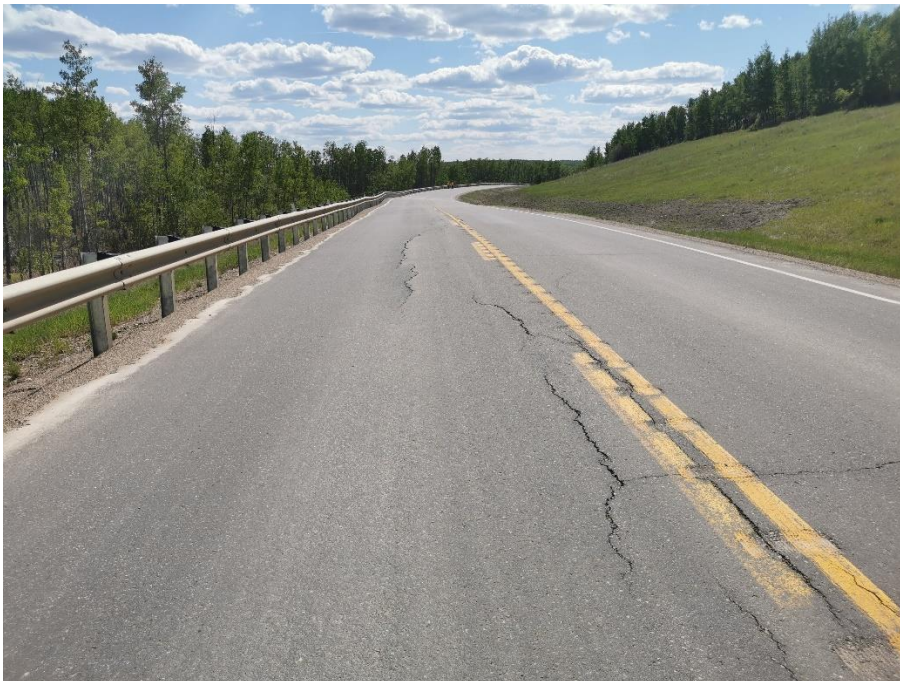
Photo 4, Site 9: Looking southwest at crack along main slide scarp.
