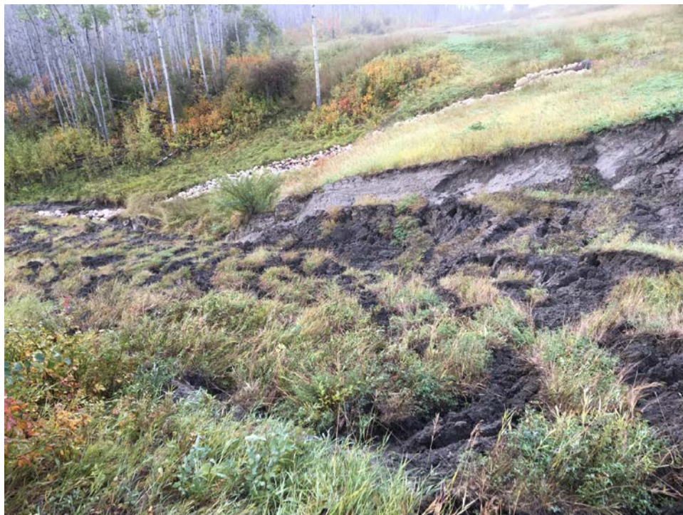
Photo 2: Looking south at upper portion of the slide.
