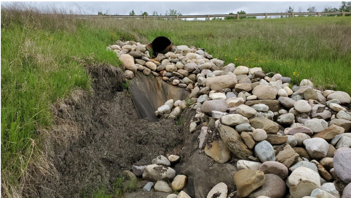
Photo 4: Looking northwest at new culvert outlet. Erosion on left-hand side (south) is significantly worse and may be part of a retrogressive tension crack from the slide further down the slope.
