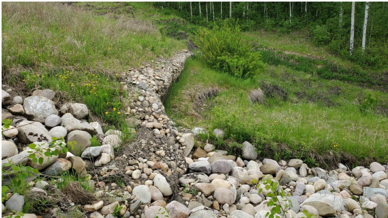
Photo 6 – Scarps above and below the gabion wall at the riprap apron.
