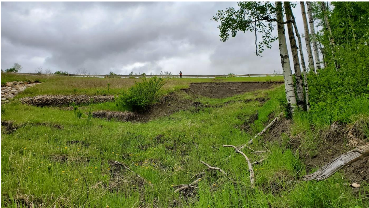
Photo 8 – Looking west at slide in the north half of the embankment with tension cracks extending into the south half at and below the gabion wall.
