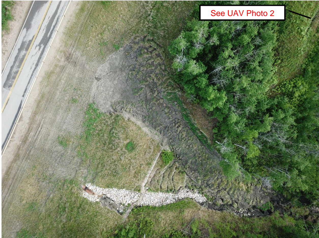
UAV Photo 1: Landslide on east side of highway embankment
