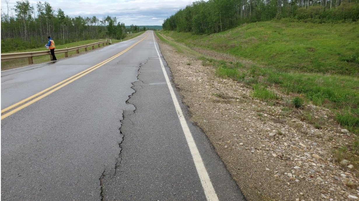
Photo 1 – Looking south at reconstructed upslope shoulder - note tension crack forming in roadway with differential settlement.
