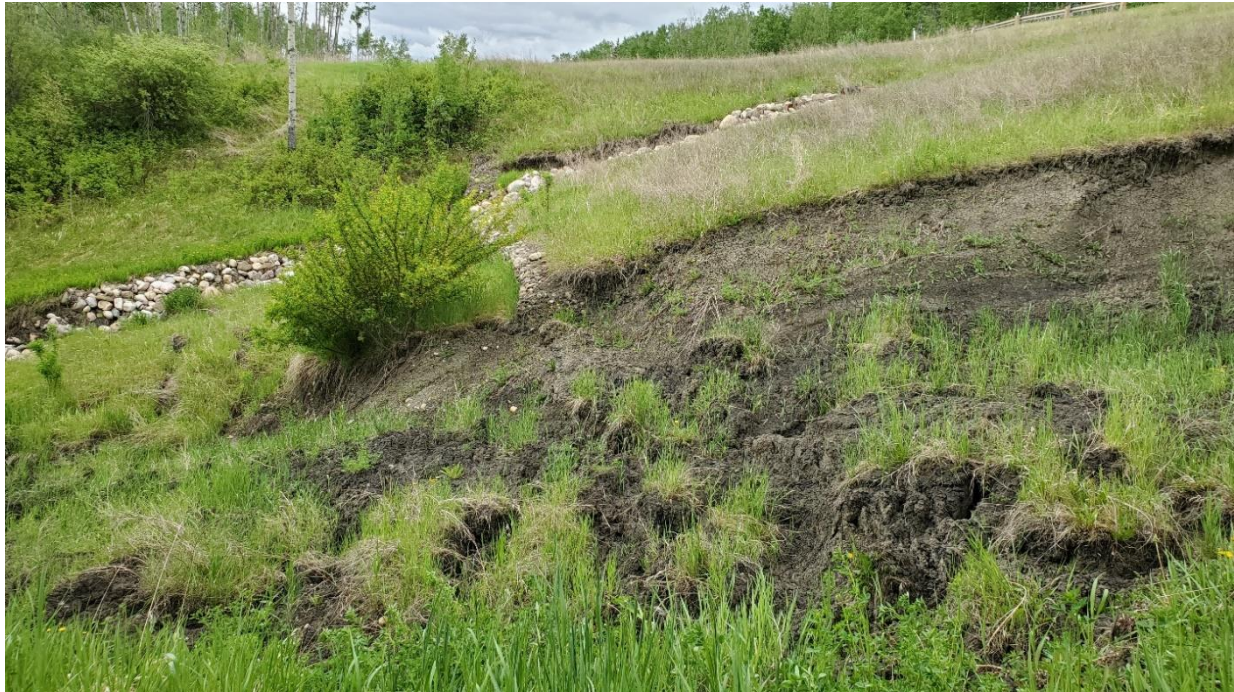
Photo 5 – Looking south at gabion wall on downslope side of embankment. Note eroded south face of new riprap apron from culvert outlet. September 2018 slide has removed about half of the gabion wall.
