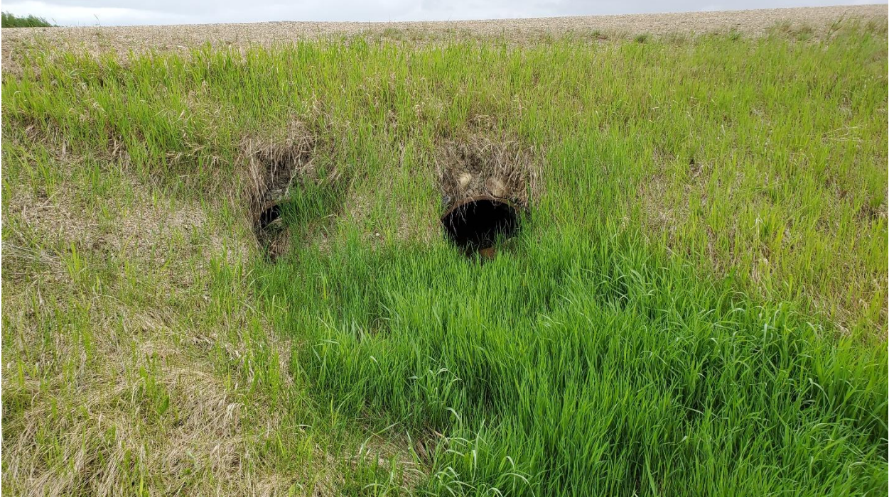
Photo 3, Site 14 – Looking at twin culverts outlets which convey west ditch flow to the east.
