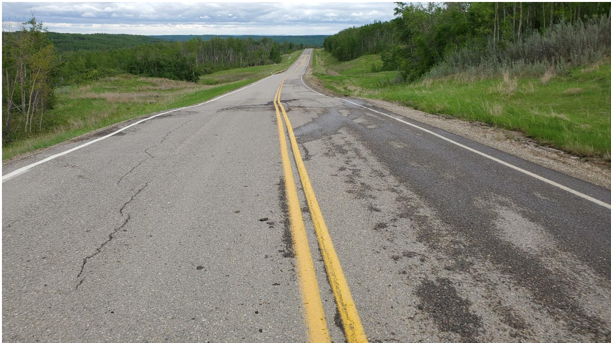
Photo 6, Site 15 – Looking south at the main crack.
