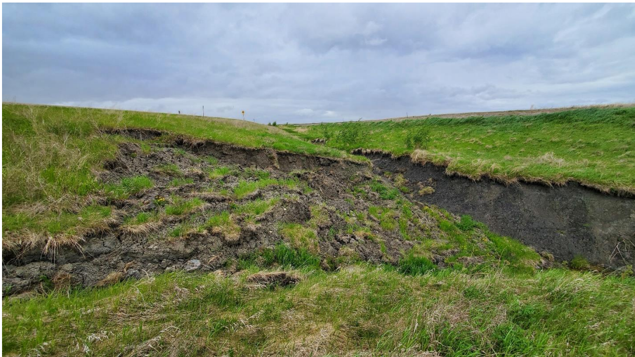
Photo 2, Site 14 – Looking north along the ditch where the erosion gully begins.
