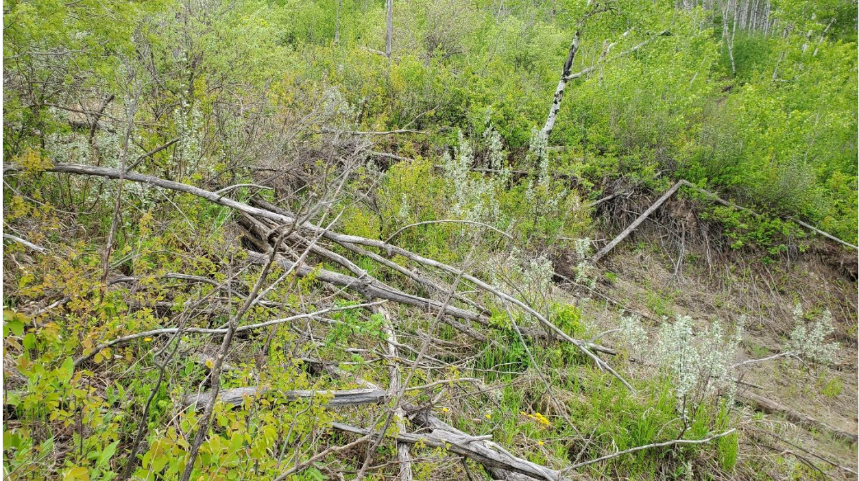
Photo 7, Site 15 – Looking north at head of shallow slump downslope of the highway.
