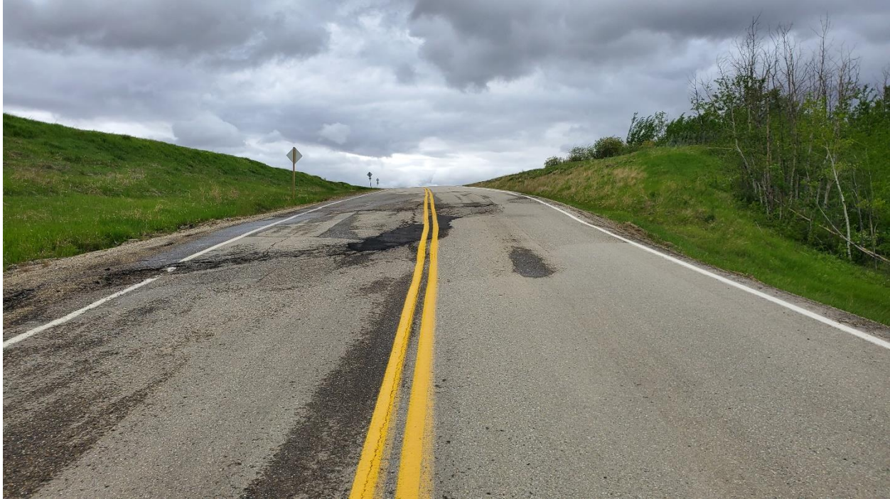
Photo 5, Site 15 – Looking north at diagonal crack intersecting the highway. There is a slight dip in the east lane on the south side (downslope) of the crack.
