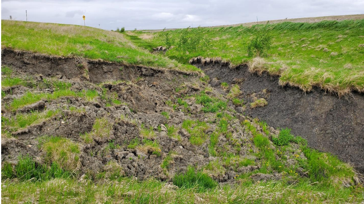
Photo 1, Site 14 – Looking north through east at increasing depth of erosion along the tributary.
