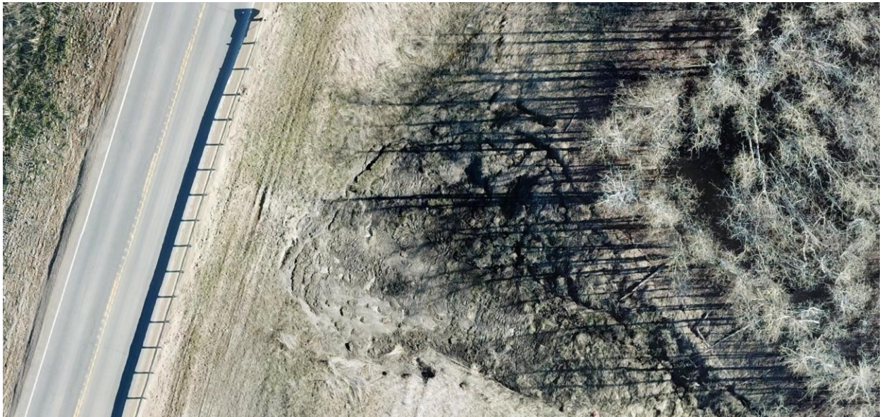
UAV Photo 2 (May 2022): Closer view of the east slump encroaching towards the highway (5.1 m from back of W-Beam guardrail).
