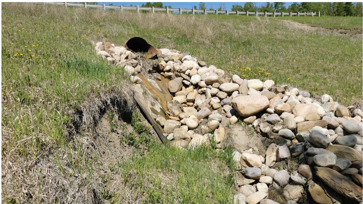
Photo 4: Looking northwest at new culvert outlet. Erosion on left-hand side (south) is significantly worse and may be part of a retrogressive tension crack from the slide further down the slope.
