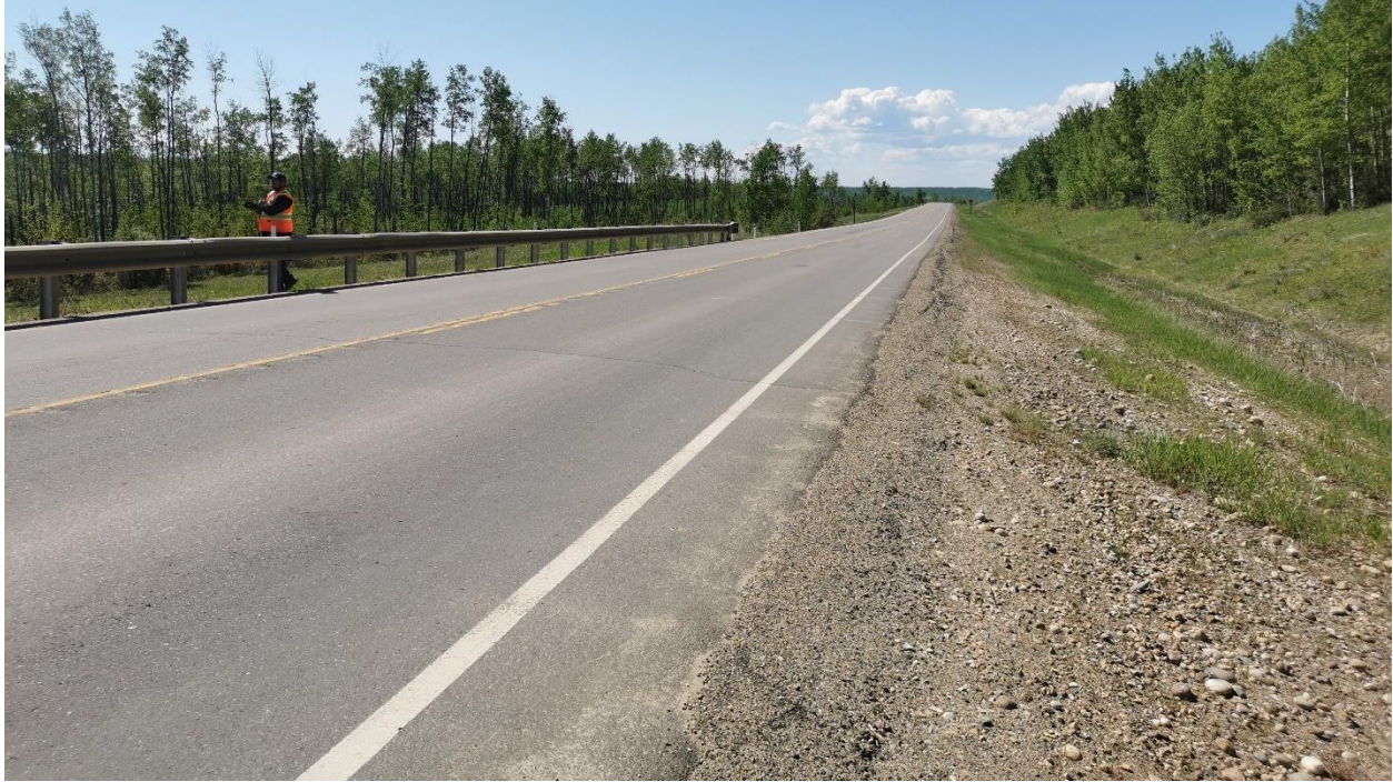
Photo 1 – Looking south at upslope shoulder – the highway was overlaid the previous year and the crack pattern is not yet fully re-established.
