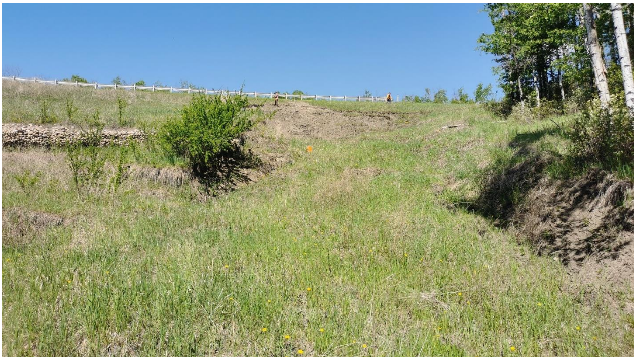
Photo 8 – Looking northwest at slide in the north half of the embankment with tension cracks extending into the south half at and below the gabion wall.
