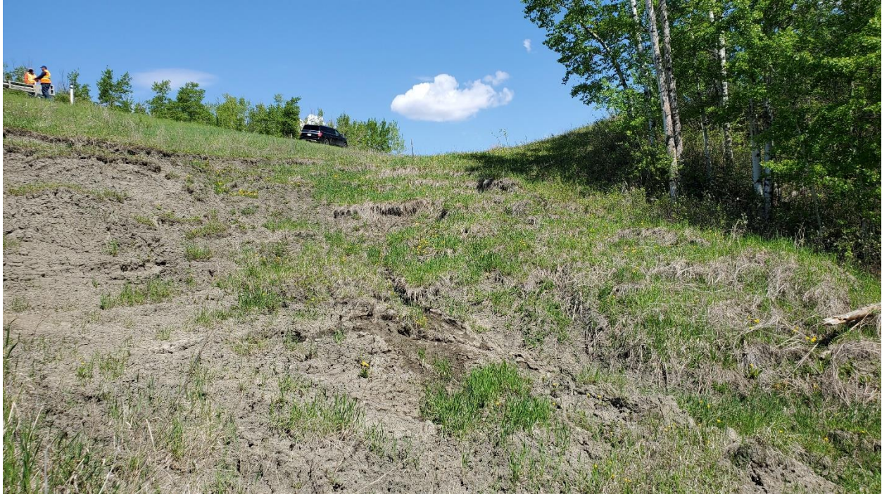
Photo 7 – Looking northwest at top of September 2019 slide block.
