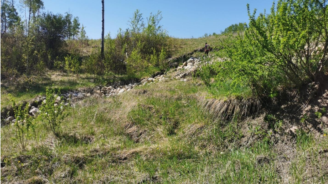
Photo 5 – Looking south at gabion wall on downslope side of embankment. Note eroded south face of new riprap apron from culvert outlet. September 2018 slide has removed about half of the gabion wall.
