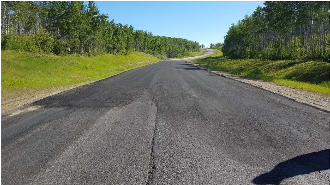
Photo 2 – Looking northeast from southwest end of recent patch and Site. Note longitudinal cracking.
