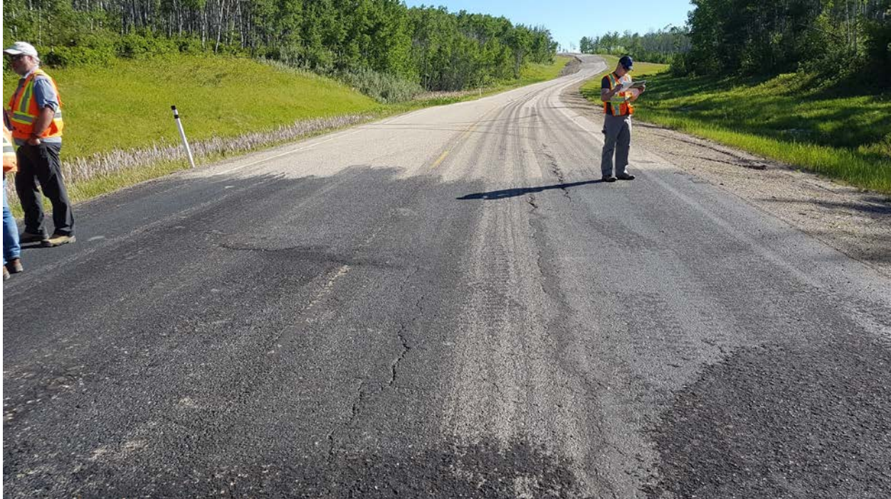
Photo 3 – Looking northeast at longitudinal cracking near northeast end of recent patch and Site.
