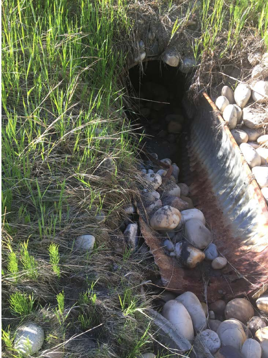
Photo 5 – Looking at culvert inlet distress: partial obstruction with cobbles from ditch lining and sinkhole (not visible in photo) forming near edge of the highway shoulder.
