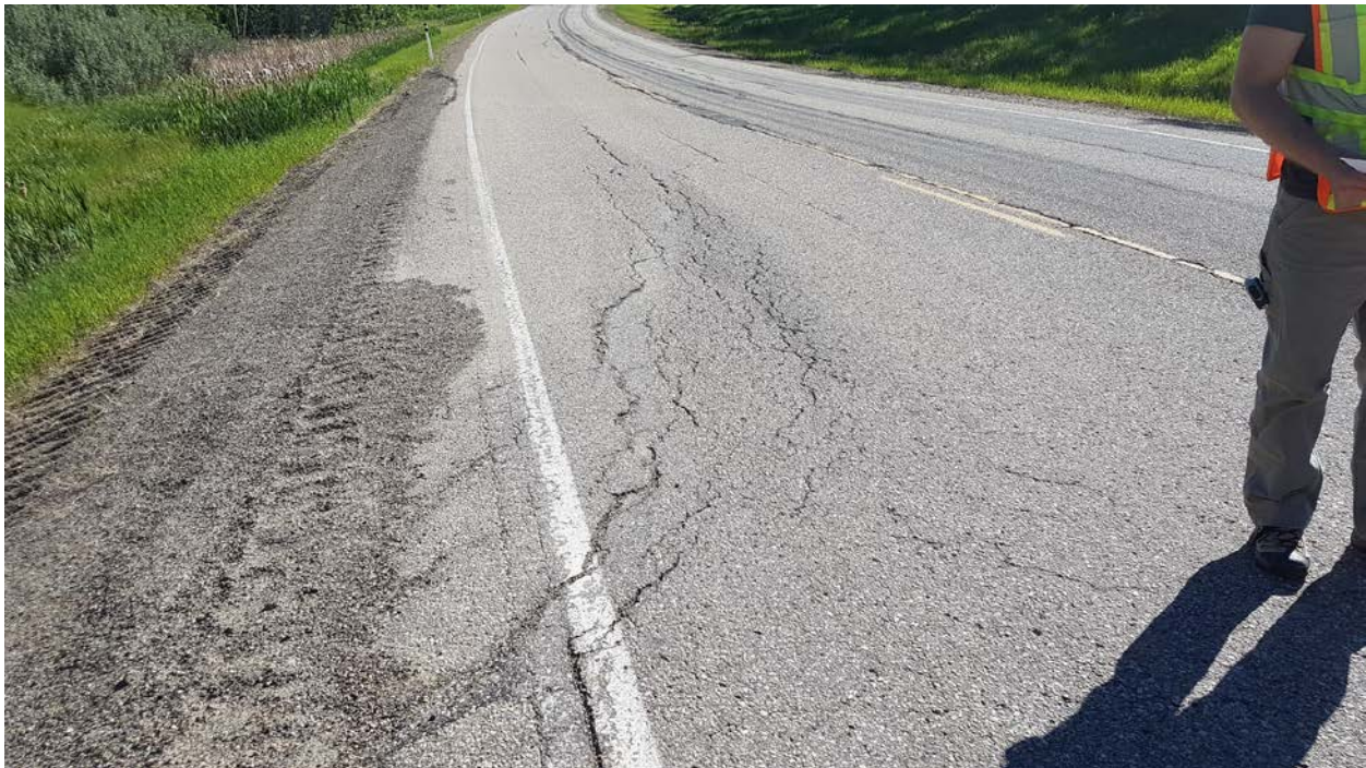
Photo 4 – Looking northeast at scarp crack northeast of patched section.
