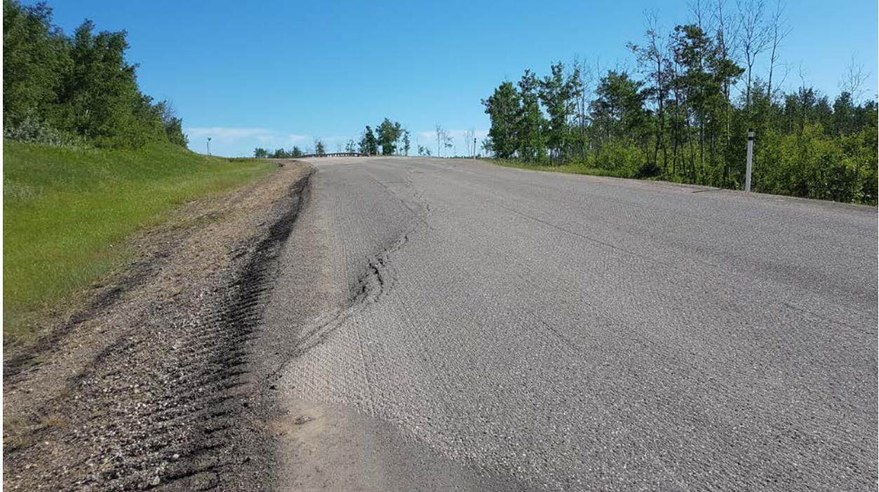
Photo 5 – Looking northeast at north scarp crack.
