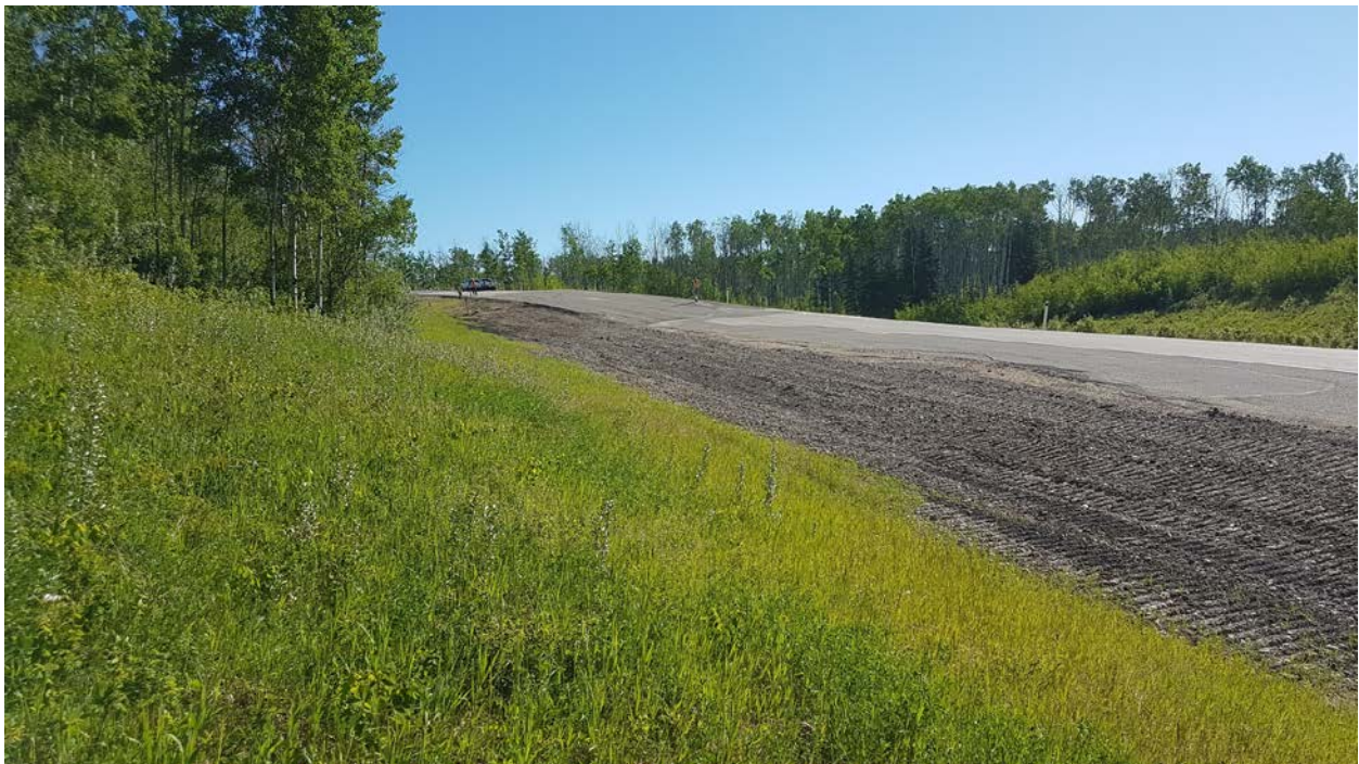
Photo 2 – Looking east at vertical distortion of highway at south end of site and regraded sideslope where there had been a significant gully.
