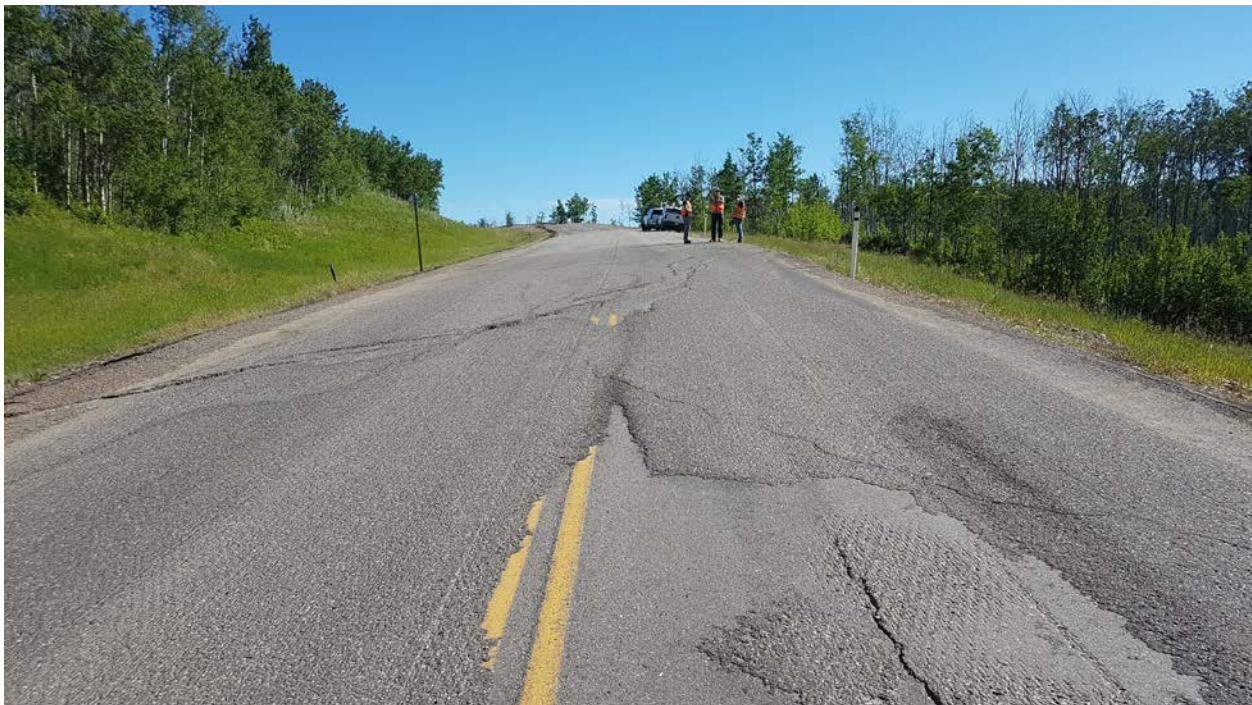
Photo 4: Looking northeast where main scarp crack crosses the highway at the central portion of Site 11.
