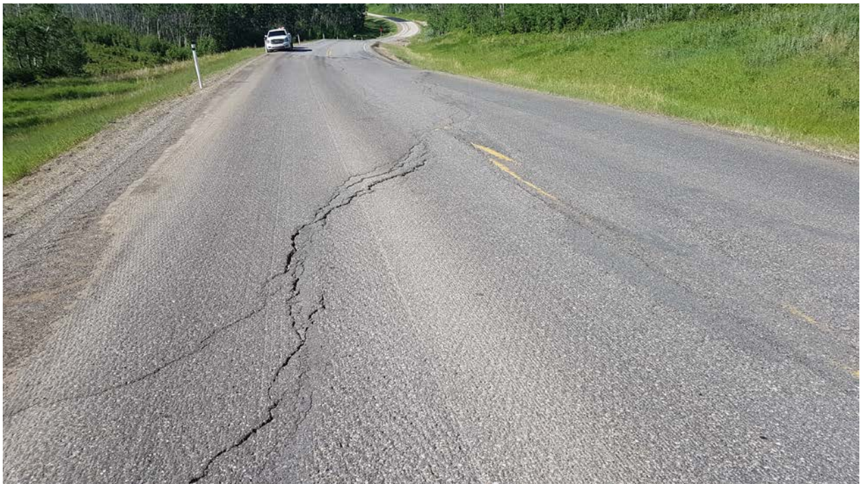
Photo 6 – Looking southwest at north scarp crack.
