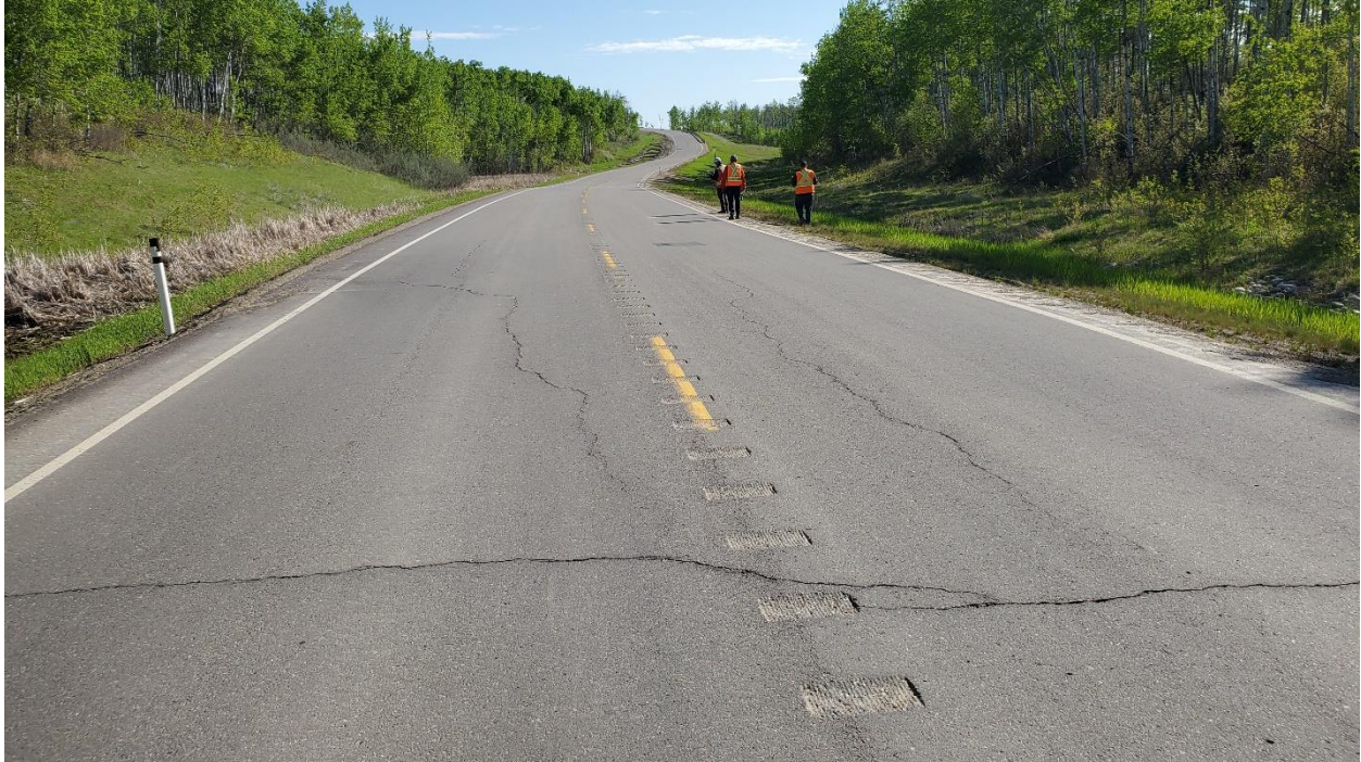
Photo 3 – Looking northeast at cracking that is starting to surface around km 20.26 (just northeast of the culvert).
