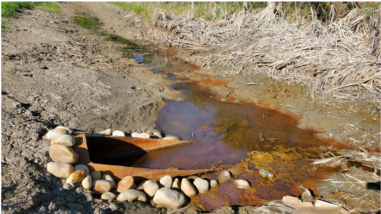
Photo 8: Poor drainage and ponding water at the km 20.38 culvert inlet.
