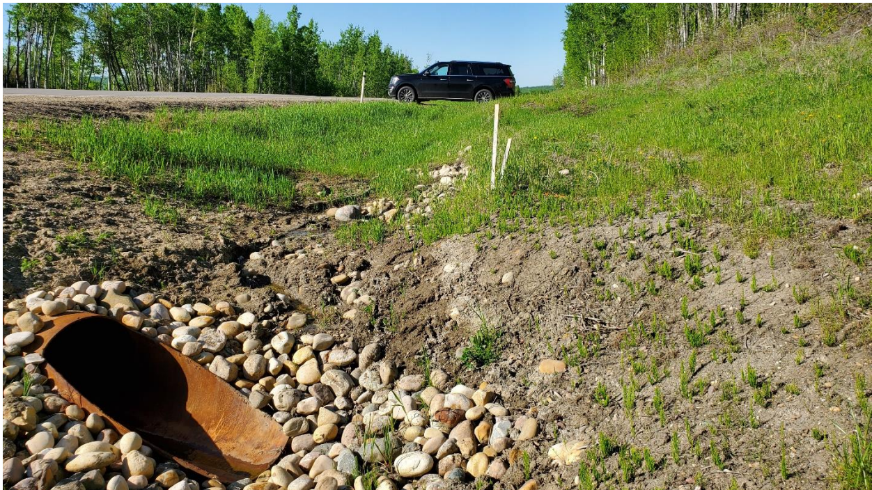
Photo 6: Erosion adjacent to km 20.22 culvert inlet (right side of Photo 5).
