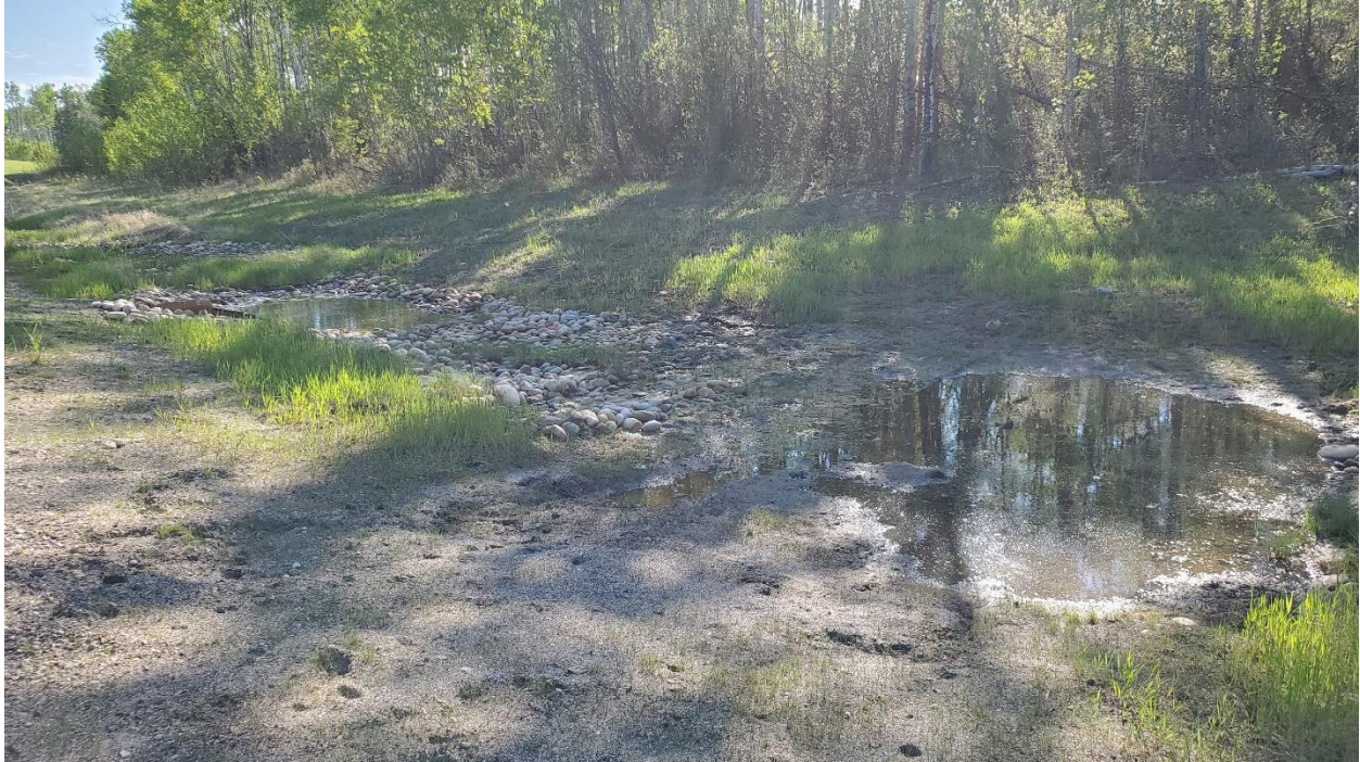
Photo 7: Ponding water in reggraded downslope ditch at the km 20.38 culvert outlet.
