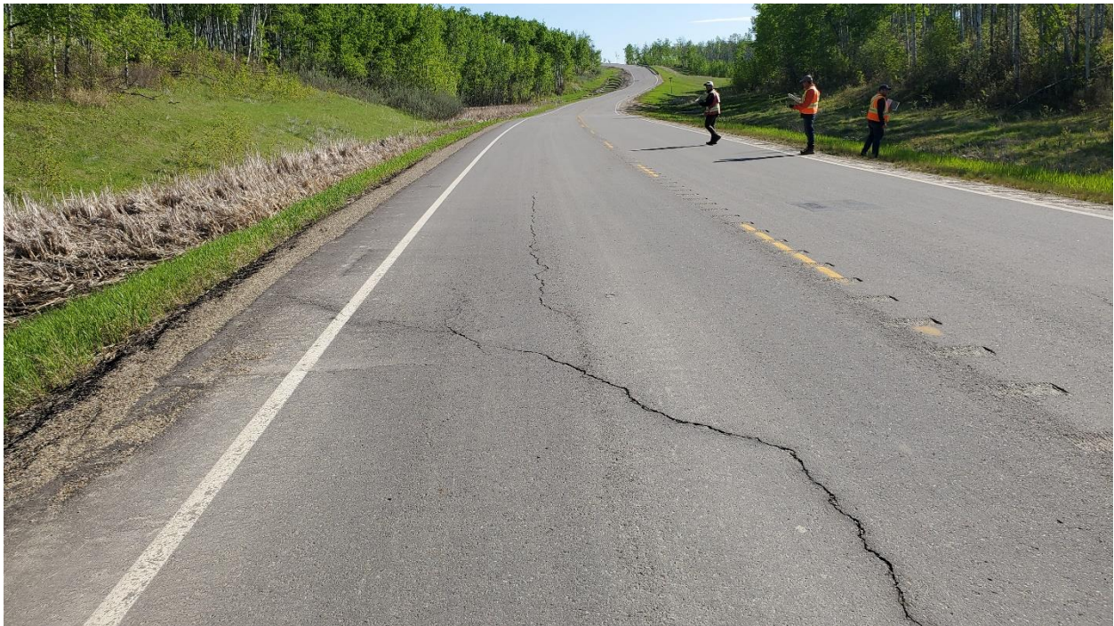
Photo 4 – Looking northeast at potential scarp crack northeast of Photo 3.
