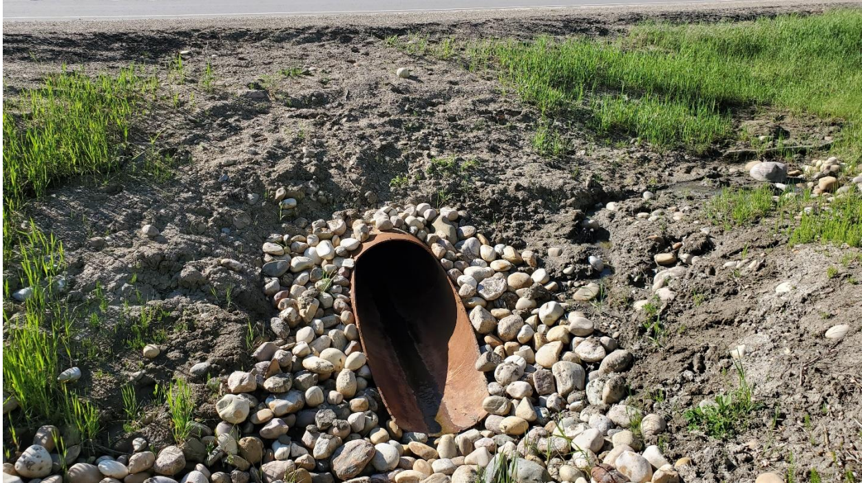
Photo 5 – Looking at inlet of new culvert at km 20.22. Note minor rill forming on the right-hand side of the photo.
