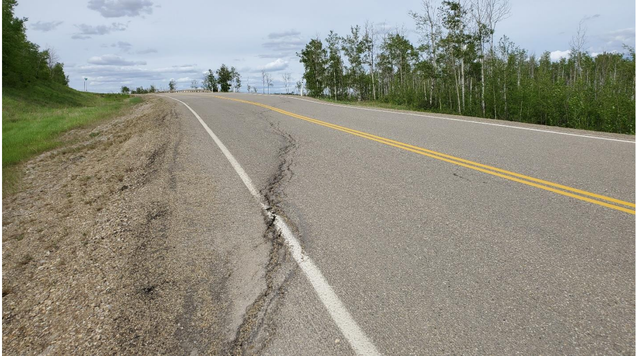
Photo 5 – Looking northeast at north scarp crack.
