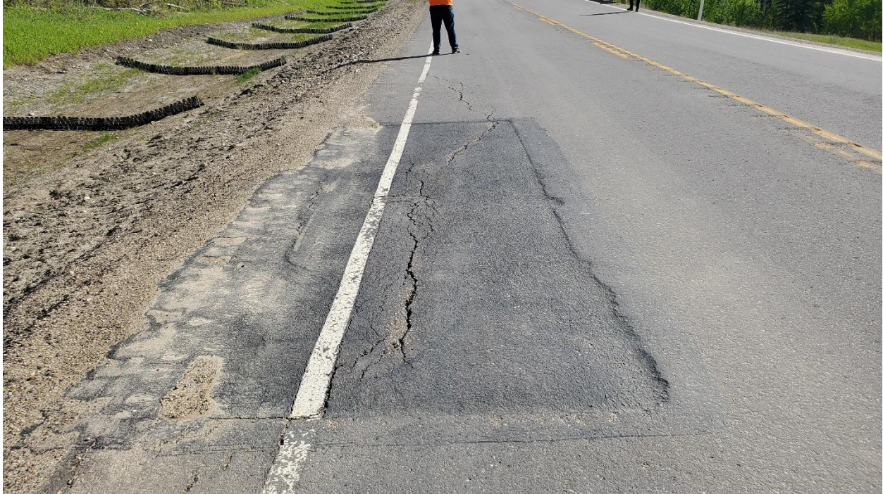
Photo 7: Scarp crack and rutting in a patch located in the SBL.
