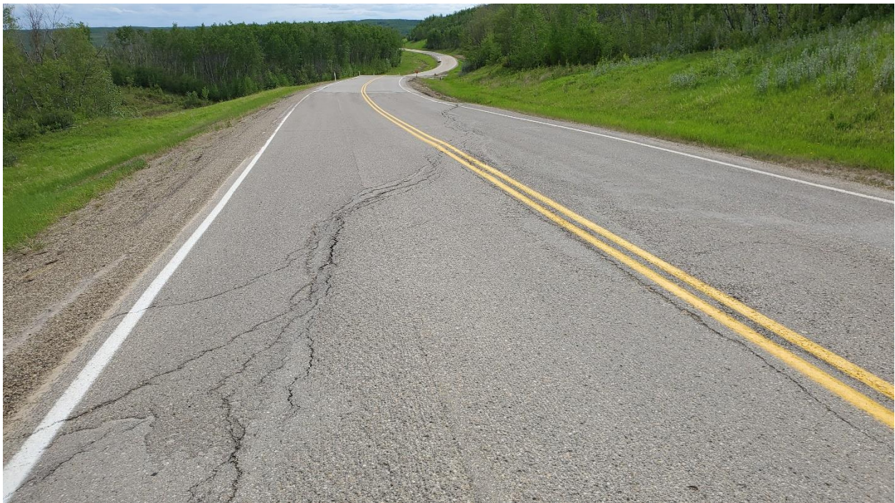
Photo 6 – Looking southwest at north scarp crack.
