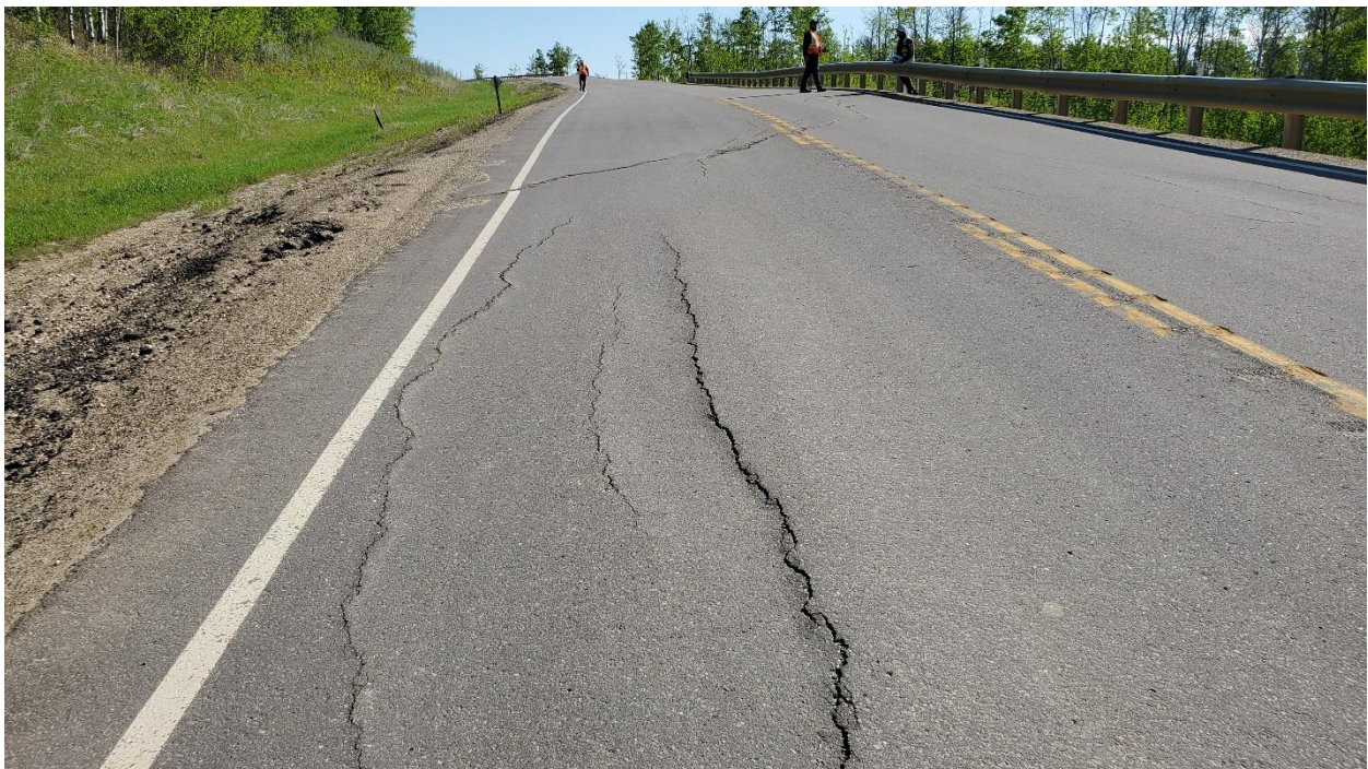
Photo 4: Looking northeast where main scarp crack crosses the highway at the central portion of Site 11.
