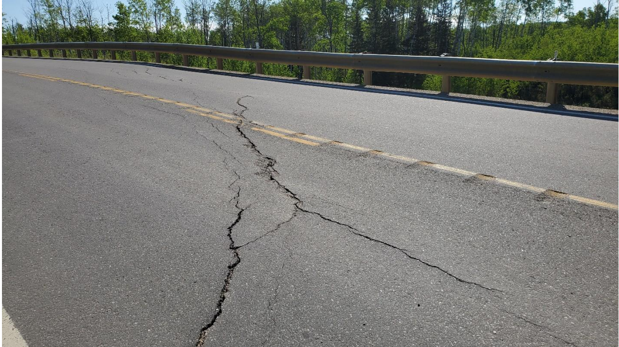
Photo 3 – Looking east at main scarp crack crossing highway (see Photo #4).
