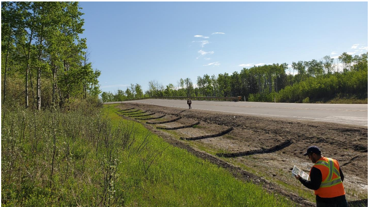
Photo 2 – Looking east highway at south end of site where previous significant gully was regraded and erosion control measures (matting and GeoRidges) were installed.
