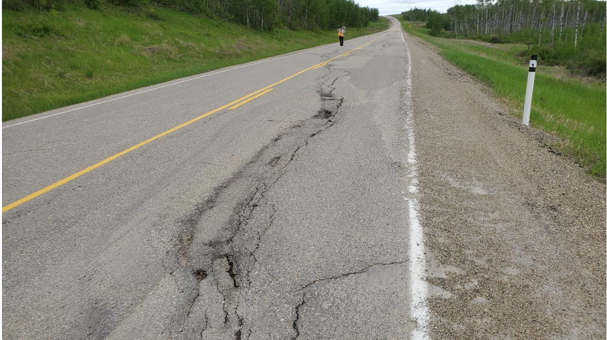
Photo 3, Site 12B: Looking north at deteriorating patch over crack at south end of site.
