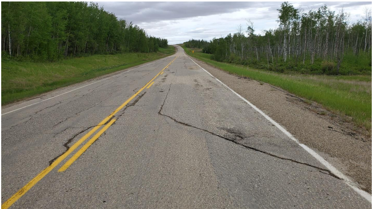
Photo 6, Site 12A – Looking north at crack forming along edge of toe berm excavation.
