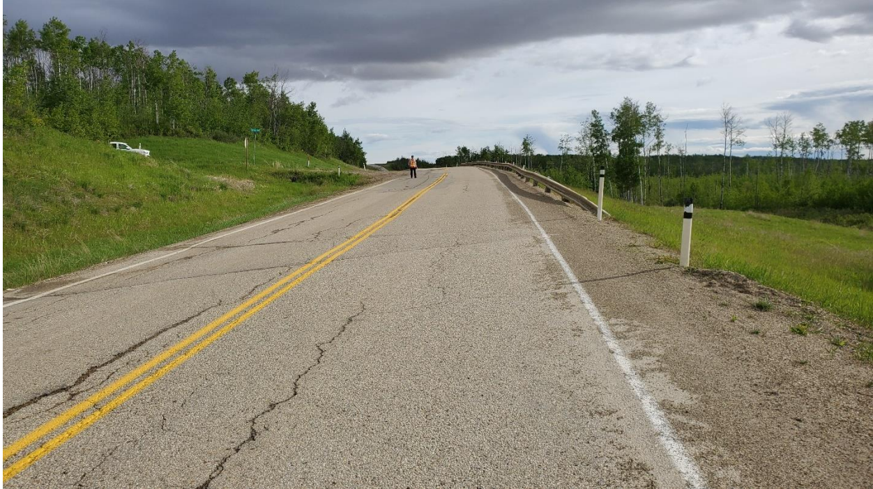
Photo 1, Site 12 – Looking northeast over toe berm. Note vertical and horizontal deformation of the guardrail.
