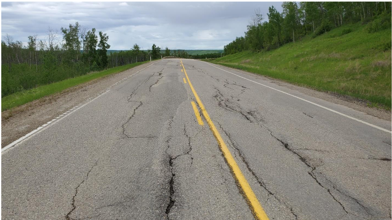
Photo 4, Site 12B – Looking south at main crack.
