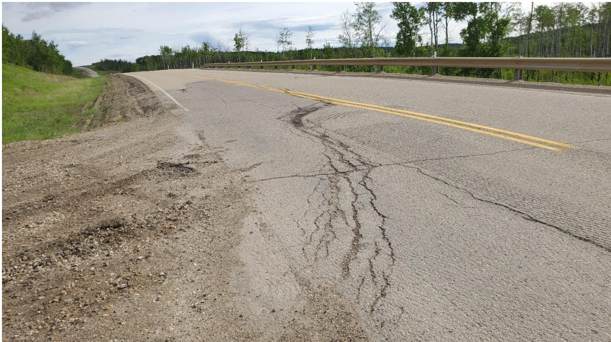
Photo 2, Site 12 – Looking north from TR764 intersection at main scarp crack.
