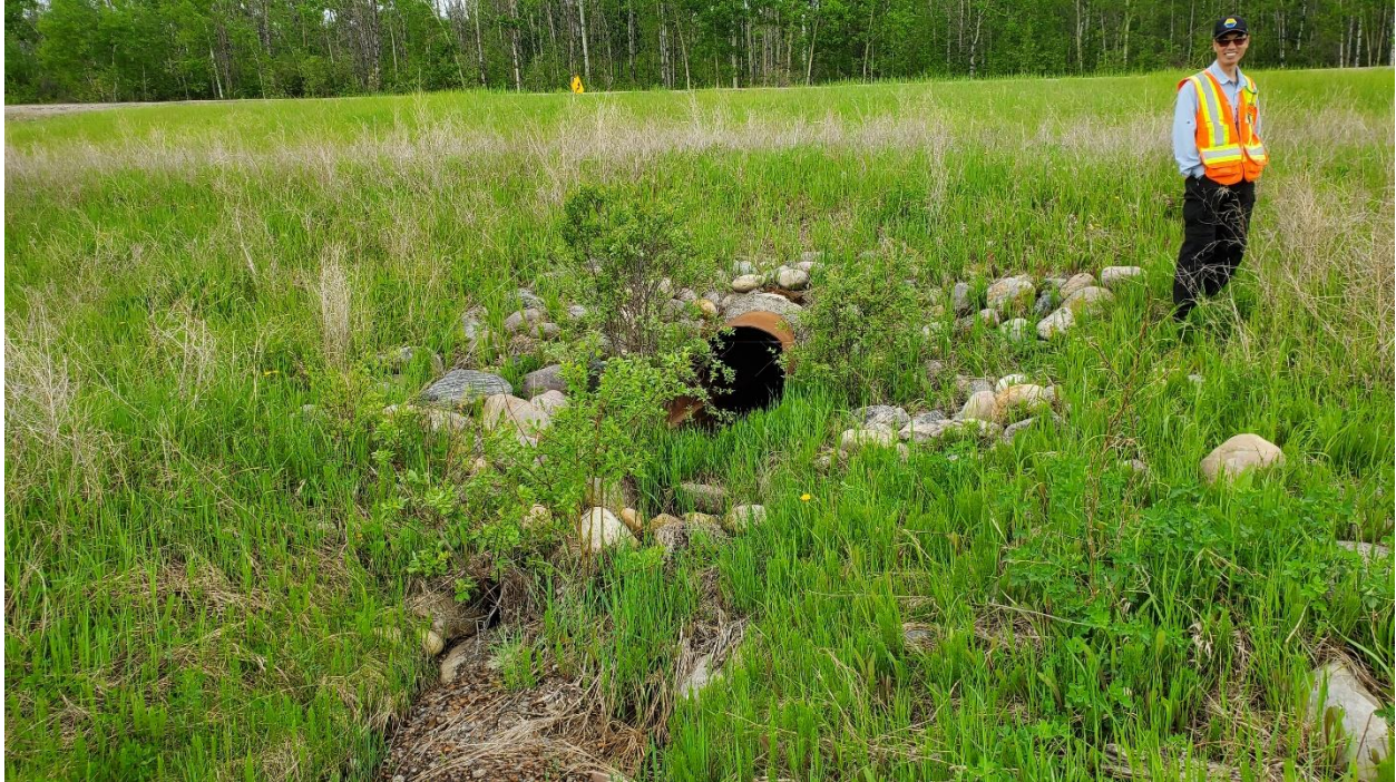
Photo 5, Site 12A – Rusting culvert liner outlet.
