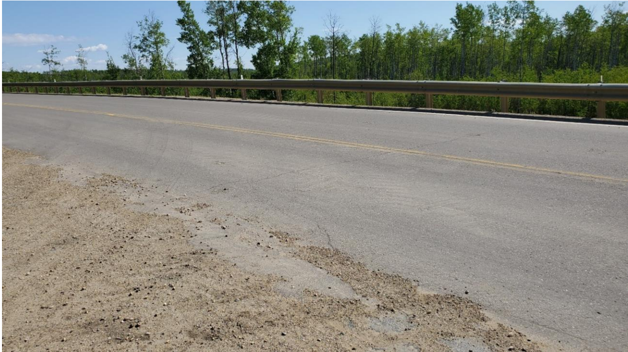
Photo 2, Site 12 – Looking south from north of the TR764 intersection at where the main scarp crack was located. It had just started reflecting through the new overlay.
