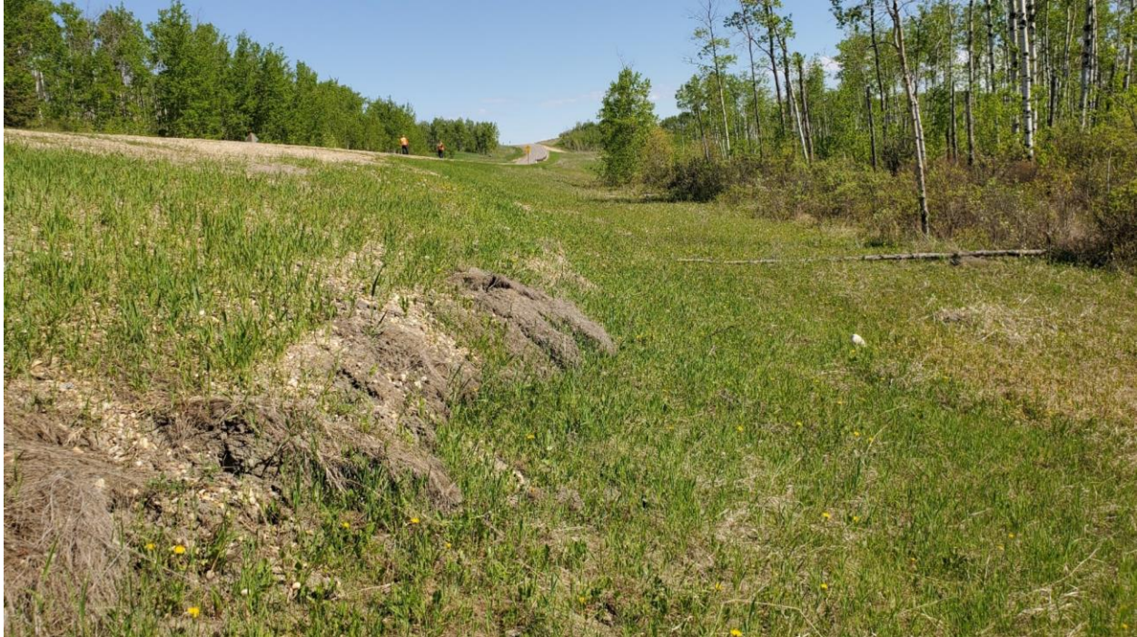
Photo 7, Site 12A – Looking north at potential toe roll on downslope slide where excess gravel appears to have been wasted on the sideslope.
