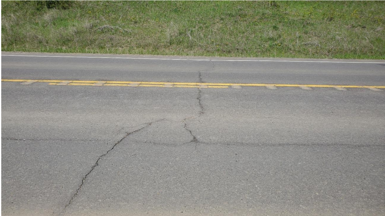
Photo 4, Site 12B – Looking west at the second transverse crack that has started reflecting through the new overlay.
