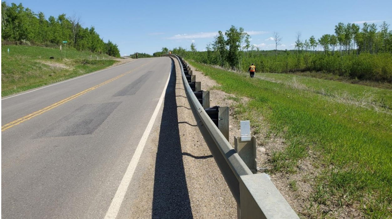
Photo 1, Site 12 – Looking northeast over toe berm. The guardrail was replaced in 2021 during the Highway 744 overlay project.
