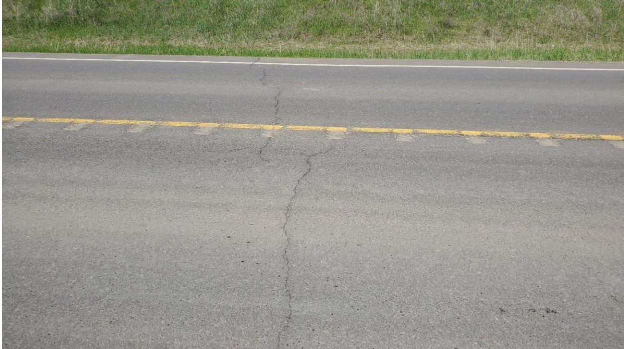
Photo 3, Site 12B: Looking west at one of the transverse cracks that has reflected through the new overlay near the south end of site.
