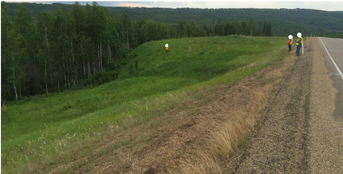
Photo 2 (looking north). The distance between the edge of the pavement and backscarp was unchanged from June 2013.
