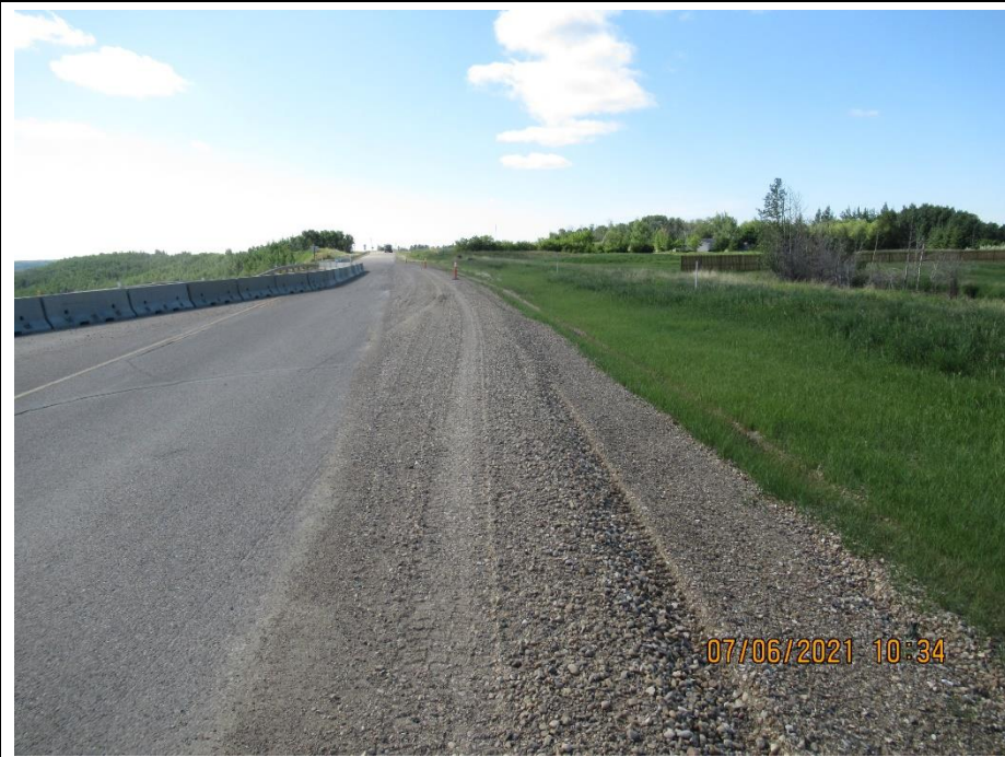
Photo 11. Looking south along the highway from the north end of the site (57+375) at the gravel detour constructed next to the SBL by Slide 1A.
