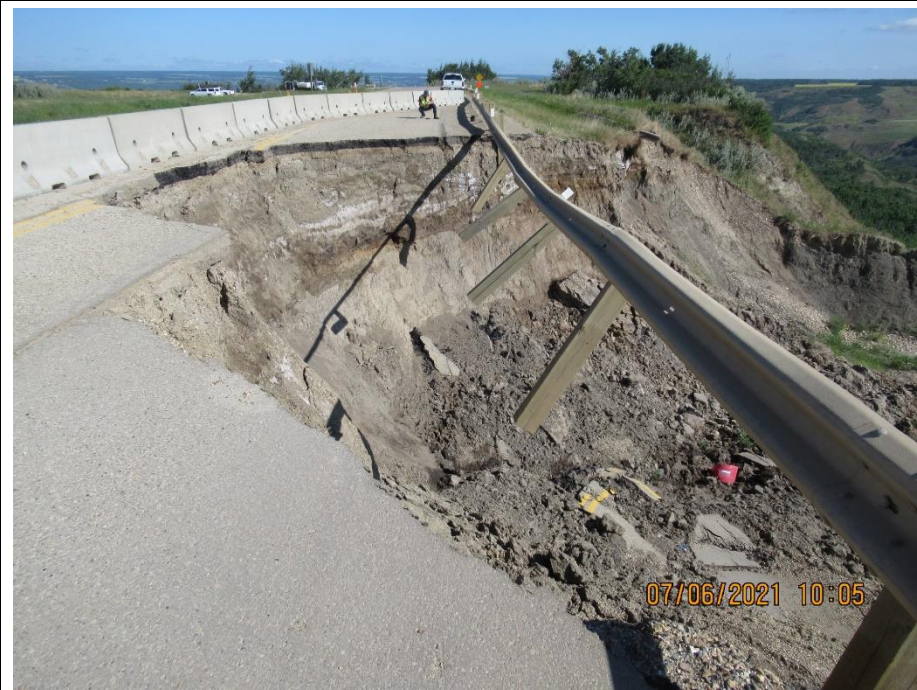
Photo 2. Looking north towards the Slide 1A bowl flank and main scarp south of Slide 1. The main scarp now has reached past the highway median. Six guardrail posts are freely hanging.
