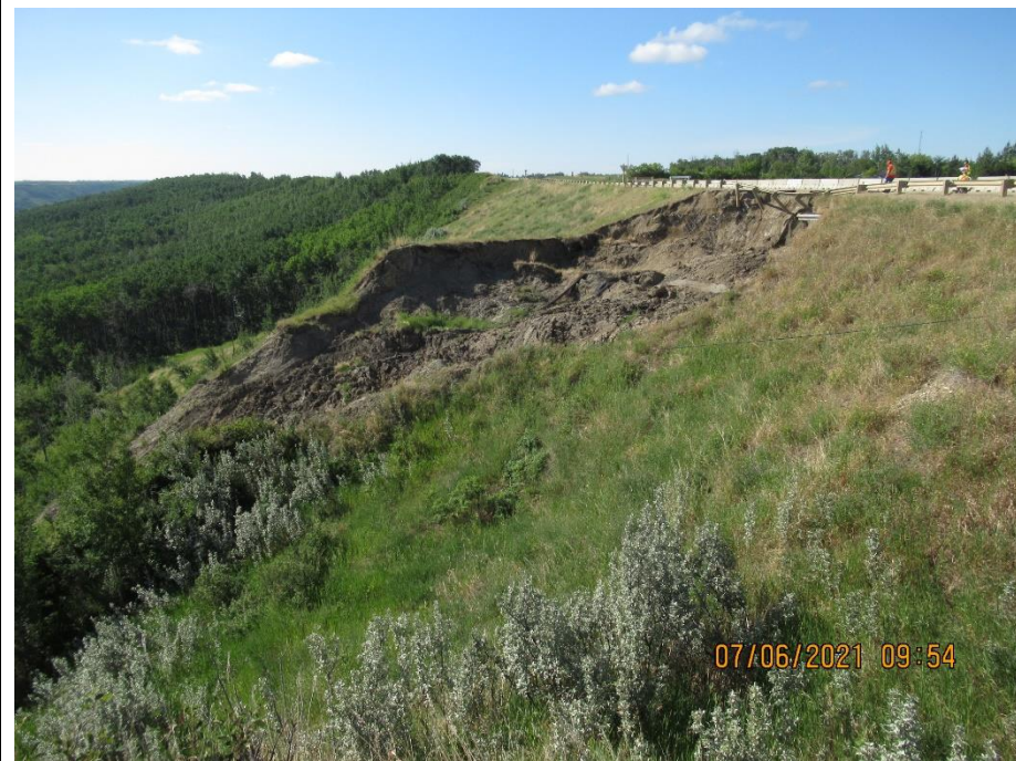
Photo 3. Looking at the south flank of the Slide 1A area. South flank area expanded since the previous inspection. North flank has had minor expansion within the upper slope relative to the previous inspection.
