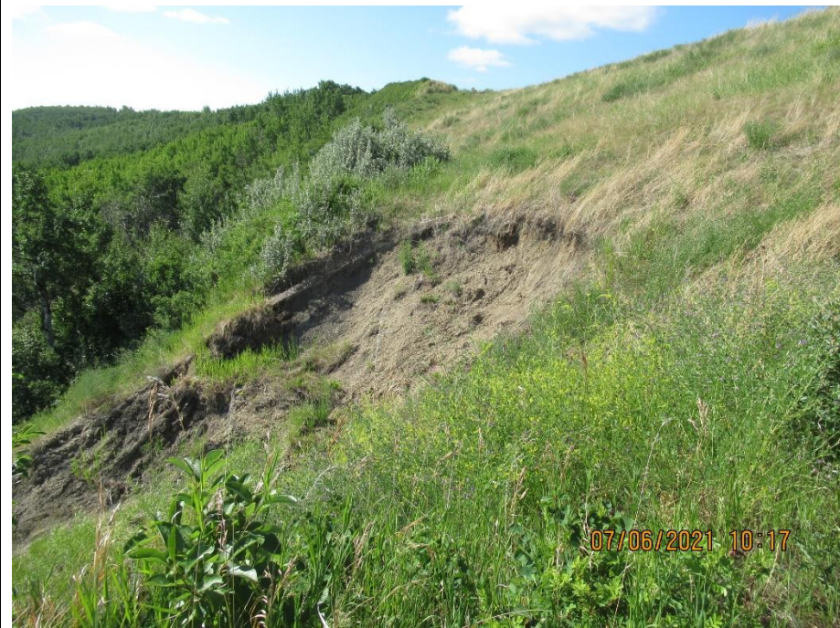
Photo 6. Looking southwest from north end of Heart River Landslide repair excavation (Former Slides 2, 3 and 4). Area has vegetated well through the Type B ECSC. Increased retrogression at the scarp and movement within the slide in the foreground.
