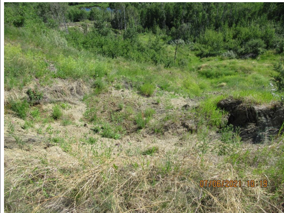
Photo 7. Looking east at mud flow at the location of former Slide 3, which has been more active since 2020. Decreased vegetation since previous inspection indicative of active soil movement.
