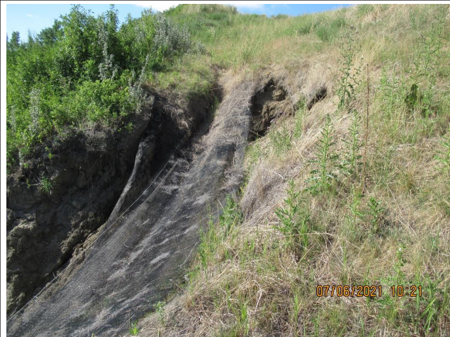
Photo 8. Looking south at the scour that has formed south of the former Slide 4. The scour is deeper and has ongoing erosion at the flanks since the 2020 inspection with evidence of recent earth flows.
