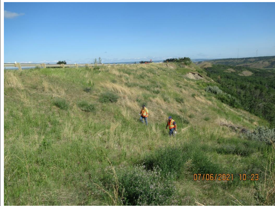
Photo 9. Looking northwest from south of the location of former Slide 4. Overall repairs from 2014 are performing well in this area. Overall slope is well vegetated and there are no apparent slumps in the granular backfill slope. No change from 2020.
