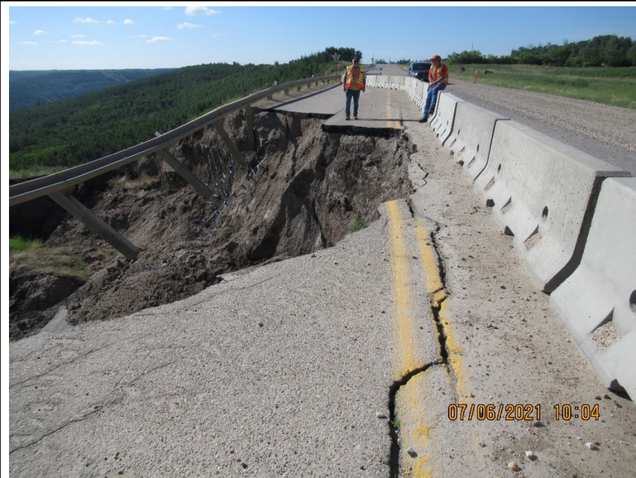
Photo 1. Looking south from south end of Slide 1 from the NBL shoulder of Hwy 744:04 towards the top of the Slide 1A bowl (57+300). The main scarp of the slide has retrogressed entirely into the NBL: and has reached just past the median strip. Gravel detour has been constructed to expand the SBL.
