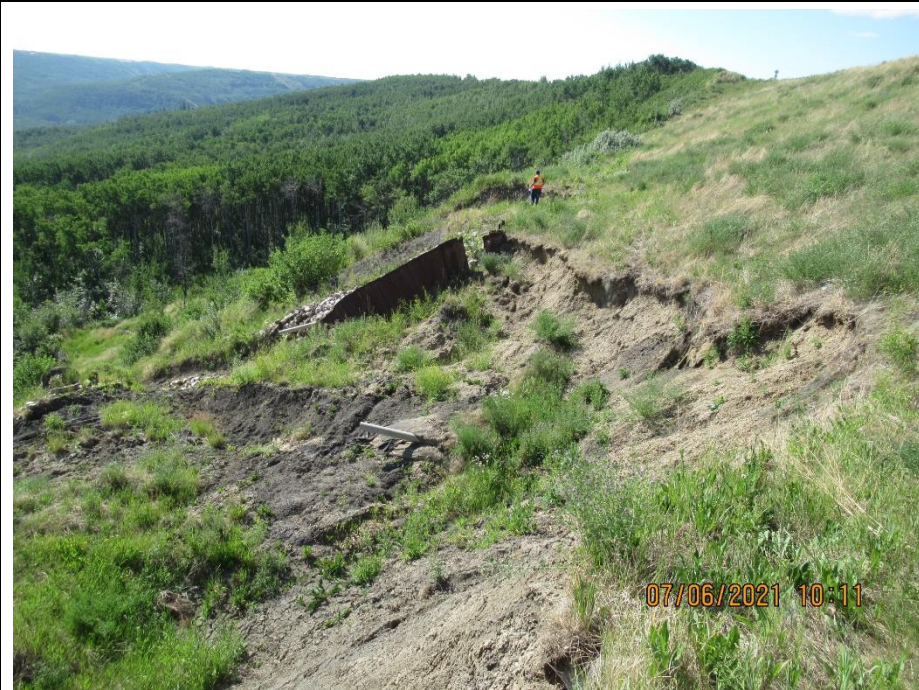
Photo 5. Looking southeast from north end of Heart River Landslide repair excavation (Former Slide 2). More slide / earth flow movement and main scarp retrogression has occurred since the previous inspection. The north end of the driven sheetpile has deflected further downslope.
