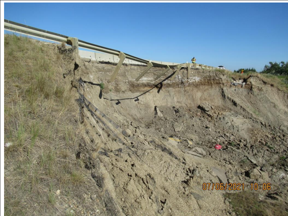
Photo 4. Looking towards the northwest at the main backscarp of Slide 1A. Note the wet soil horizon and dried water deposits from seepage.
