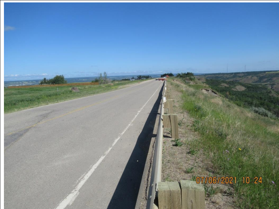
Photo 10. Looking north along the highway from the south end of the site (57+120). No apparent pavement changes south of Slide 1A. Note detour signage at Slide 1A.
