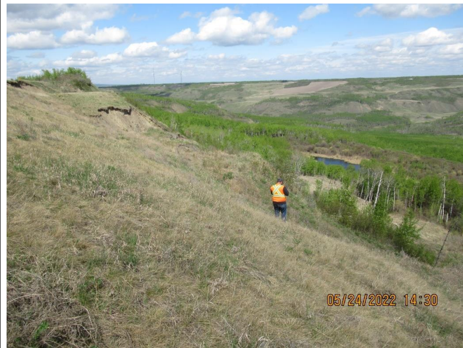
Photo 9. Looking northwest from south of the location of former Slide 4. Overall repairs from 2014 are performing well in this area. Overall slope is well vegetated and there are no apparent slumps in the granular backfill slope.
