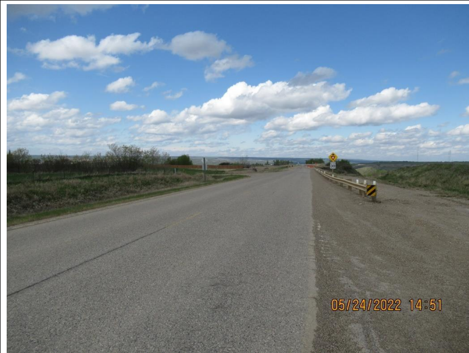
Photo 10. Looking north along the highway from the south end of the site. No apparent pavement changes south of Slide 1A. Note detour signage at Slide 1A.
