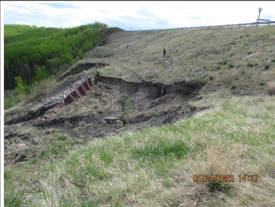
Photo 4. Looking southeast from north end of Heart River Landslide repair excavation (Former Slide 2). Ongoing downslope movement but no significant retrogression of the main scarp or further deflection of the sheet pile wall.
