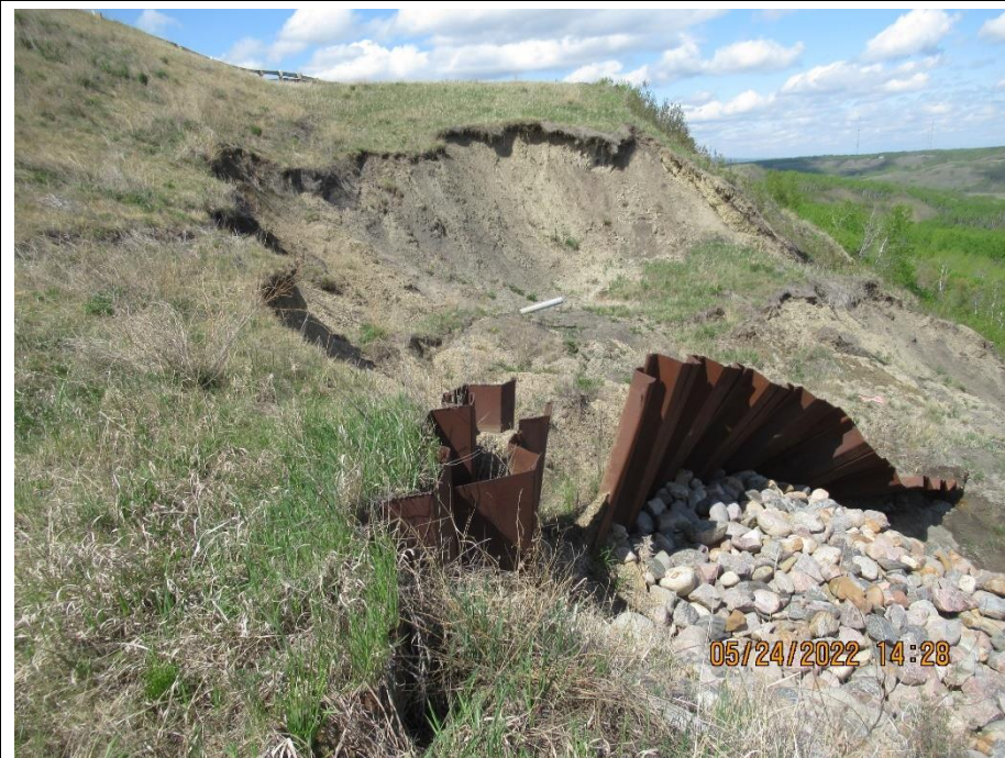
Photo 6. Looking north at the former Slide 2 area with ongoing slide movement and erosion damage. Some retrogression of the main scarp since 2021.
