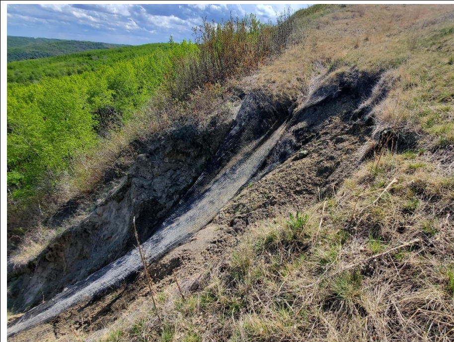
Photo 8. Looking south at the scour that has formed south of the former Slide 4. Ongoing erosion since 2021.
