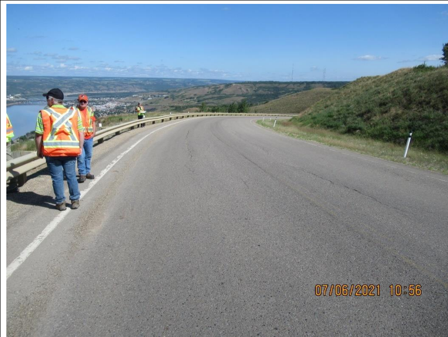
Photo 4. Looking northwest along from SBL of Hwy 744:04 at km 57.6 at south end of realignment done in 2015-2016. Minor longitudinal cracking that is largely unchanged since 2020.
