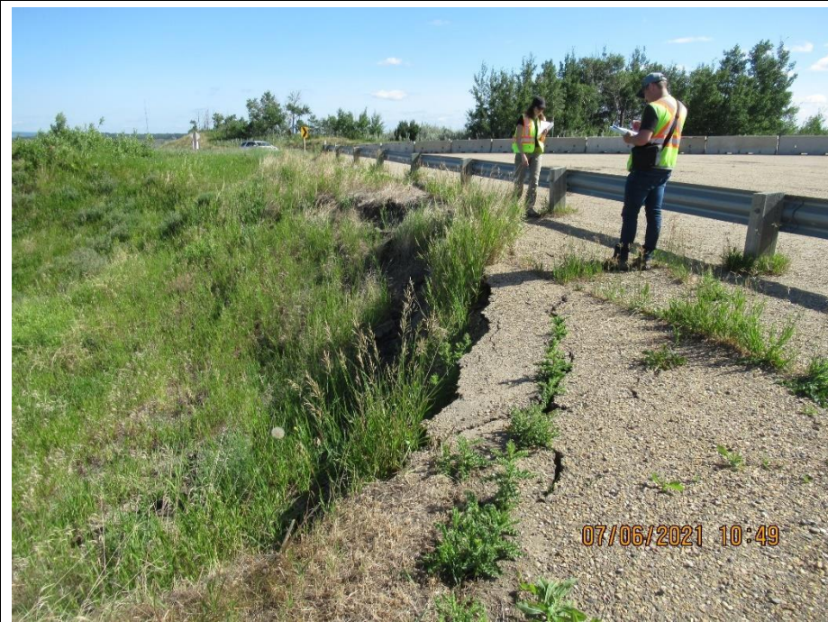
Photo 2. Looking northeast along backscarp of Slide 2 which is 1.3 m from the parking lot guardrail. Some minor localized main scarp retrogression, flank retrogression and additional pavement cracking since 2020.
