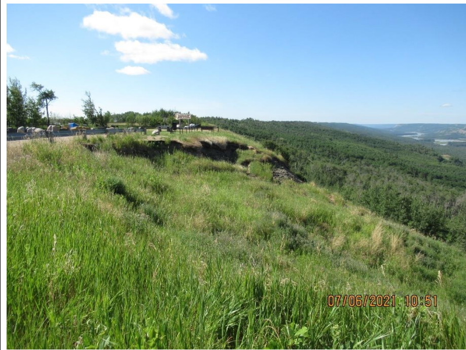
Photo 3. Looking southwest towards the upper part of Slides 2 and 3. Some minor retrogression and movement in the flanks and movement of the disturbed slide mass since 2020. Disturbed slide mass area is well vegetated.
