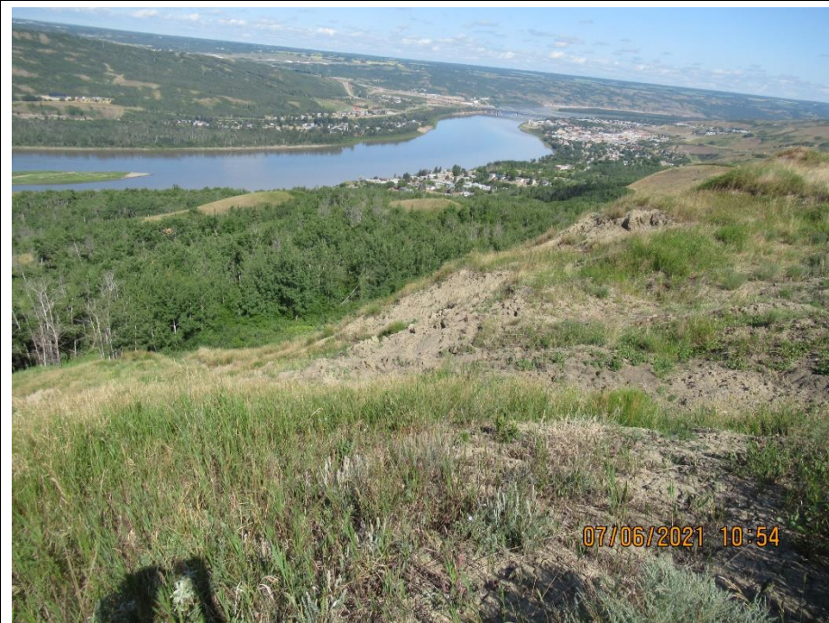
Photo 6. Looking northwest from downslope of the SBL of Hwy 744:04 at km 57.63. Additional downslope movement apparent within disturbed slide mass.
