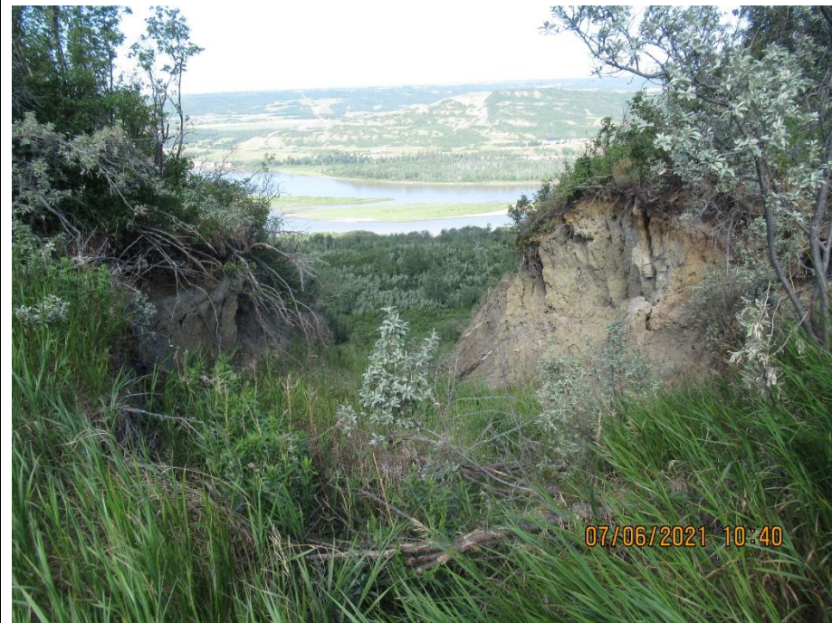
Photo 8. Looking at the top an erosion gully located at the southern edge of the site, approximately 50 m south of the Slide 4 area. Gully is offset approximately 70 m west of the highway.
