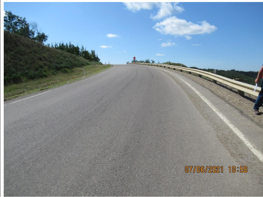
Photo 7. Looking south along SBL of Hwy 744:04 at km 57.68. Some additional minor longitudinal cracking noted in the NBL.
