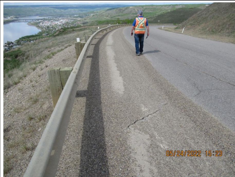
Photo 4. Looking northwest along from SBL of Hwy 744:04 at km 57.6 at south end of realignment done in 2015-2016. New transverse cracks have formed joining the previous longitudinal crack in the NBL to form arc-shaped crack within the downslope slide extents.
