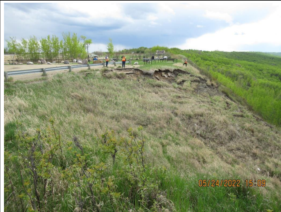
Photo 3. Looking southwest towards the upper part of Slides 2 and 3. Visible retrogression and movement in the main scarp and upper southern flank since 2021. Disturbed slide mass area is well vegetated.
