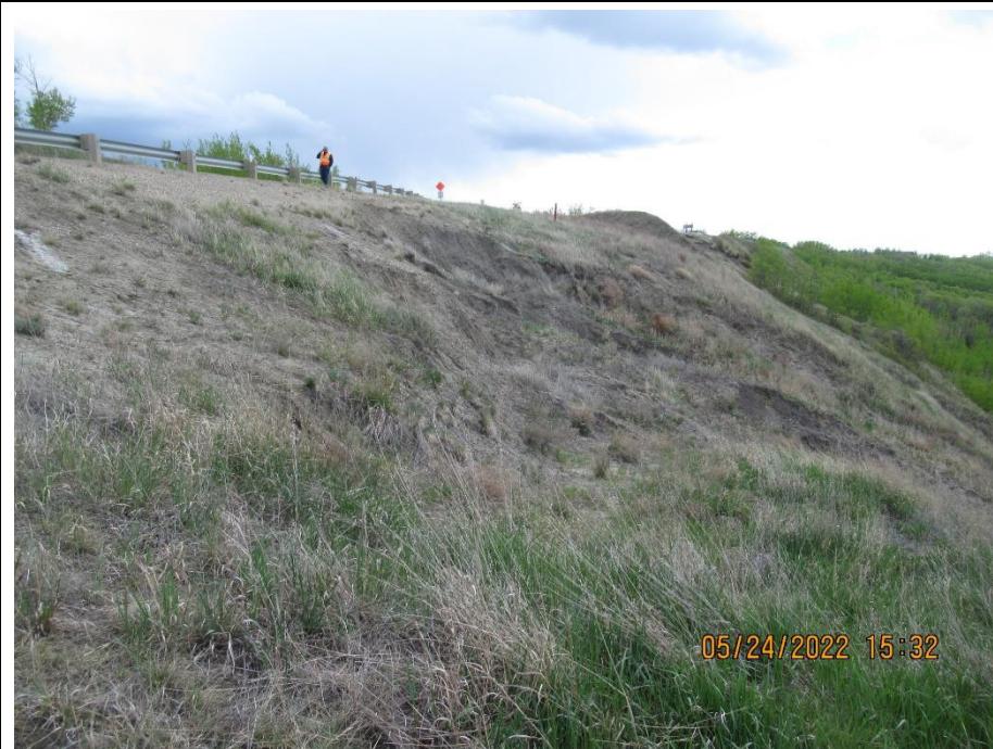
Photo 6. Looking south at the active slide near km 57.65. Ongoing retrogression and erosion at the main scarp and south flank.
