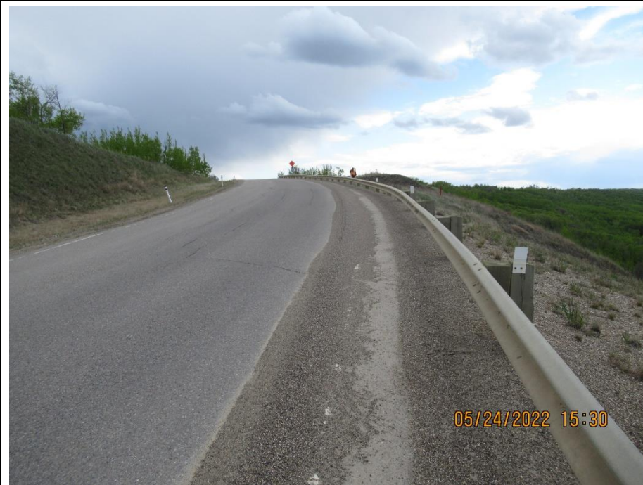
Photo 7. Looking south along SBL of Hwy 744:04 at km 57.68. New transverse cracks have formed joining the previous longitudinal crack in the NBL to form arc-shaped crack within the downslope slide extents.
