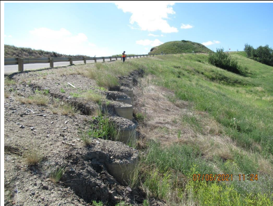
Photo 5. Looking south along the west side of Hwy 744:04 at protruding piles near km 57.9. Max drop of 1.8 m below top of pile.
