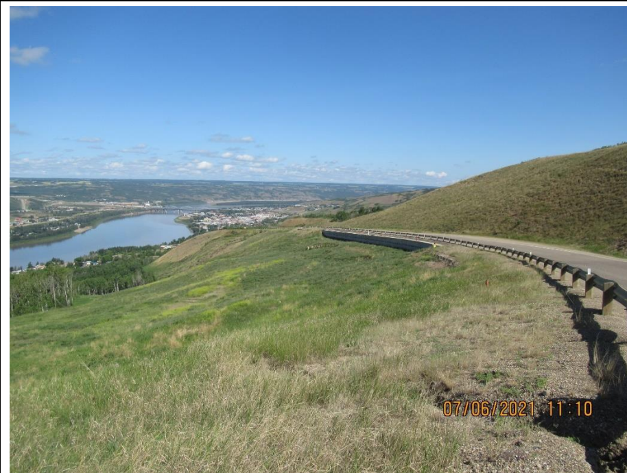
Photo 2. Looking north along the west sideslope of Hwy 744:04 at km 57.94 below the old pile wall.
