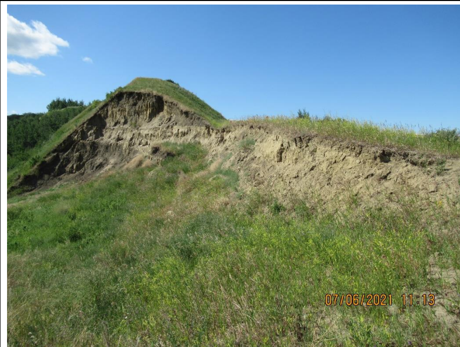
Photo 4. Looking south along the backscarp of the landslide at the top of the Heart River valley on Hwy 744:04 at km 57.85. North end of the slide area has less movement relative to the southern end.
