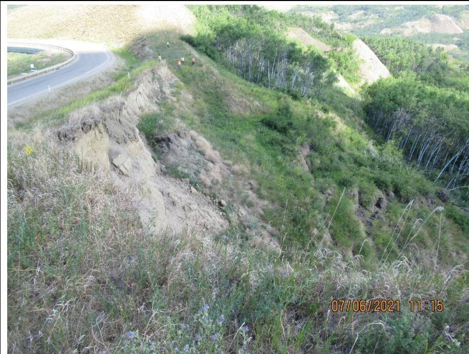
Photo 3. Looking northeast along the backscarp of the landslide at the top of the Heart River valley on Hwy 744:04 at km 57.8. Slide area has active movement within the disturbed scarp face leaving a higher backscarp since the previous inspection. Minor retrogression towards the road. The abandoned ATCO pipeline has been removed.
