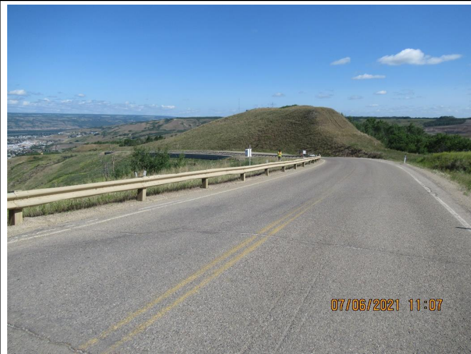
Photo 7. Looking north along Hwy 744:04 from km 57.8 at the crack and dip across the road.
