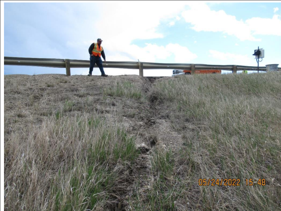
Photo 8. Drainage erosion from the west side of the road near KM 58.86 that has become worse relative to the 2021 condition.
