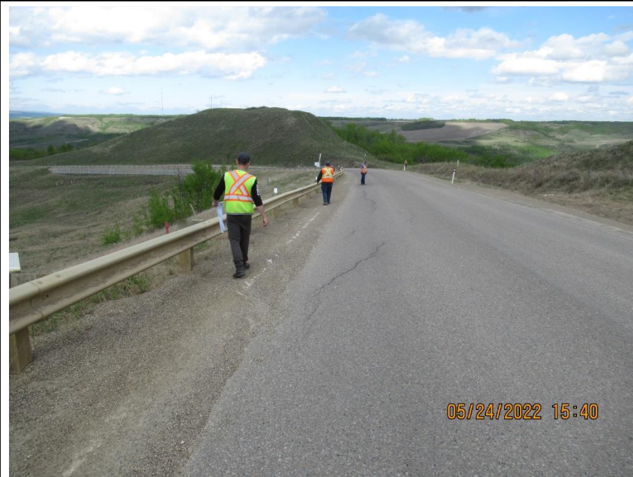
Photo 1. Looking northeast along the centerline of Hwy 744:04 at km 57.75 at the north end of the 2014-2015 realignment. Cracks have become more apparent and there was increased localized settlement at the shoulder relative to the 2021 condition.
