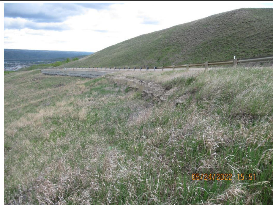
Photo 5. Looking north along the west side of Hwy 744:04 at protruding piles near km 57.9. Max drop of 1.8 m below top of pile.
