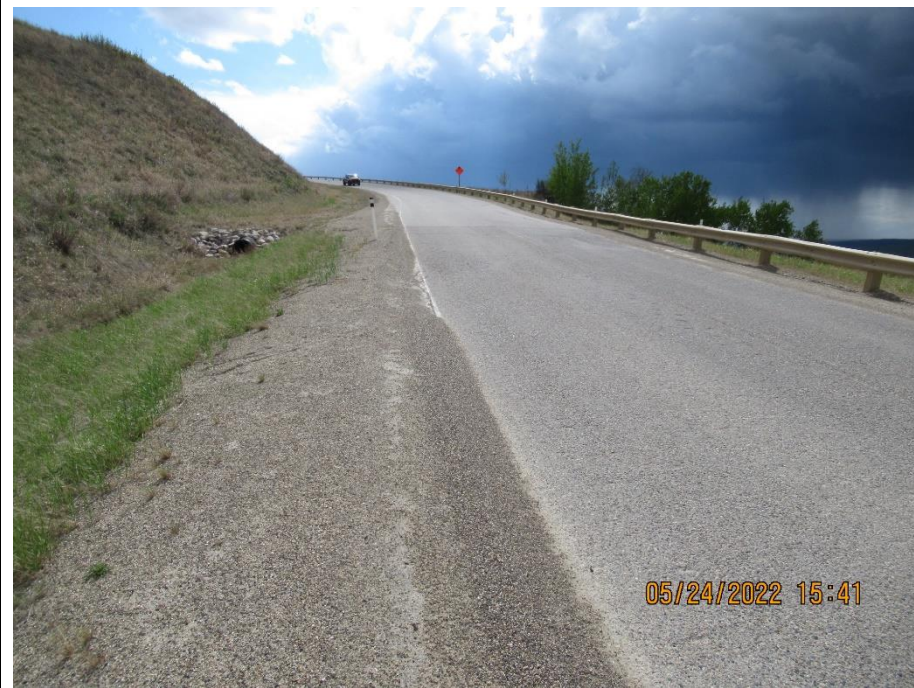
Photo 7. Looking southwest along Hwy 744:04 from km 57.85 at the crack and dip across the road.
