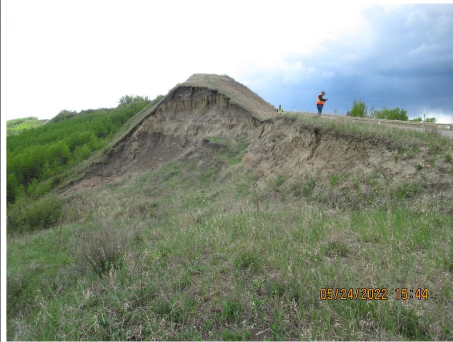
Photo 4. Looking south along the backscarp of the landslide at the top of the Heart River valley on Hwy 744:04 at km 57.85. Larger buildup of soil at base of vertical scarp, indicative of ongoing erosion but no major retrogression since 2021.
