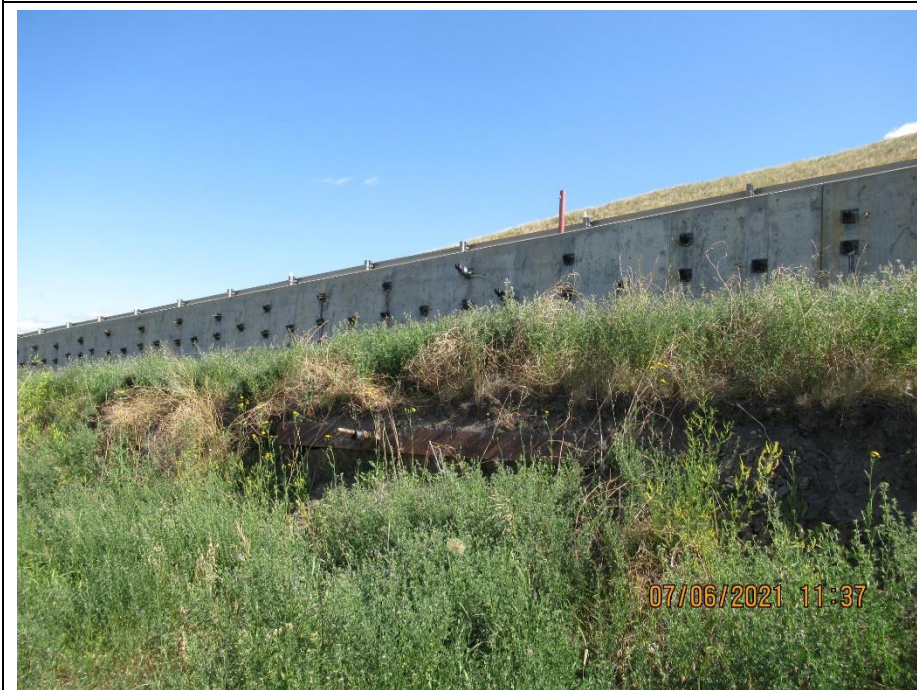
Photo 4. Looking northeast from below the north end of the km 58 pile wall. The old landslide scarps below the pile wall that were regraded in 2015 have ongoing movement. Additional old tieback and waler was exposed from the movement at the south end. Highest drop was 2.0 m from the top of the exposed piles.
