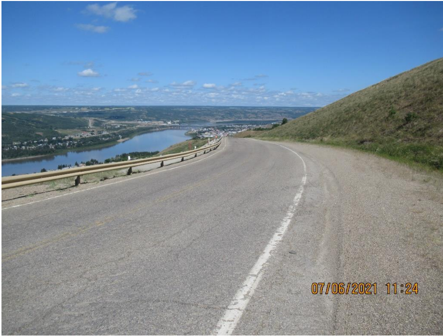
Photo 1. Looking northwest from the SBL shoulder of Hwy 744:04 at km 57.96 along the guardrail above the km 58 pile wall. There has been no major changes in the cracks in the ACP since 2020.
