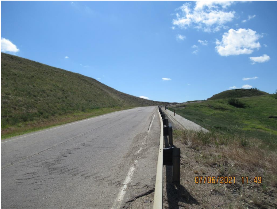
Photo 7. Looking south from the north end of the km 58 pile wall. Slightly worse crack and dip within the ACP directly behind the wall but overall road condition has not significantly changed since the 2020 condition.
