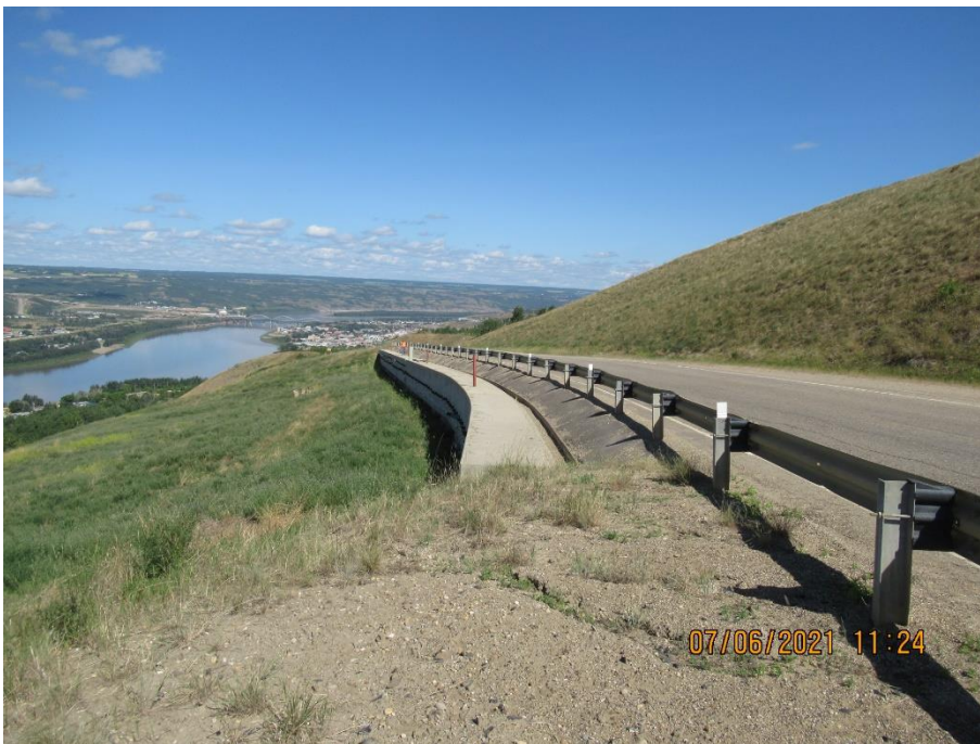
Photo 2. Looking northwest from the south end of the km 58 pile wall. The ACP shoulder protective cover was in good condition. No significant changes were noted downslope of the wall at this site relative to the 2020 condition.
