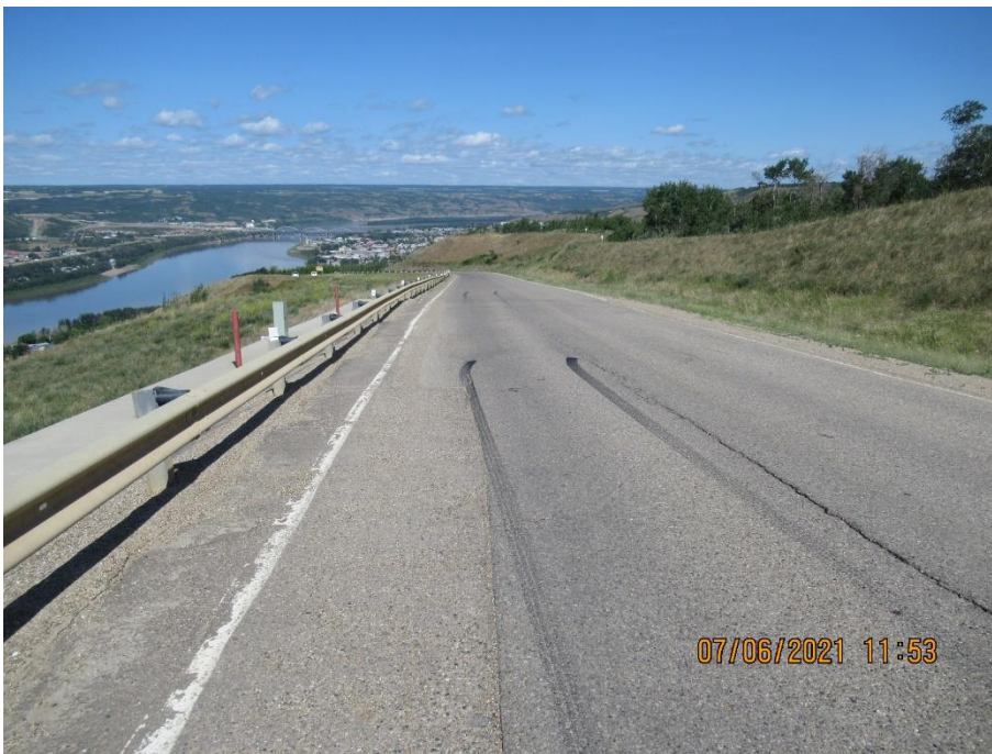
Photo 8. Looking northwest at the highway above the "Makeout" pile wall. No major change to the dip around the SBL shoulder near the middle of the wall or ACP cracking relative to the 2020 condition.
