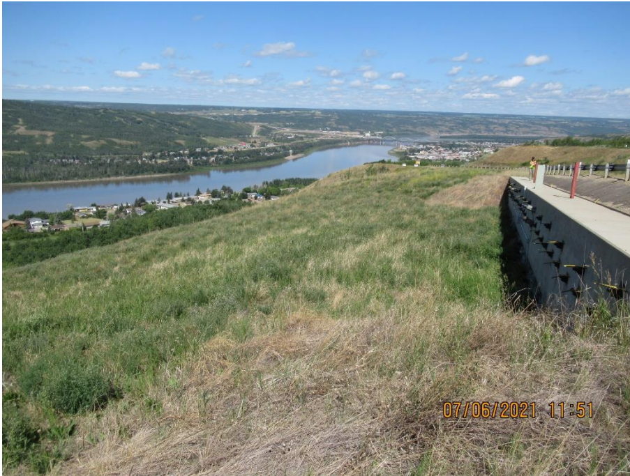
Photo 9. Looking north at the bench and graded area below the “Makeout” pile wall. Area appeared in good condition and had no observable changes from 2020.
