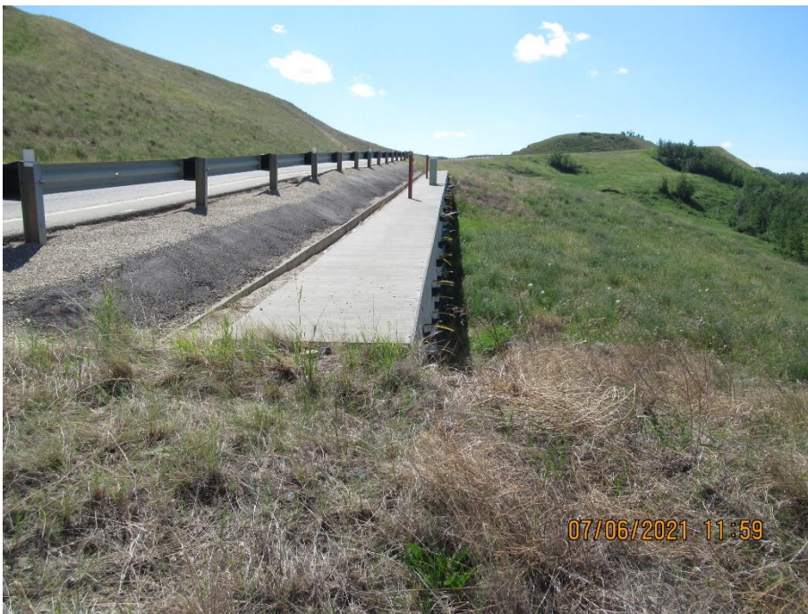
Photo 10. Looking south along the top of the “Makeout” pile wall. ACP shoulder protective cover was in good condition. Drainage trough was relatively clear and functioning.
