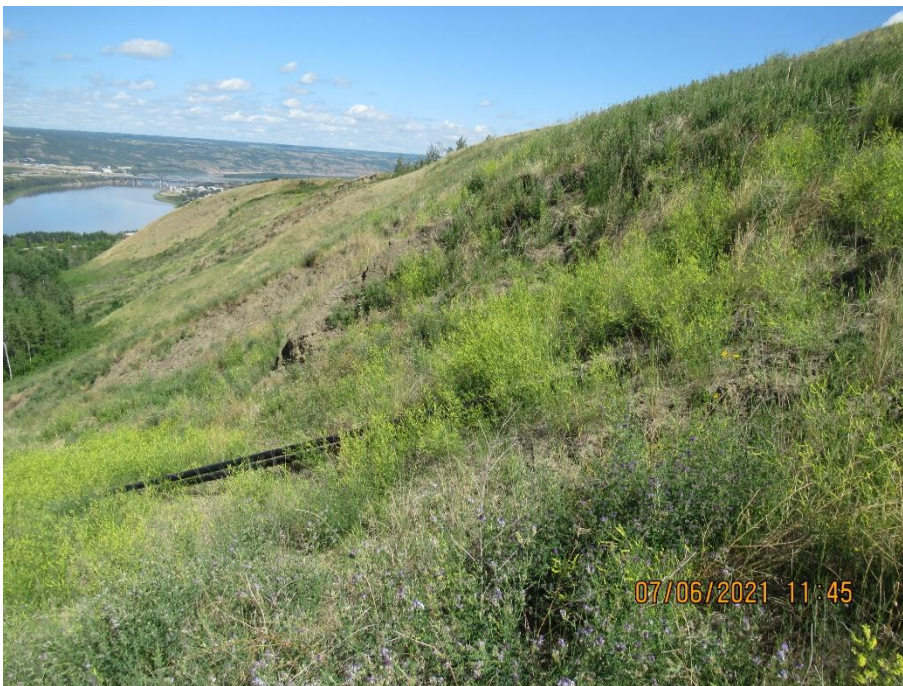
Photo 6. Looking at the north flank of the lower slide area between the pile walls. Seepage from a disconnected drainage pipe is causing erosion and exacerbating slide movement.
