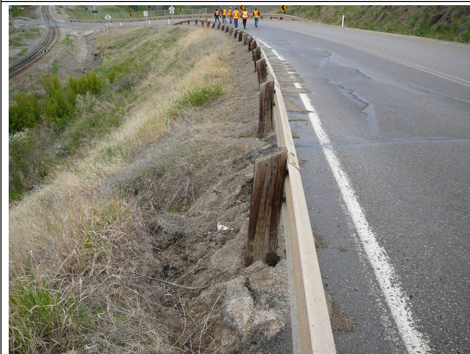
Photo 8. Erosion on the road shoulder due to drainage off the road. Also note the cracking along the road.
