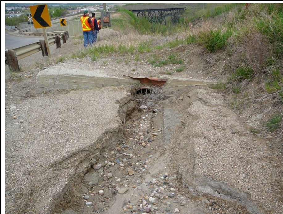
Photo 9. Inlet to the CNR Trunk down drain – the inlet is partly clogged, and requires maintenance.
