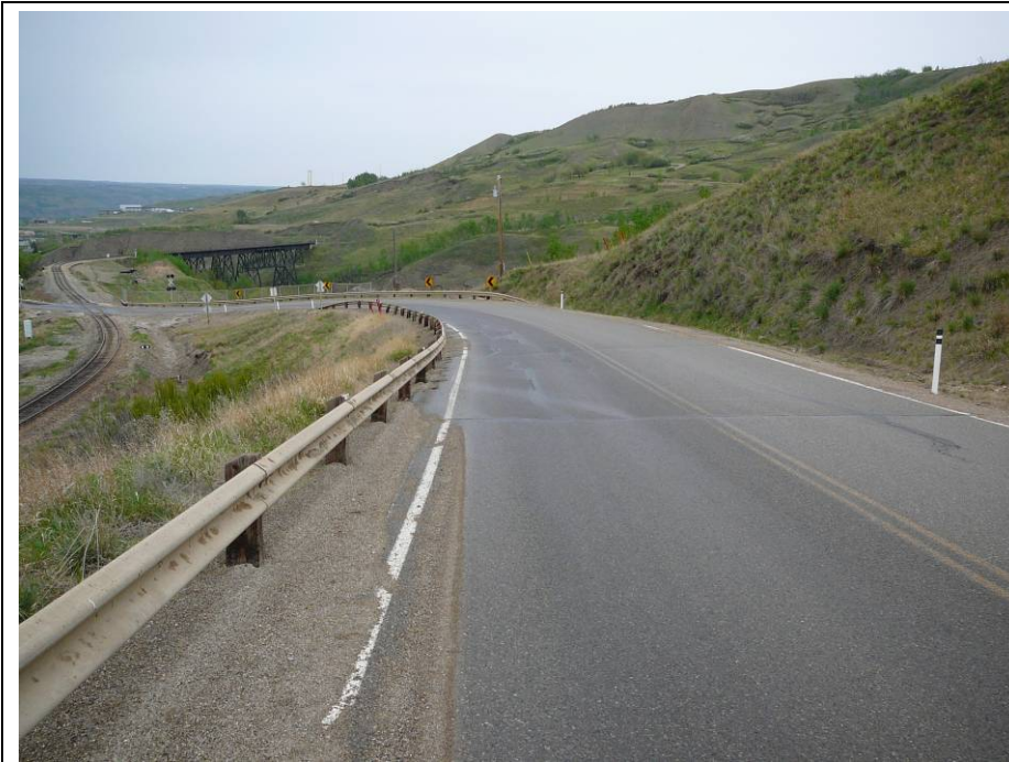
Photo 7. Some cracking in the road on the inside of the bend on the approach to the CNR crossing.
