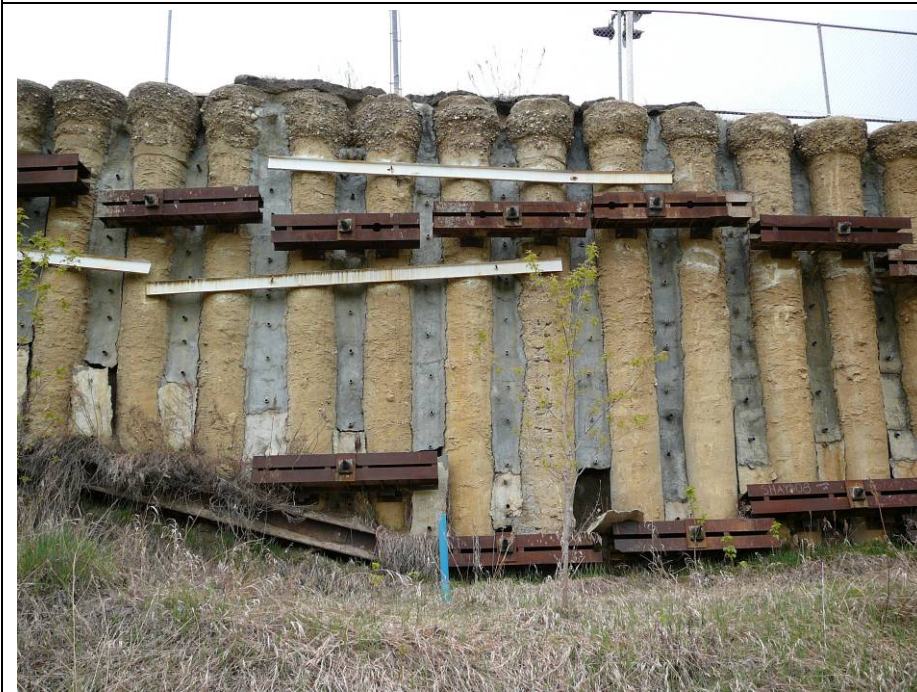
Photo 10. Looking up at the CNR retaining wall. There are portions of parging between the piles that has spalled. There isn't evidence that significant soil is being lost from between the piles.
