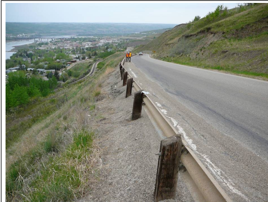
Photo 5. Cracking in the road and erosion / sloughing of the road shoulder, north of km 59.
