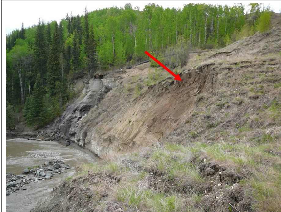
Photo 12. Toe of the slope below the CNR pile wall. Significant additional slide movement has occurred, particularly at the south end of the failure. There was an area of active slide movement during the inspection (arrow).
