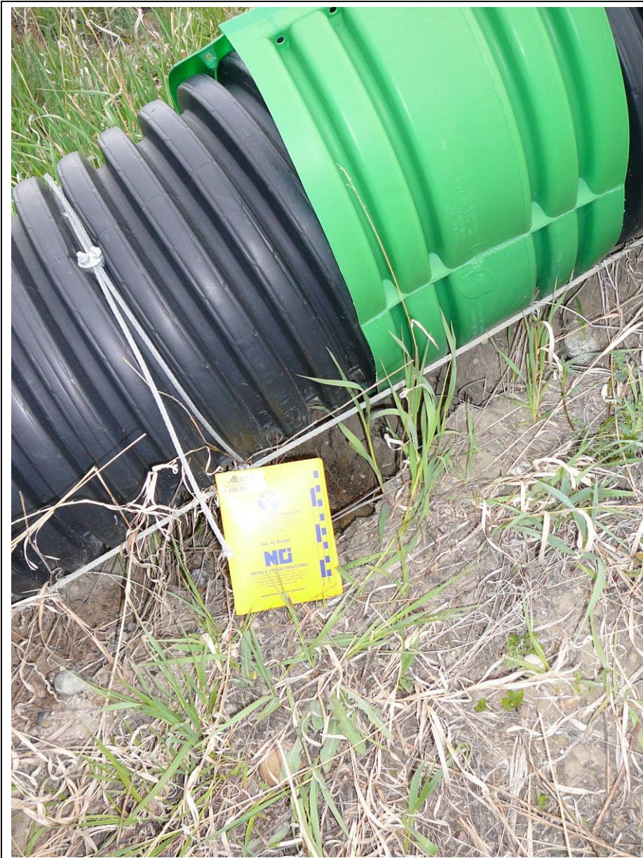
Photo 3. All of the band couplings on the Judah Trunk down drain have failed. At the uppermost band coupling, erosion under the drain has worsened.
