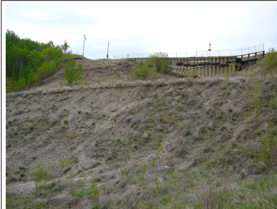
Photo 11. Backscarp of slide in the toe berm in front of the CNR pile wall. The backscarp has not retrogressed significantly since 2008.
