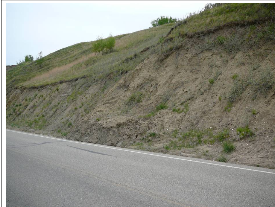
Photo 6. New skin failure in the upslope road cut. The failed material partially blocks the ditch and should be removed.
