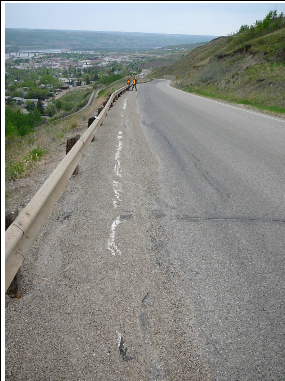
Photo 4. Cracking along the downslope road shoulder has worsened since 2008.
