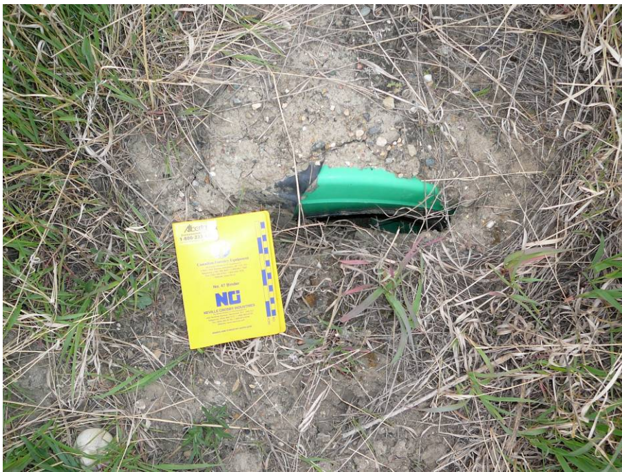
Photo 2. Connection between the culvert and the down drain has failed, and should be repaired.
