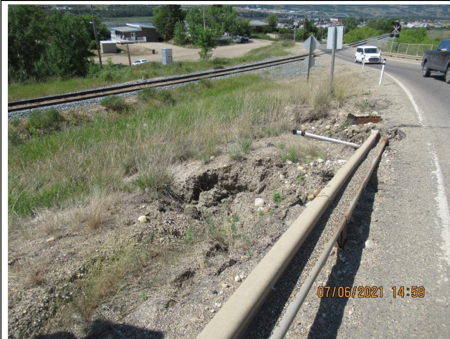
Photo 10. Looking west at erosion rills and ACP shoulder damage in the embankment near KM 59.53. Slightly worse from previous inspection.
