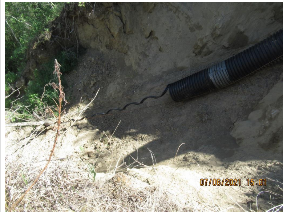
Photo 4. Looking east at break in CNR CPP Trunk pipe and erosion gully at crest of the Heart River valley slope.
