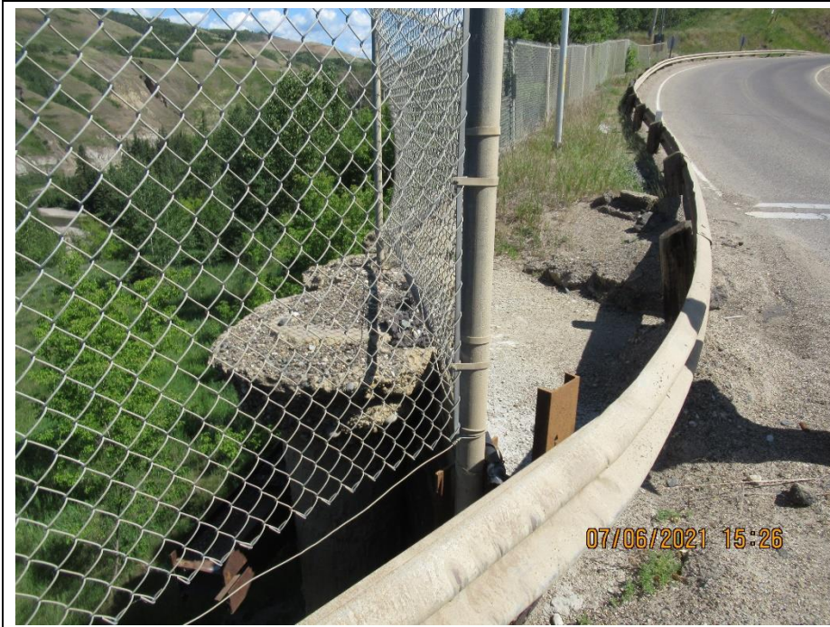
Photo 2. Repaired area above the piles where a void formed from soil loss between the two northernmost piles at the CNR pile wall along the NBL shoulder of Hwy 744:04 at km 59.62 was backfilled with concrete. Repair was in good condition.
