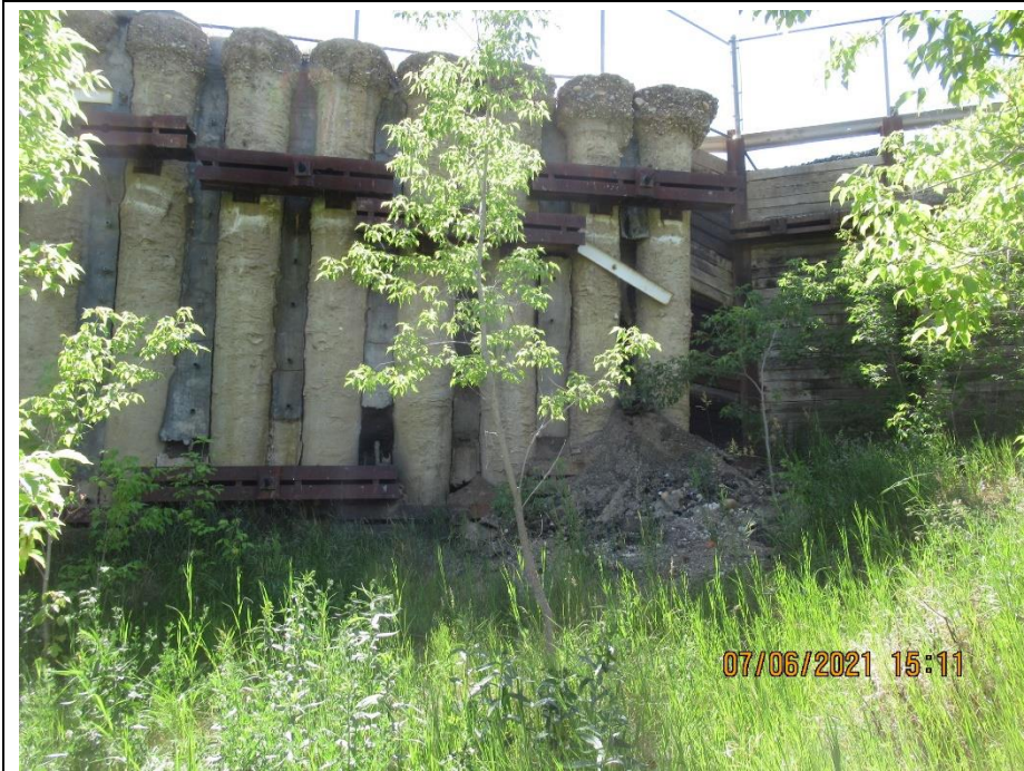
Photo 3. Looking south at the soil loss between the northernmost piles of the CNR pile wall north of Hwy 744:04 at km 59.61. Increased buildup of soil and concrete spalling between the piles since 2020.
