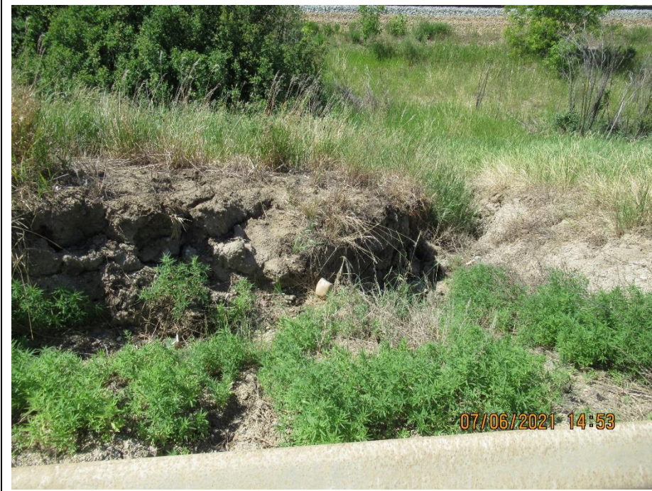
Photo 9. Looking west at erosion gully in the embankment near KM 59.48. Expanded from previous inspection.
