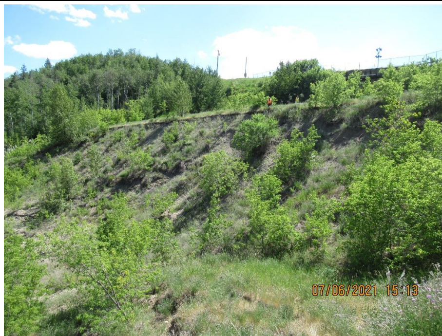
Photo 6. Looking southeast from the north side of the lower slide. No major changes observed in the slope area below the pile wall since 2020.
