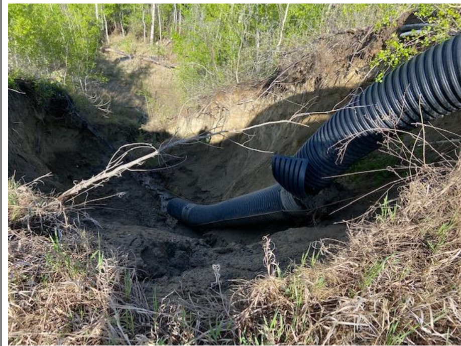
Photo 4. Looking northeast at break in CNR CPP Trunk pipe and erosion gully at crest of the Heart River valley slope.
