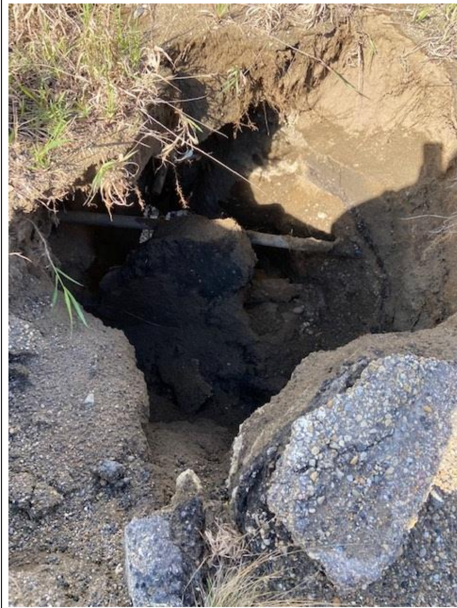
Photo 2. View into the new erosion void behind the pile wall. Void has been created as a result of soil loss between the piles. Void was 3 x 2 m wide in size and over 5 m deep. The void 'bridged' to the other void repair area to the west.
