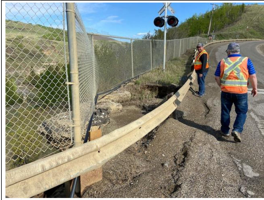
Photo 1. Looking southeast from the north end of the CNR pile wall. A new erosion void has opened up behind the wall adjacent to the previously repaired void area.
