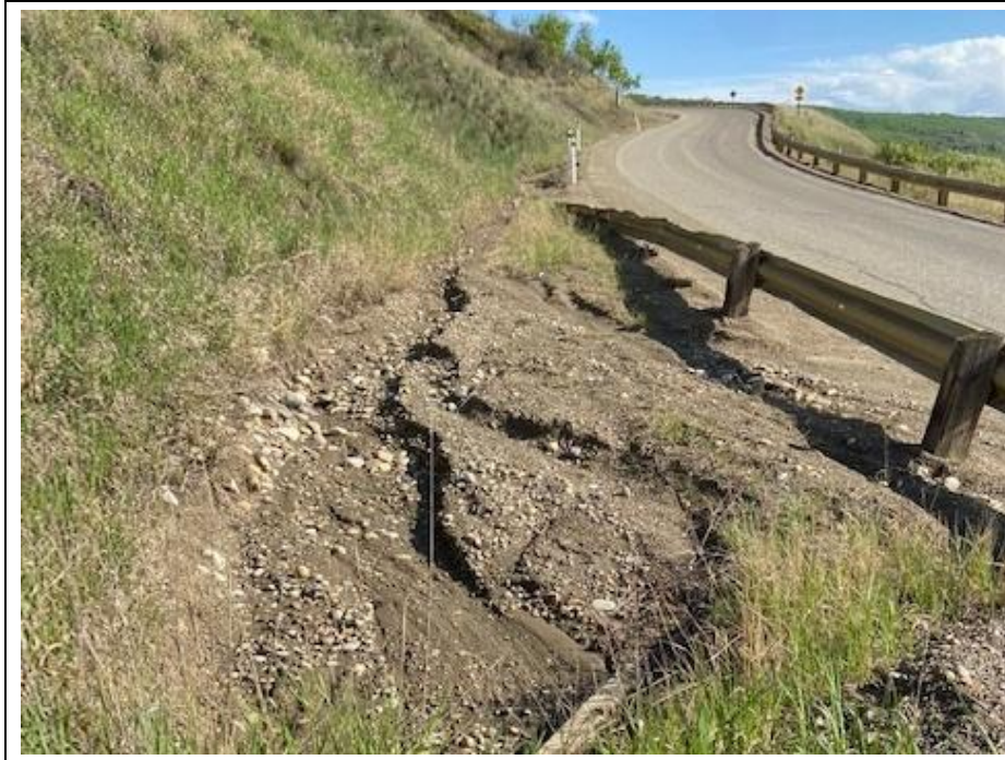
Photo 8. Looking south towards the erosion in the east ditch upslope from the draining pipe inlet.
