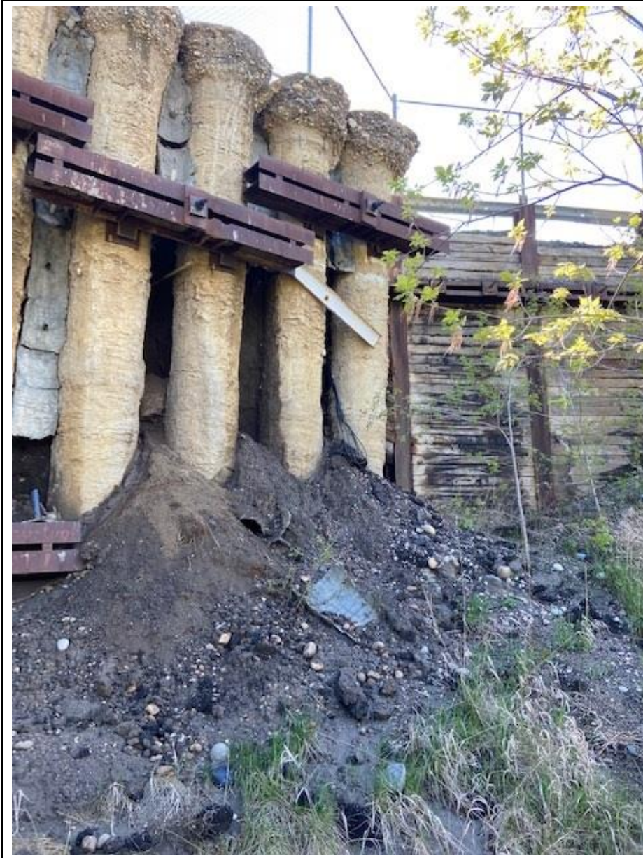
Photo 3. Looking south at the soil loss between the northernmost piles of the CNR pile wall north of Hwy 744:04 at km 59.61. Increased buildup of soil and concrete spalling between the piles since 2021 that has resulted in an open void at the surface between the wall and the road.
