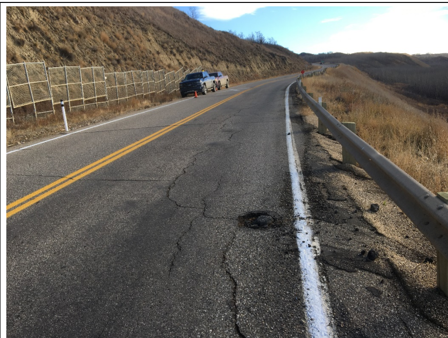
Photo 9. Looking southeast along the shoulder of the SBL at km 59.255. There is an old stone column protruding through the ACP and the dip in the guardrail is at 150 mm at SI10-15.
