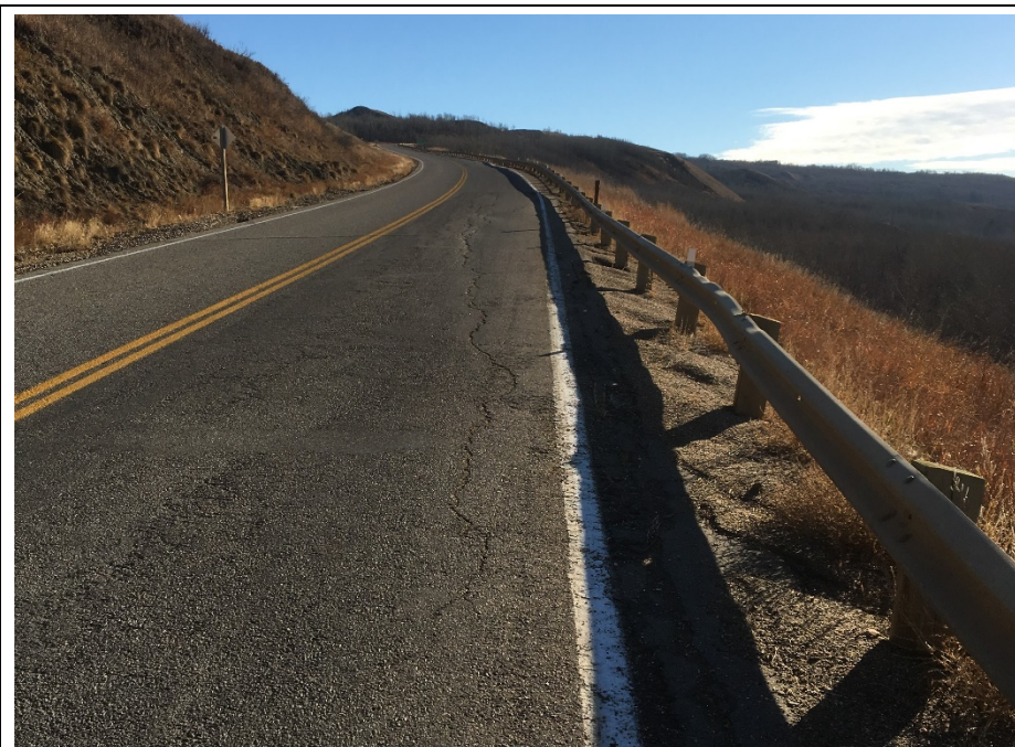
Photo 1. Looking southeast from the shoulder of the SBL at km 59.135 towards the cracks and dip in the pavement at SI10-12. The dip in the guardrail is at 210 mm and the cracks in the ACP or open from 50 to 60 mm with drops along the edges of cracks up to 70 mm.
