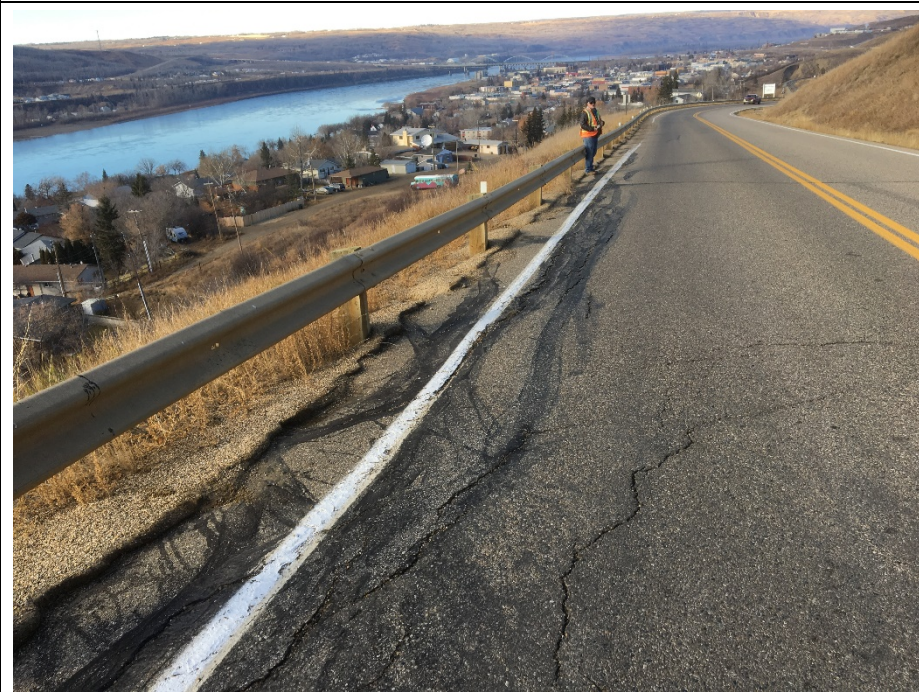
Photo 10. Looking south from the SBL at km 59.265 at the cracks in the shoulder of the ACP are open to 30 mm.
