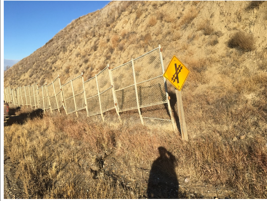
Photo 8. Looking northeast from NBL shoulder at km 59.23 towards the south end of the chain link fence. The six southernmost fence panels are more tilted/jacked than in May 2018.
