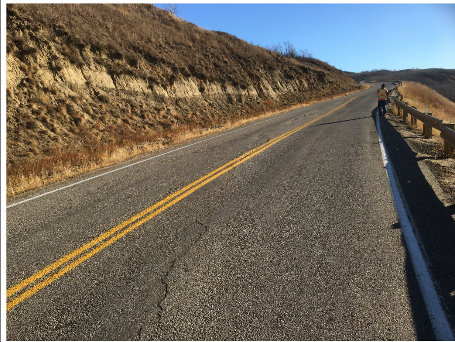
Photo 7. Looking southeast from km 59.198 in the SBL at the large dip. There are more cracks along the edge of the dip than in May 2018 and the overall drop along the dip at 400 mm.
