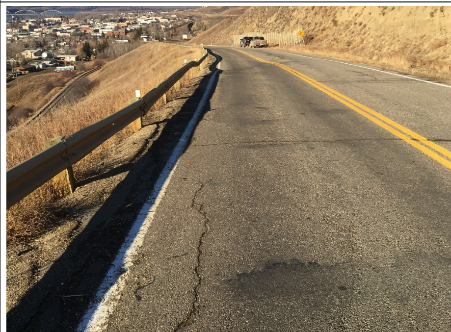
Photo 2. Looking northwest from km 59.145 along the outer edge of the SBL. The cracks along the white line in the SBL are open from 30 mm to 60 mm.
