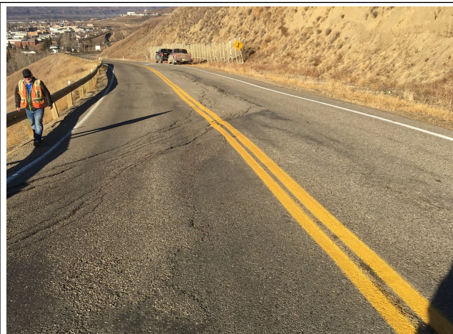
Photo 3. Looking north from km 59.15 at the south end of the Fence Slide repair. The dip and grown and extends 1.5 m into the NBL. Cracks in the SBL shoulder of the are now open to 60 mm.
