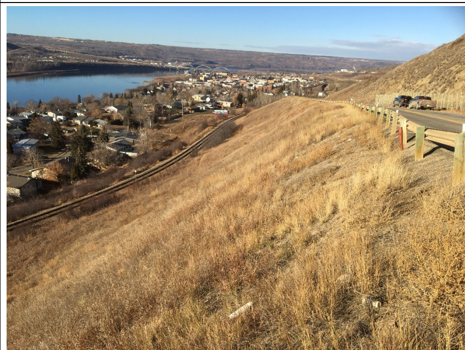
Photo 4. Looking north from km 59.155 along sideslope towards SI10-13. The dip in the guardrail is at 700 mm near the lowest point in the dip in the SBL. The shallow slump below SI10-13 is more apparent than in May 2018.
