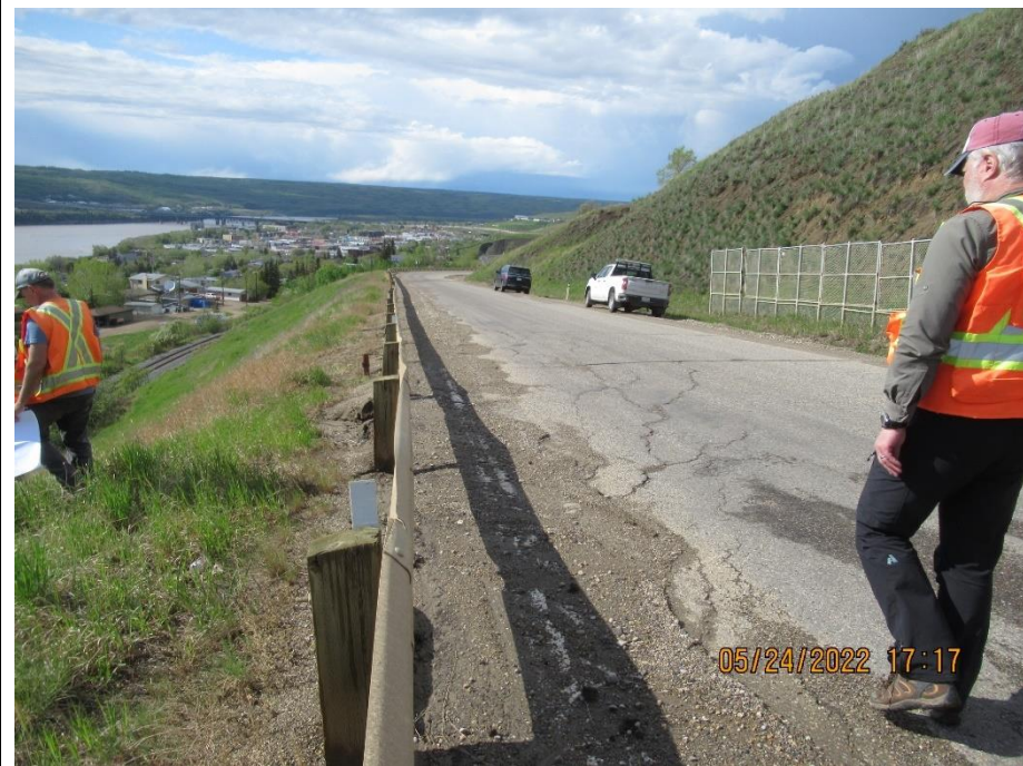
Photo 5. Looking northwest from km 59.21 at the west sideslope below S110-15. Minor rill erosion otherwise no major change from 2021.
