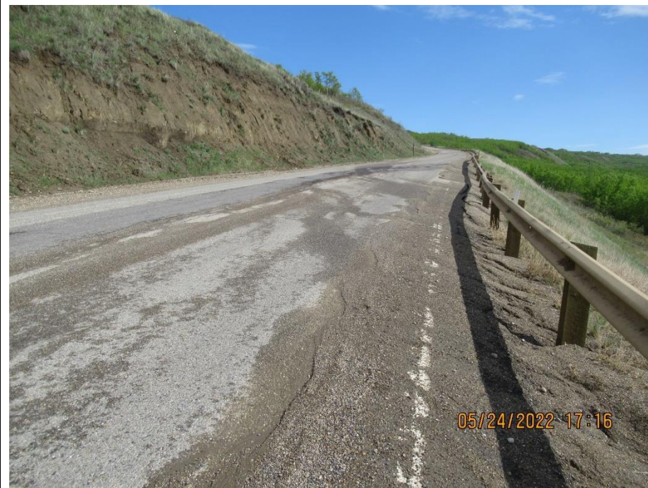
Photo 3. Looking south from the north end of the Fence Slide repair at km 59.18. Depression extends into the NBL and appears more pronounced. Differential pavement edge has been milled.
