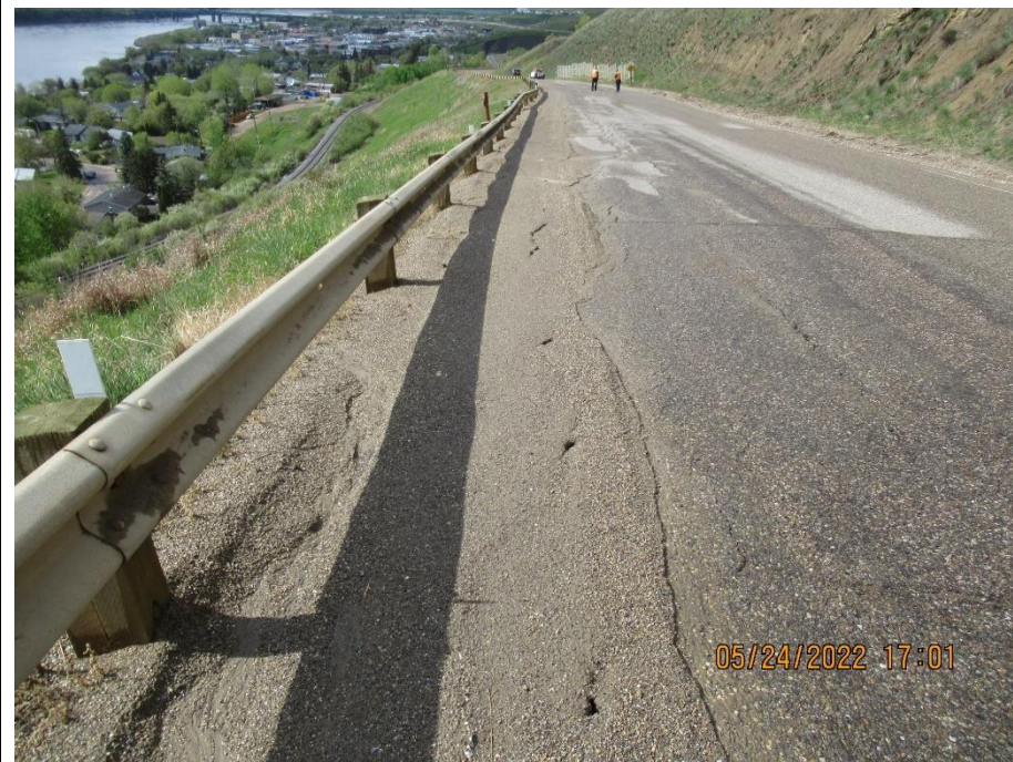
Photo 1. Looking northwest from km 59.07 at the cracking and pavement distress along the downhill side of the road near S110-12. No significant visual change in the pavement from the 2021 condition.
