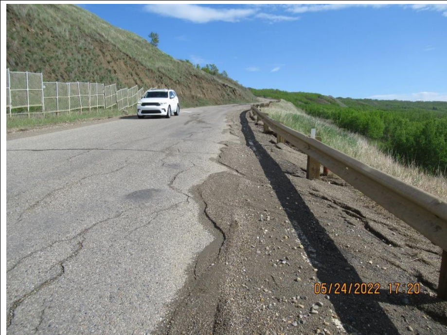
Photo 6. Looking southeast from km 59.25 along the SBL. Cracking and dip along the shoulder appeared slightly worse relative to the 2021 condition. Sand buildup along the shoulder.
