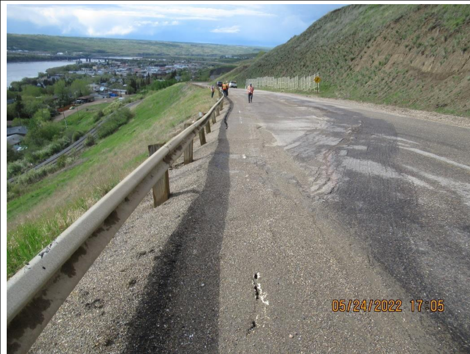
Photo 2. Looking north from the south end of the Fence Slide repair at km 59.14. Slide damage extends into the NBL. The sharp pavement edge due to the dip has been milled.
