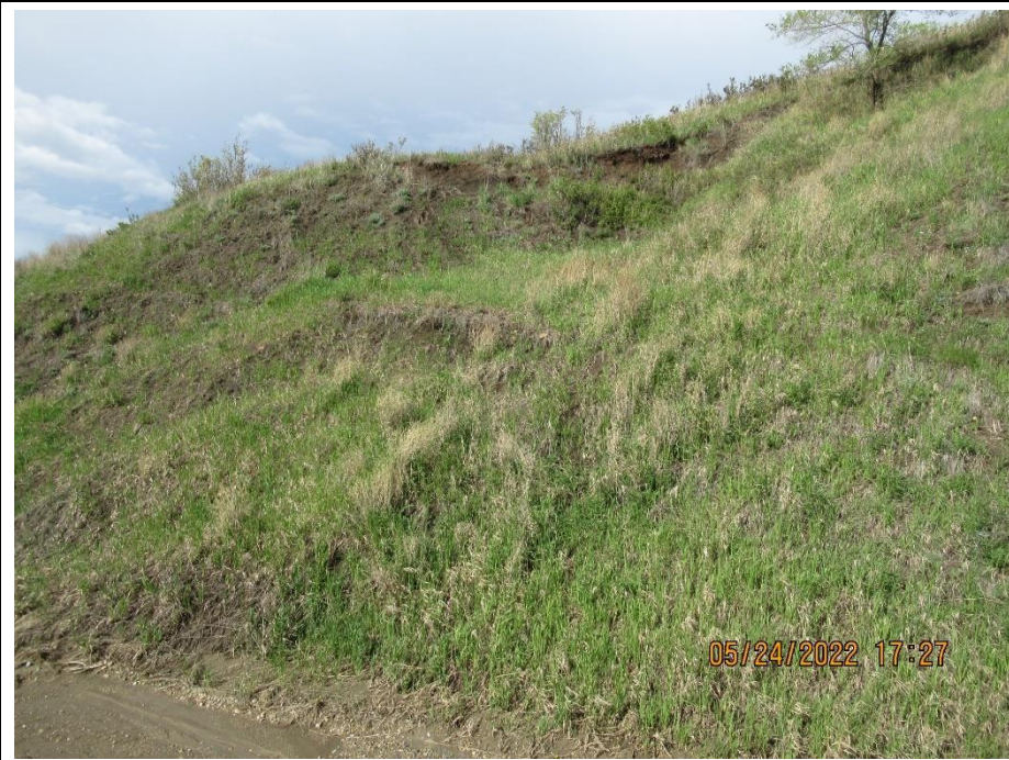
Photo 7. View of old slump in the backslope near km 59.3. Fresh soil visible in the upper scarp since the 2021 condition.
