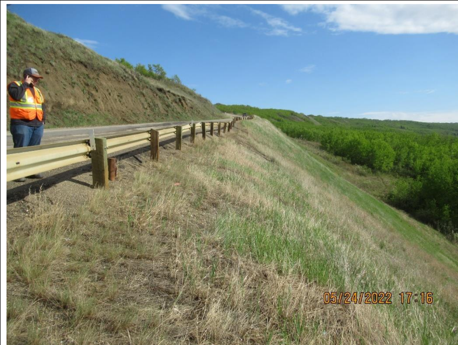
Photo 4. Looking south from the west sideslope of Hwy 744:04 from km 59.18. The bow and vertical deflection in the guardrail are visible.
