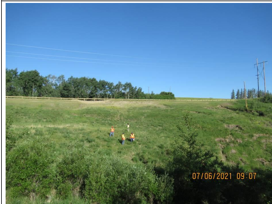
Photo 65-4. View towards recently active slide area above culvert outlet that has retrogressed to the pavement on the east embankment (44+975). Note visible toe roll.
