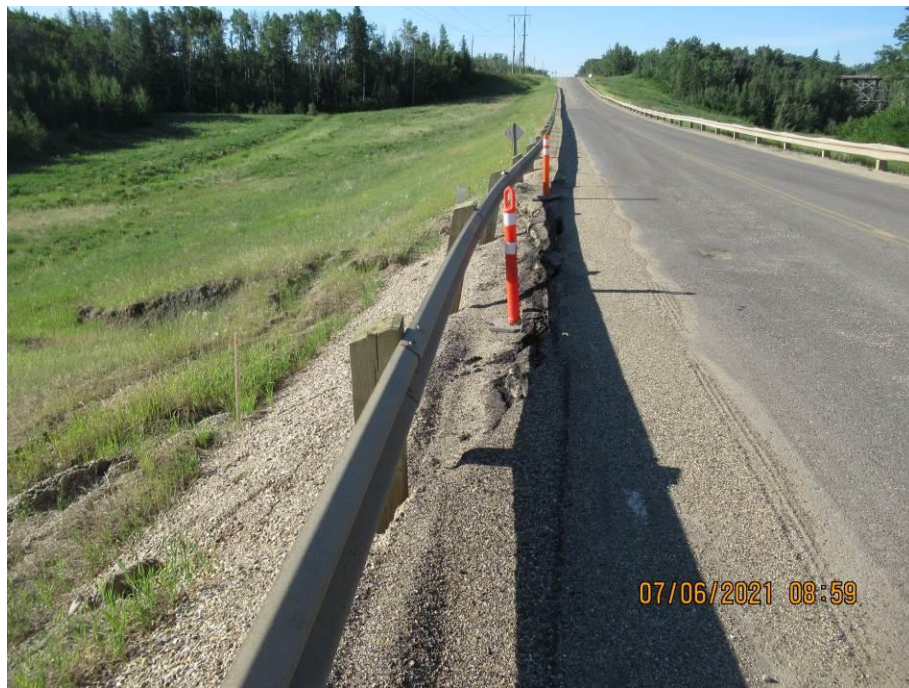
Photo 65-2. Looking south towards the scarp retrogressing into the road pavement (45+00). Slide scarp was first noted in 2016 and is now approximately 1.7 m high at the pavement and retrogressed 0.7 m from the guardrail into the pavement with three posts hanging freely.
