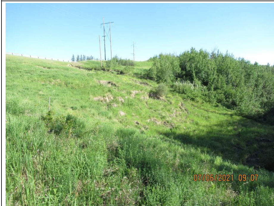
Photo 65-6. Looking northwest towards multiple active, shallow slides coalescing above the culvert outlet. Area has ongoing movement, especially near the toe where there is active bank erosion (44+975) but no significant retrogression of the headscarp towards the highway.
