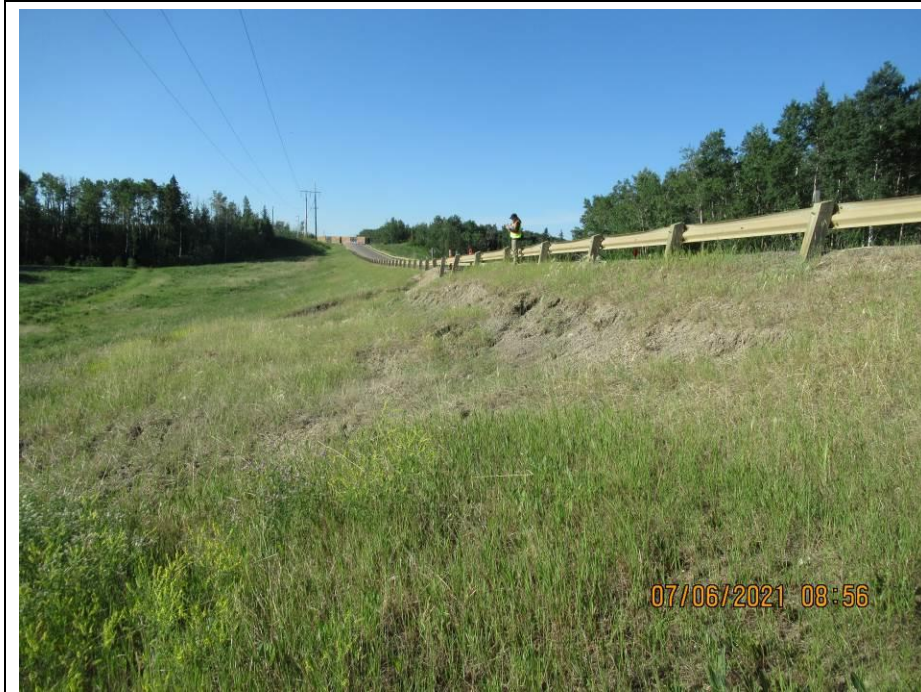
Photo 65-3. Looking south along the east side of the highway embankment towards an active main slide scarp (45+015) first identified in 2016. Increased dropdown since 2020.
