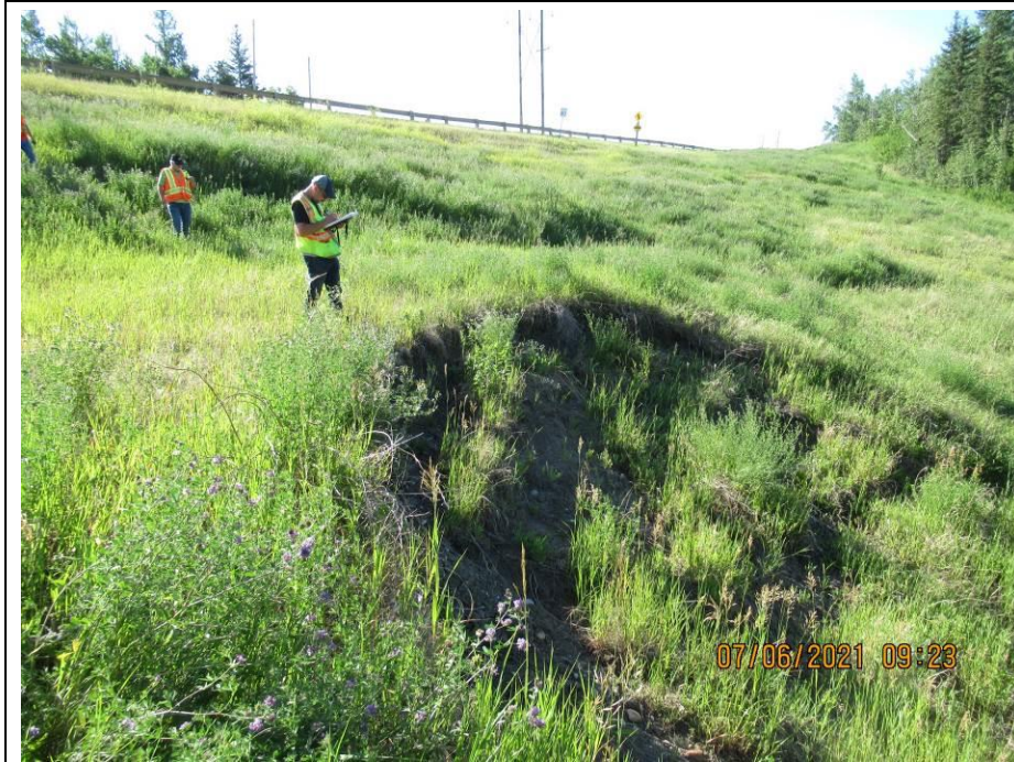
Photo 65-9. Looking southeast towards a recently active shallow earth slide above the culvert inlet (44+830). Slide is offset approximately 27 m west of the highway edge.
