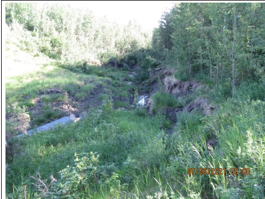
Photo 65-5. Active bank sliding and erosion area around the culvert outlet (44+975). Worse since 2020.
