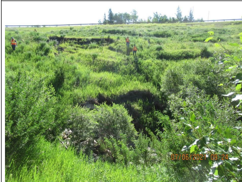
Photo 65-10. Looking east towards the road embankment with active shallow slide activity immediately above the culvert inlet (near inspectors) and near the headwall.
