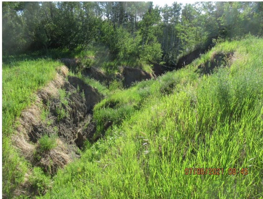
Photo 65-1. Erosion gully at the culvert outlet (45+200) had increased sliding along the flanks.
