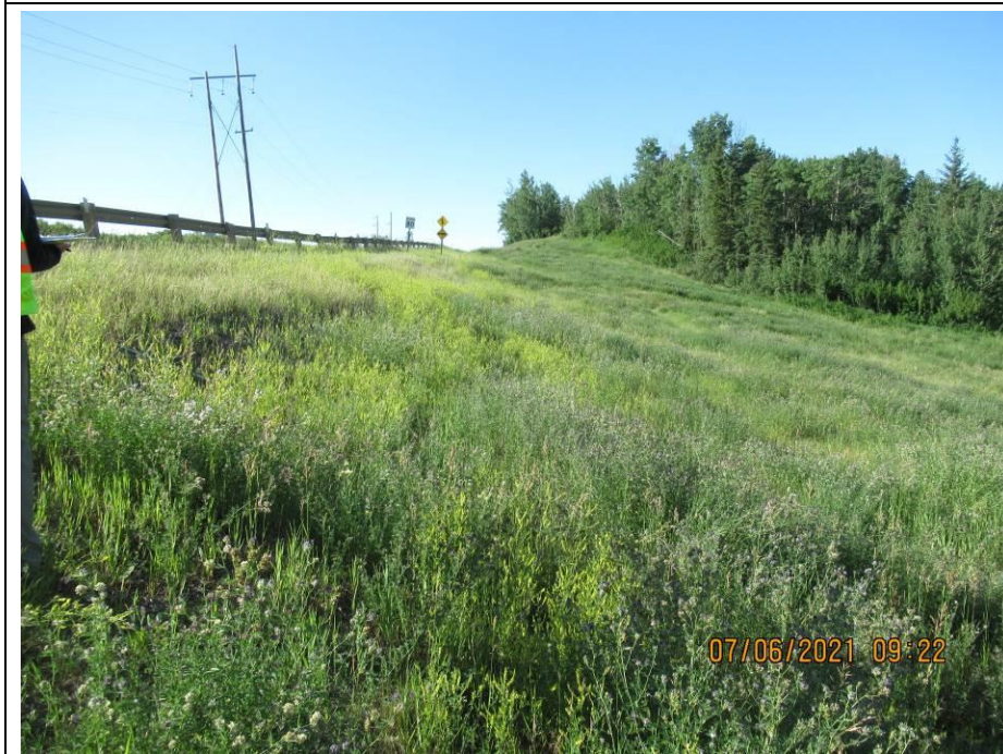
Photo 65-8. Looking south along the upper slope of the west side of the road embankment. No major changes noted since previous inspection.
