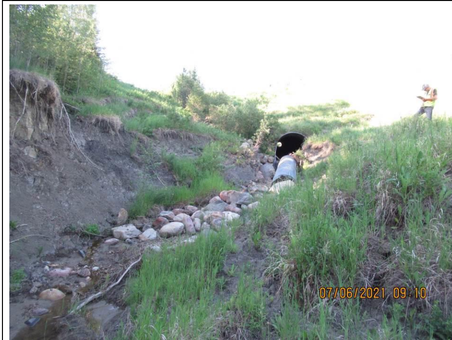
Photo 65-7. Active sliding and erosion area around the headwall of the culvert outlet (45+000). Movement has pinched the outlet area of an armoured swale to the south of the outlet. Note old washed through culvert section causing debris jam.
