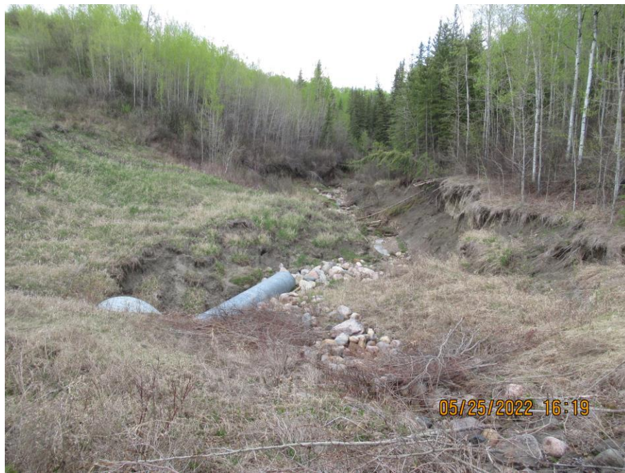
Photo 65-4. Active bank sliding and erosion area around the culvert outlet (44+975). Worse since 2021.
