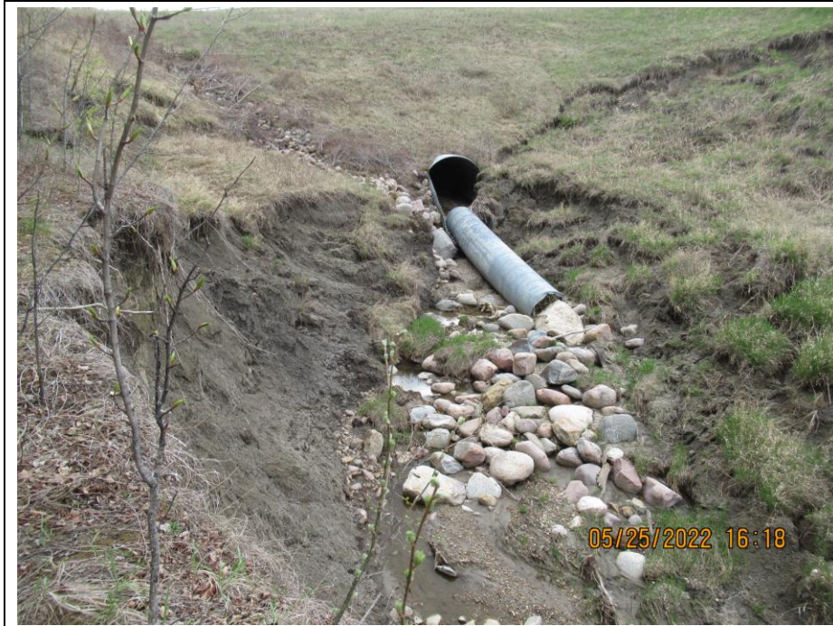
Photo 65-6. Active sliding and erosion area around the headwall of the culvert outlet (45+000). Movement has pinched the outlet area of an armoured swale to the south of the outlet. Note old washed through culvert section causing debris jam. There was increased erosion around the outlet and creek banks.
