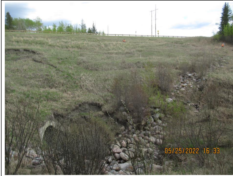
Photo 65-9. Looking east towards the west road embankment with active shallow slide activity immediately above the culvert inlet (near inspectors) and near the headwall. Note visible toe roll of slide which has begun to encroach into the armored drainage swale on the right side of the photo.
