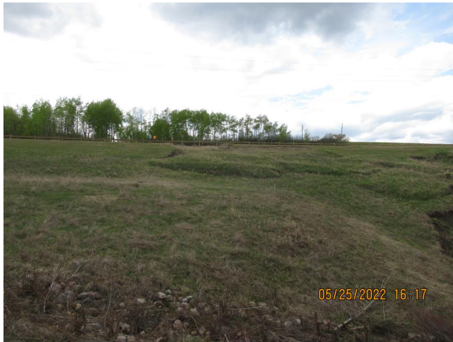
Photo 65-3. View towards recently active slide area above culvert outlet that has retrogressed to the pavement on the east embankment (44+975). Note visible toe roll.
