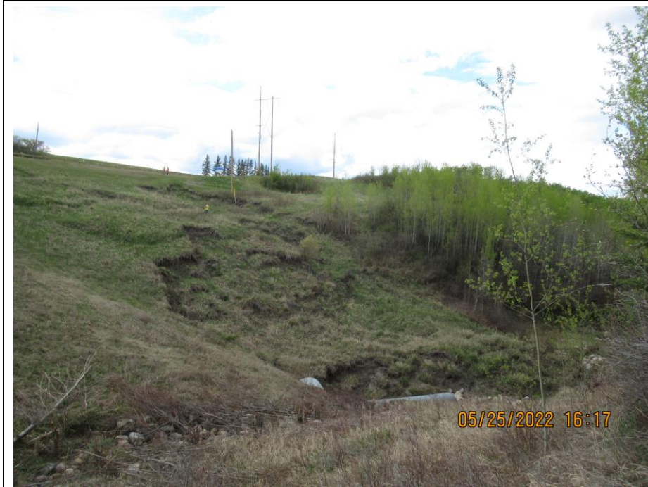
Photo 65-5. Looking northwest towards multiple active, shallow slides coalescing above the culvert outlet. Area has ongoing movement, especially near the toe where there is active bank erosion (44+975) but no significant retrogression of the headscarp towards the highway.
