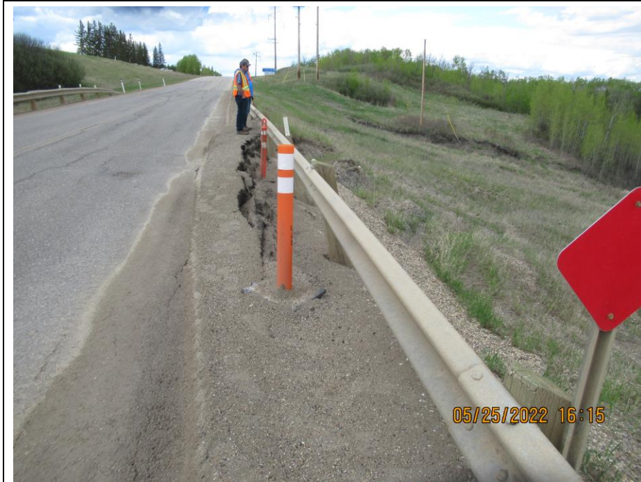
Photo 65-1. Looking north towards the scarp retrogressing into the road pavement (45+00). Slide scarp was first noted in 2016 and is now approximately 1.7 m high at the pavement and retrogressed 0.8 m from the guardrail into the pavement with three posts hanging freely.
