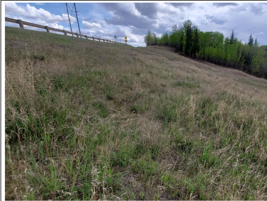
Photo 65-7. Looking south along the upper slope of the west side of the road embankment. No major changes noted at the head of the slides near the highway.
