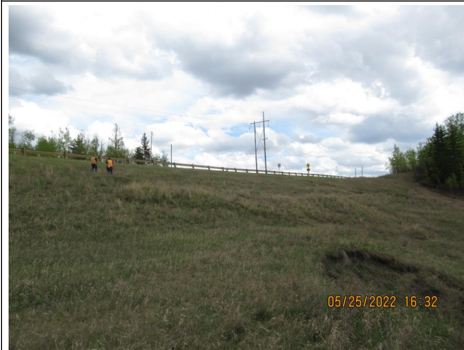
Photo 65-8. Looking southeast towards a recently active shallow earth slide above the culvert inlet (44+830). Slide is offset approximately 27 m west of the highway edge. Minor retrogression has occurred at the main scarp (lower right of photo).
