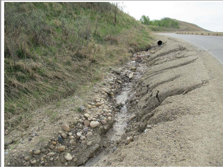
Photo 8. Looking south from the NBL shoulder of Hwy 744:04 at km 58.38. The scour in the ditch bottom is worse than in 2017 and is now at 1.6 m from the white line.
