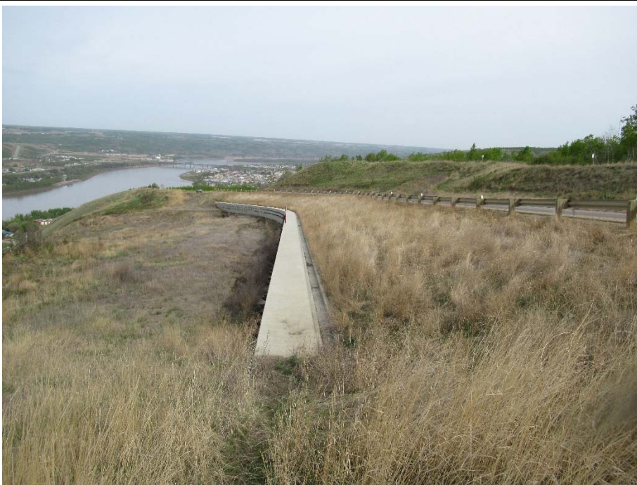
Photo 2. Looking northwest from south end of the Sunshine pile wall at km 58.200. Vegetation directly above the pile wall is still thick.
