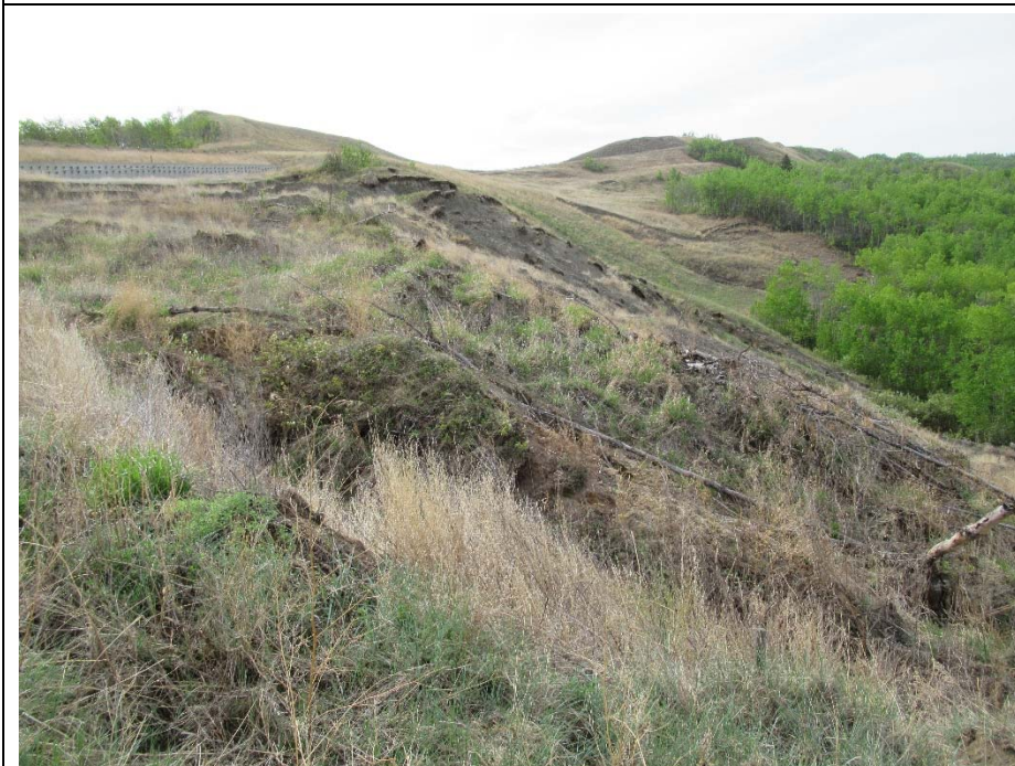
Photo 6. Looking southeast from 30 m south of the pile wall along the backscarp at the slide bowl.
