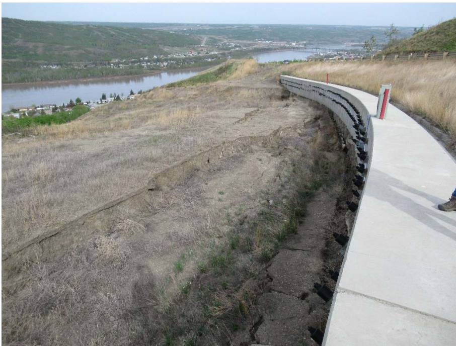
Photo 3. Looking northwest from below the pile wall at km 58.26. Slide in bench below wall is very active. Some piles are exposed to 1.5 m. About 20 anchor grease caps have fallen off.
