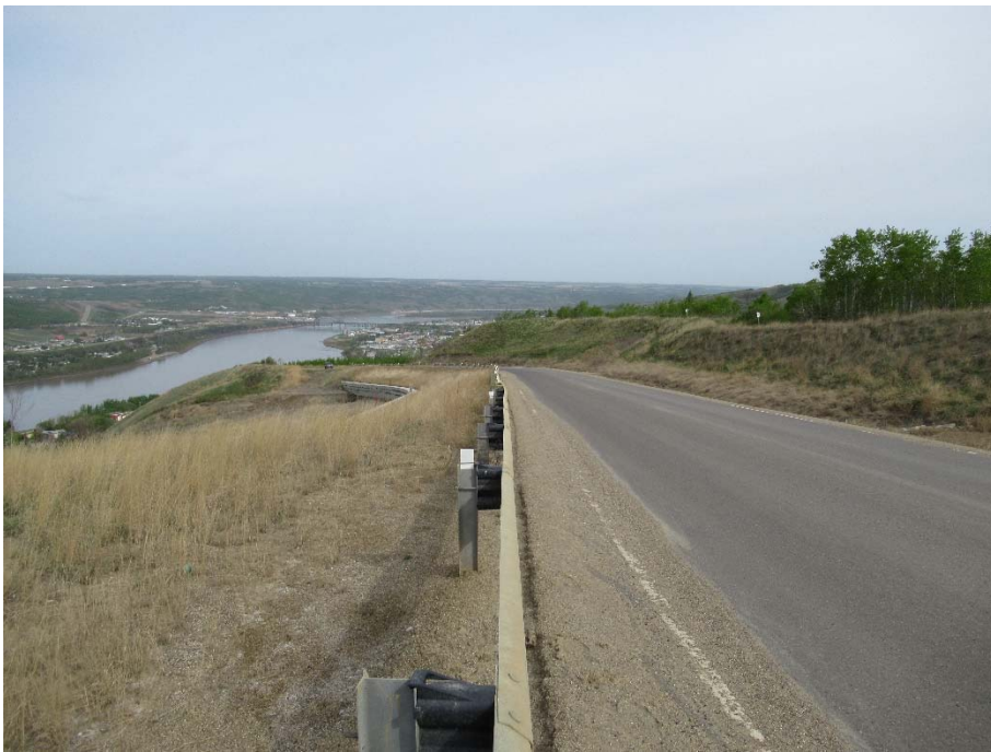
Photo 1. Looking northwest from the guardrail of the SBL of Hwy 744:04 at km 58.170 at the south end of the Sunshine pile wall. No signs of any cracks in the ACP.
