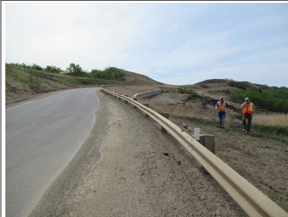
Photo 7. Looking southeast from the centerline of Hwy 744:04 at km 58.34 at the reinstated embankment.
