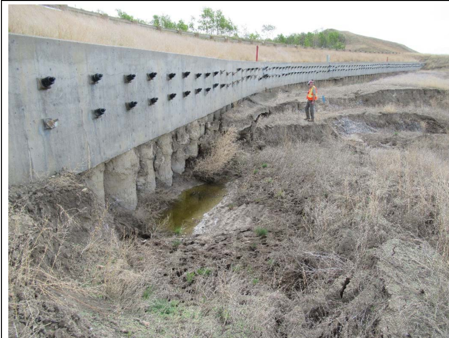
Photo 5. Looking southeast along the pile wall at km 58.33. The cracking in the passive soil bench below the pile wall has grown since 2017. Some piles are exposed to 1.5 m. About 20 anchor grease caps have fallen off. Water is ponding in graben area along the wall.
