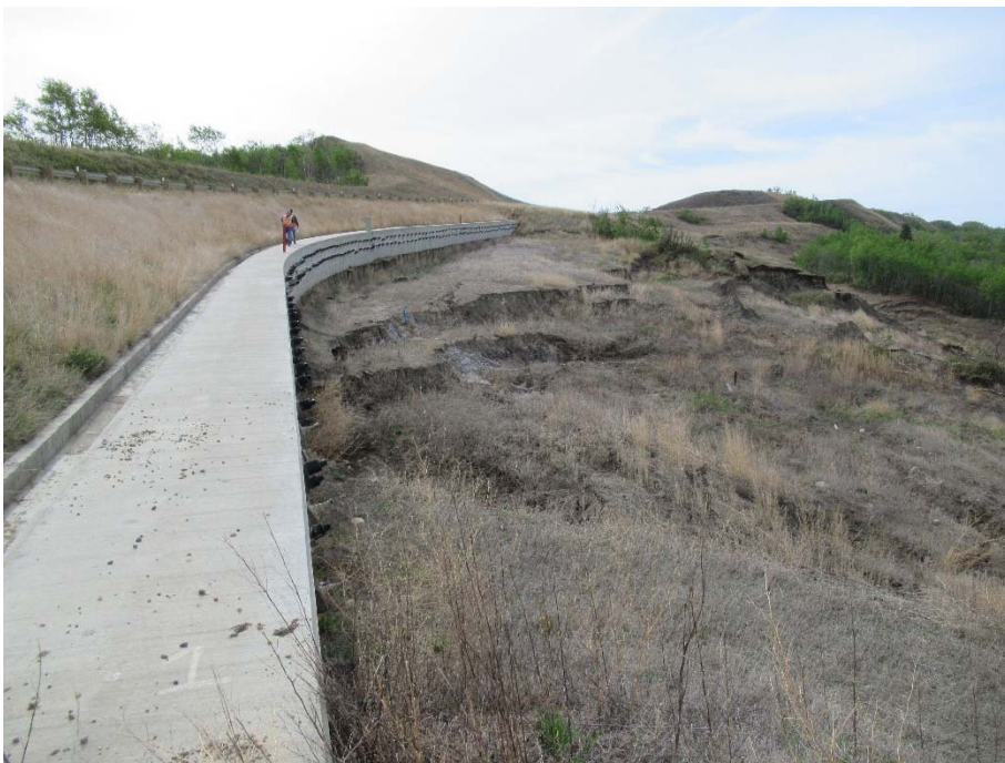
Photo 4. Looking southeast along the pile wall at km 58.33. The cracking in the passive soil bench below the pile wall has grown since 2017.
