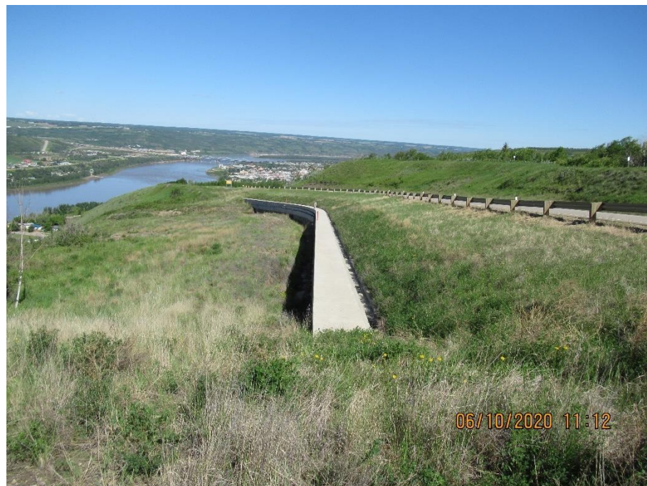
Photo 2. Looking northwest from south end of the Sunshine pile wall at km 58.200. Vegetation directly above the wall is well established. Some thicker vegetation growth noted directly below the wall relative to the previous inspection.
