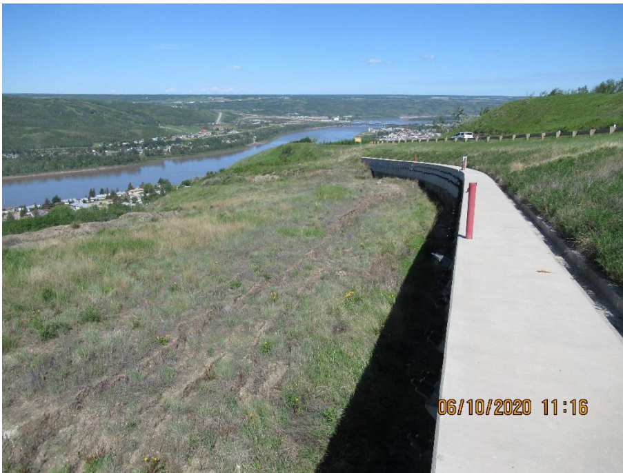
Photo 3. Looking northwest from below the pile wall at km 58.26. Slide in bench below wall is very active. Some piles are exposed up to 1.6 m in height (no change from 2019).
