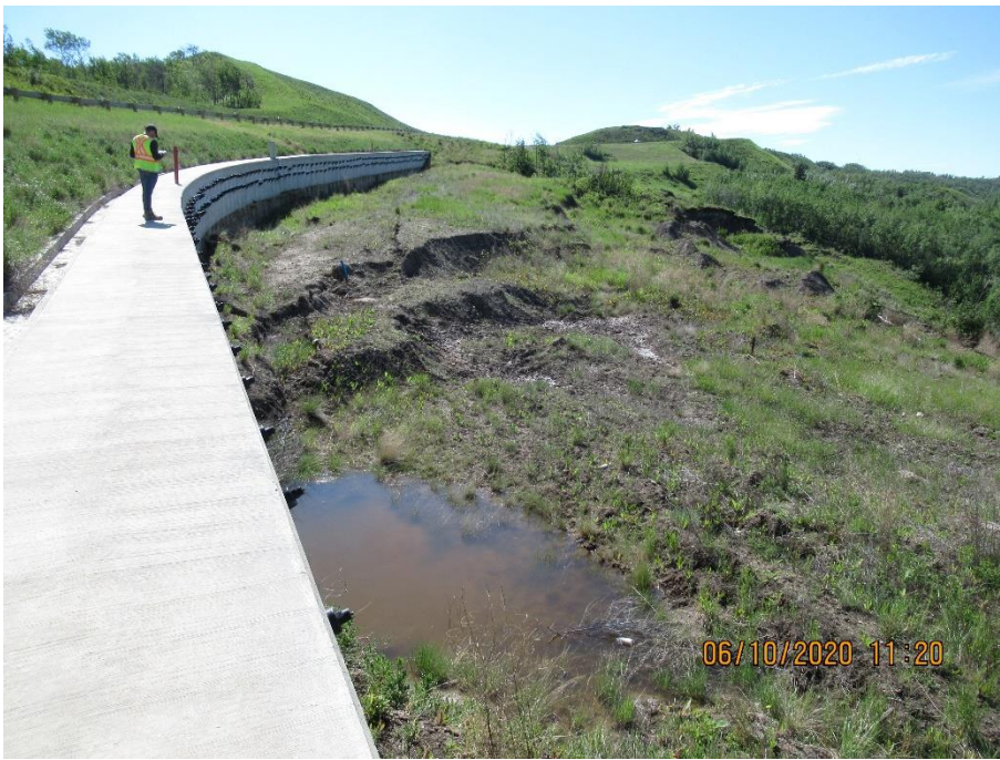
Photo 4. Looking southeast along the pile wall at km 58.33. The cracking/ signs of visible movement in the passive soil bench below the pile wall has not changed significantly. Sliding in the lower slope appears active. Water had increased ponding in graben area along the wall relative to the 2019 inspection.
