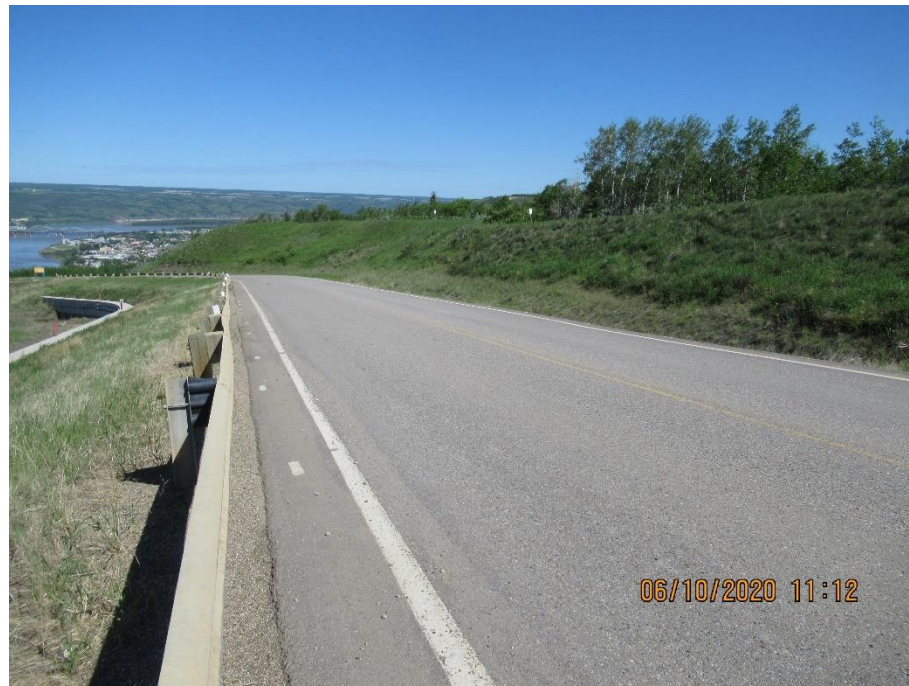
Photo 1. Looking northwest from the guardrail of the SBL of Hwy 744:04 at km 58.2 at the south end of the Sunshine pile wall. No signs of any damage in the ACP.
