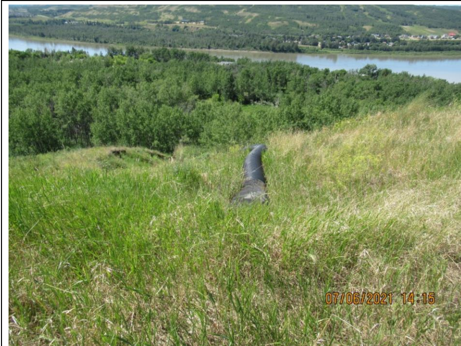
Photo 3. Looking west at km 58.9 at the corrugated plastic down-drain at connection to the centerline culvert. No change from 2020.
