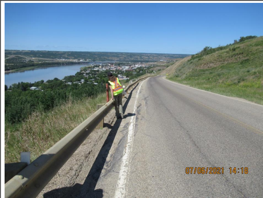
Photo 6. Looking northwest from km 58.95. Dip in the SBL has not visibly changed. Crack apertures are open from 50 mm to 170 mm in width.
