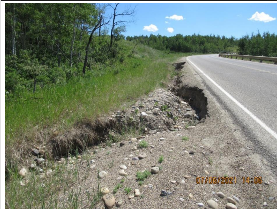
Photo 1. Looking south at the ditch erosion upslope from the Judah Truck Inlet towards the Sunshine Slide site. Erosion is worse and cutting towards the road and has begun to undermine the ACP shoulder in select areas creating a hazard for vehicles.
