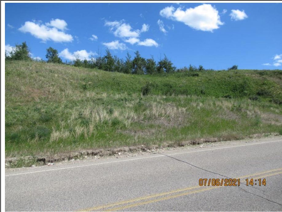
Photo 5. Looking east from km 58.9 at vegetated backslope slide scarp No change from 2020.
