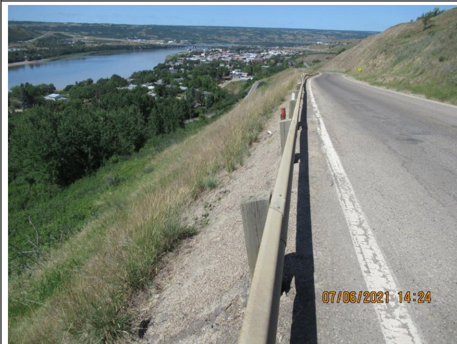
Photo 8. Looking northwest from km 59.01 at cracking within the shoulder and southbound lane near SI10-11. Stone columns showing through the ACP in the SBL. No major change since 2020.
