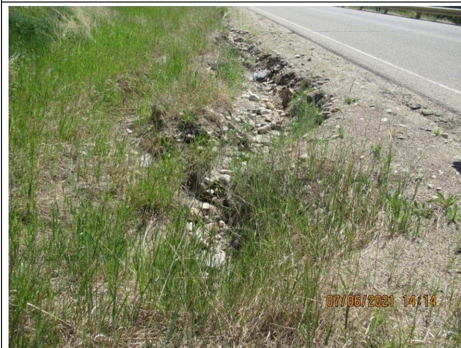
Photo 2. Looking southeast at the ditch erosion upslope from the Judah Truck Inlet. No significant change from 2020 condition.
