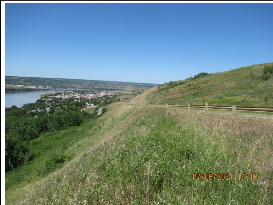
Photo 7. Looking northwest from km 58.93 at slope below the highway near SI10-10. No change from 2020.
