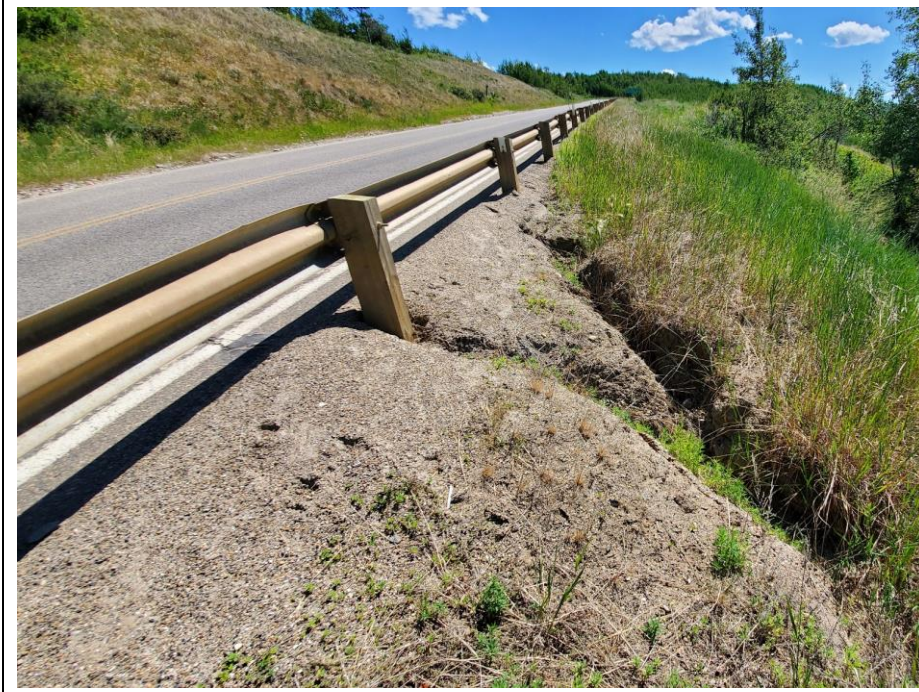
Photo 9. Looking south at erosion rills on the west side of the highway near km 58.85. Slightly worse from 2020 condition.
