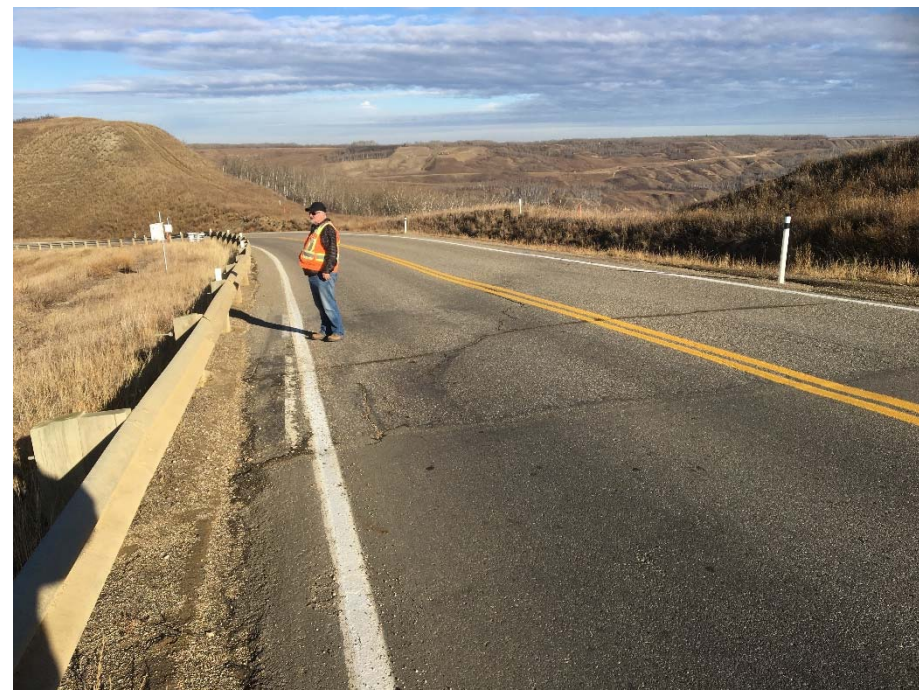
Photo 1. Looking northeast along the SBL guardrail of Hwy 744:04 from km 57.8 at the dip in the SBL immediately north of the 2015 realignment. No significant change since May 2018.
