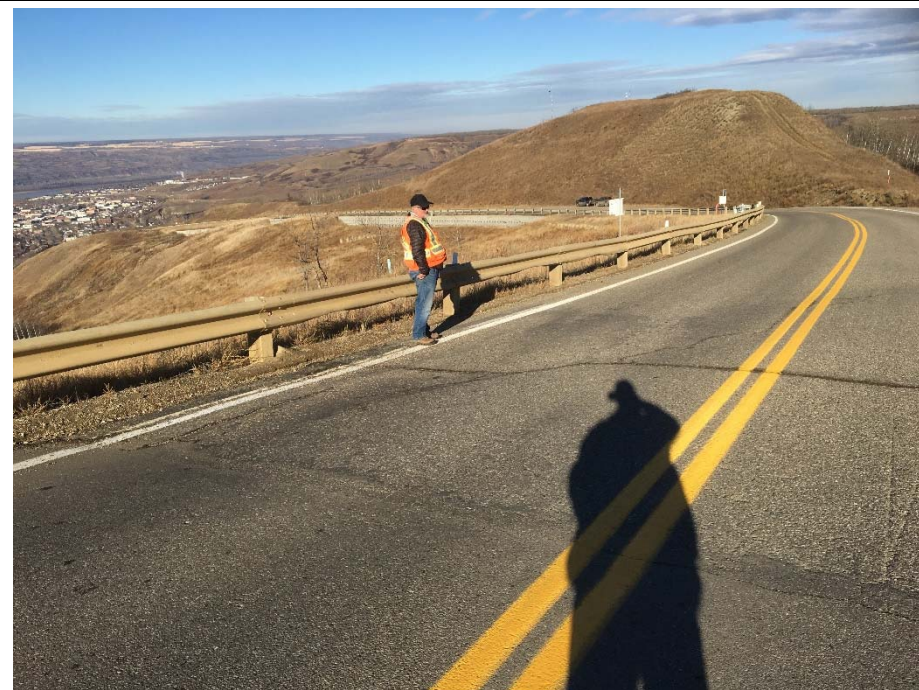
Photo 2. Looking north from the centerline of Hwy 744:04 from km 57.81 at the dip in the SBL to the north of the 2015 realignment.
