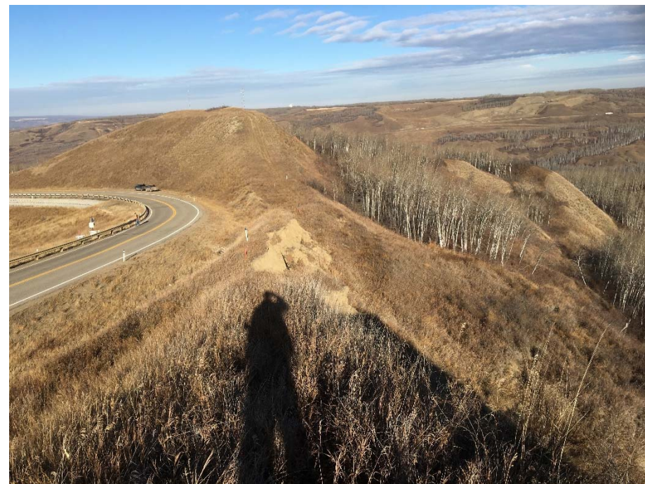
Photo 3. Looking northeast from the top of scarp of the slide on the Heart River side along the former ATCO pipeline right-of-way. There has been some retrogression of the backscarp and the graben at the center of the slide has dropped since May 2018.
