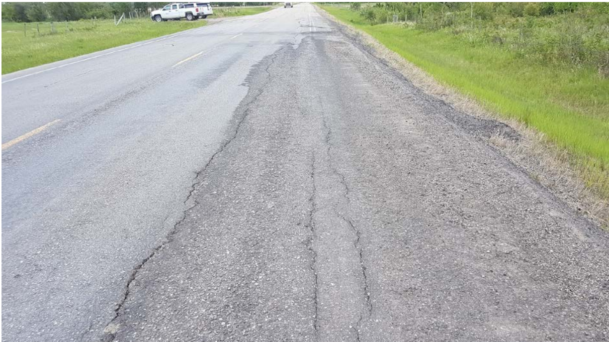
Photo 4: Looking south at previous location of significant cracking in SBL and shoulder.
