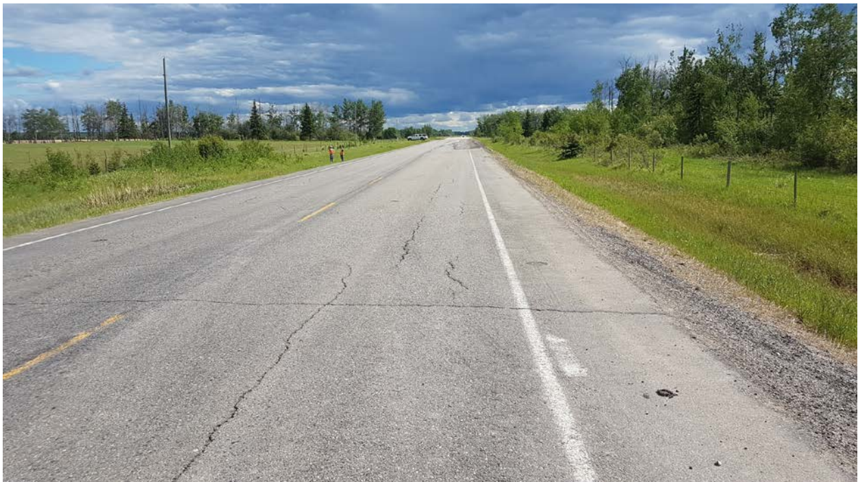
Photo 6 – Looking south at typical SBL cracking near residence approach.
