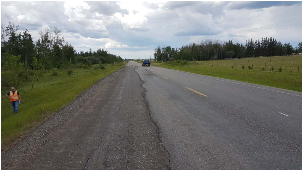
Photo 2 – Looking north at south end of main crack.
