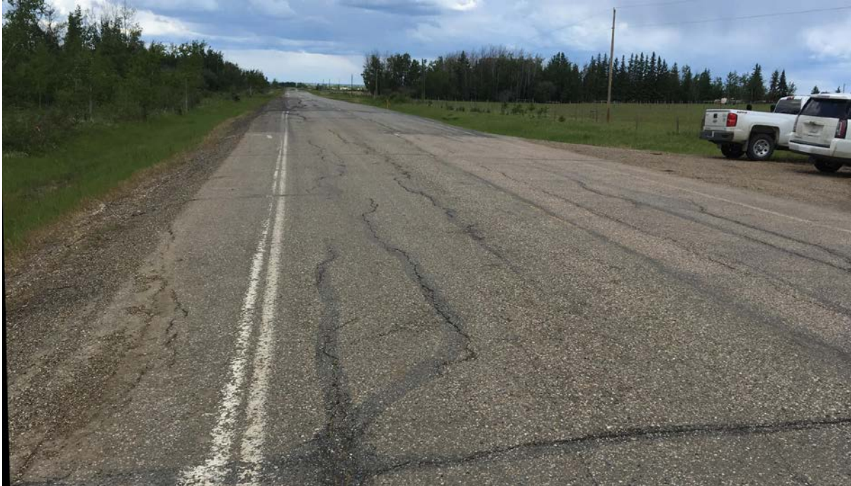
Photo 1 – Looking north along (west) shoulder of SBL just north of 1800 mm dia. culvert where there is a slight bulge along the embankment.
