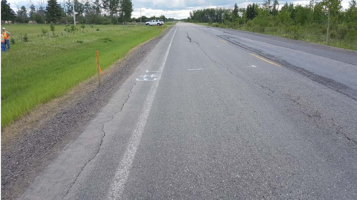
Photo 3: Looking south at new cracking in outer wheel path of NBL and shoulder.
