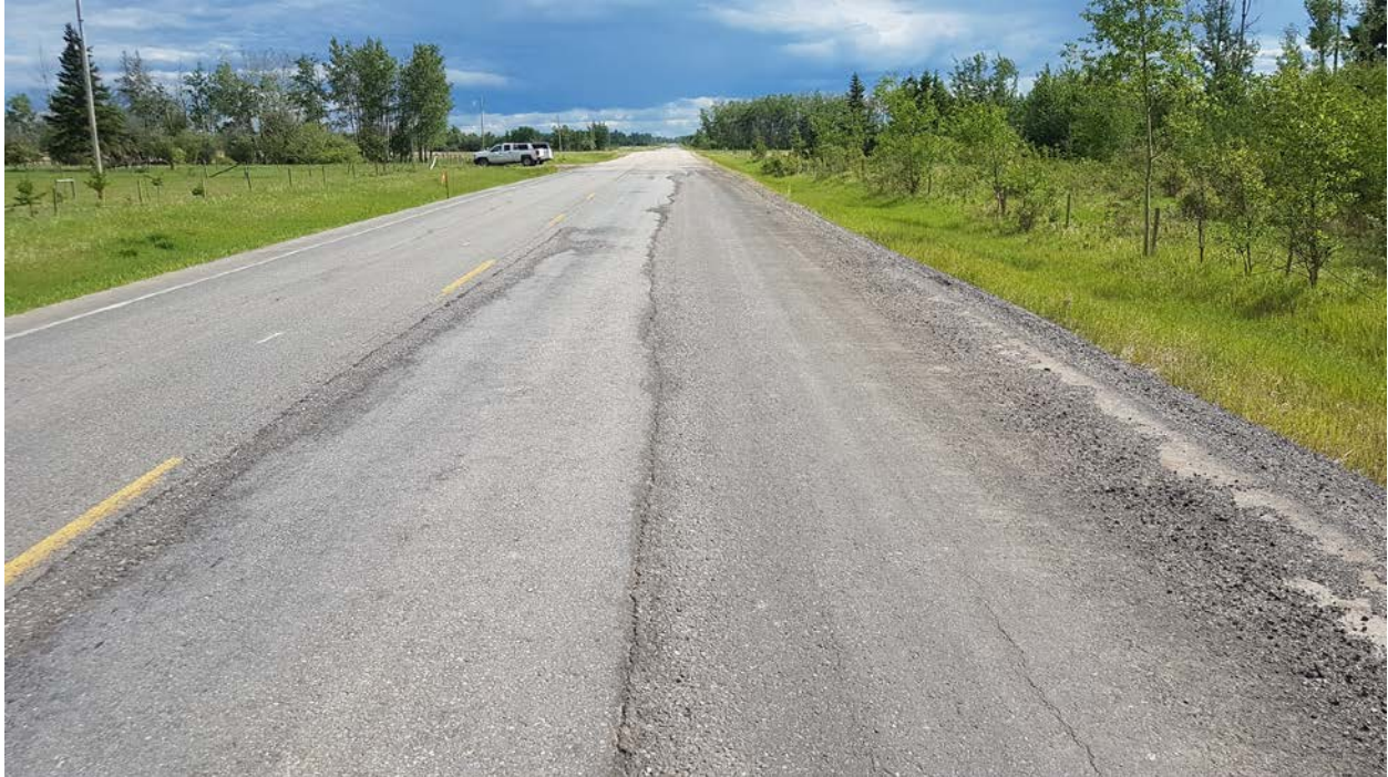
Photo 5: Looking south at main crack and previous void in the shoulder of the SBL.
