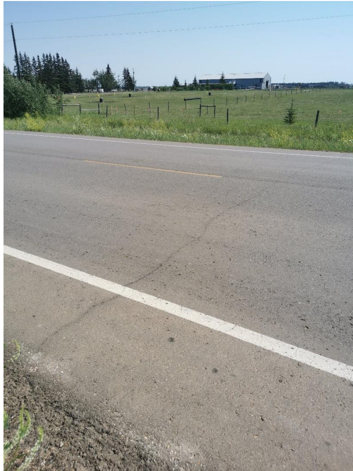
Photo 4: Looking northeast at transverse cracking on the pavement at the middle portion of the site.
