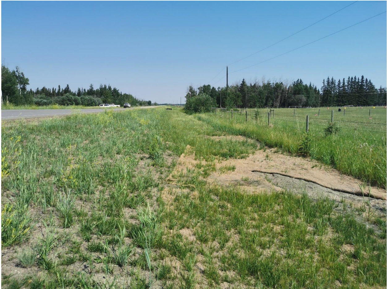
Photo 5: Looking north along east ditch where erosion control matting is bunched up.
