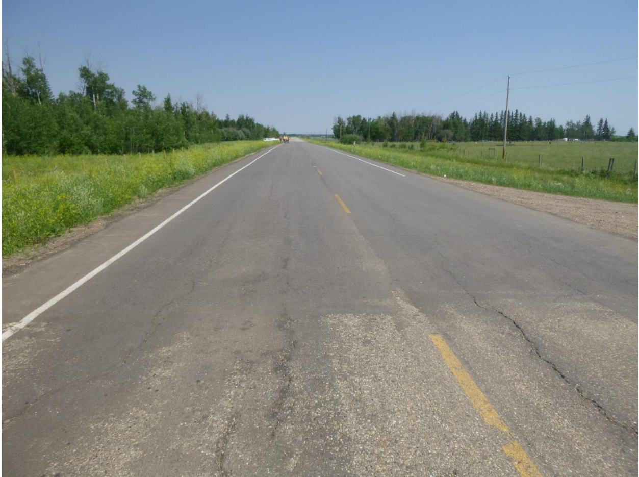
Photo 3: Looking north from the south end of the site near the 1800 mm diameter culvert.
