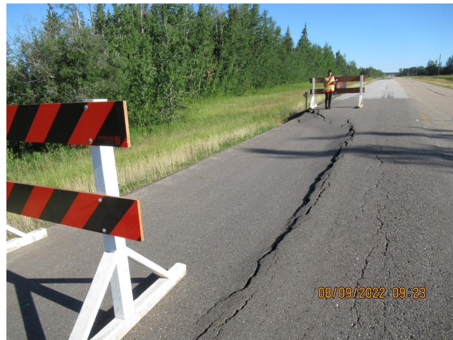
Photo 1. Looking north at scarp affecting the southbound lane.
