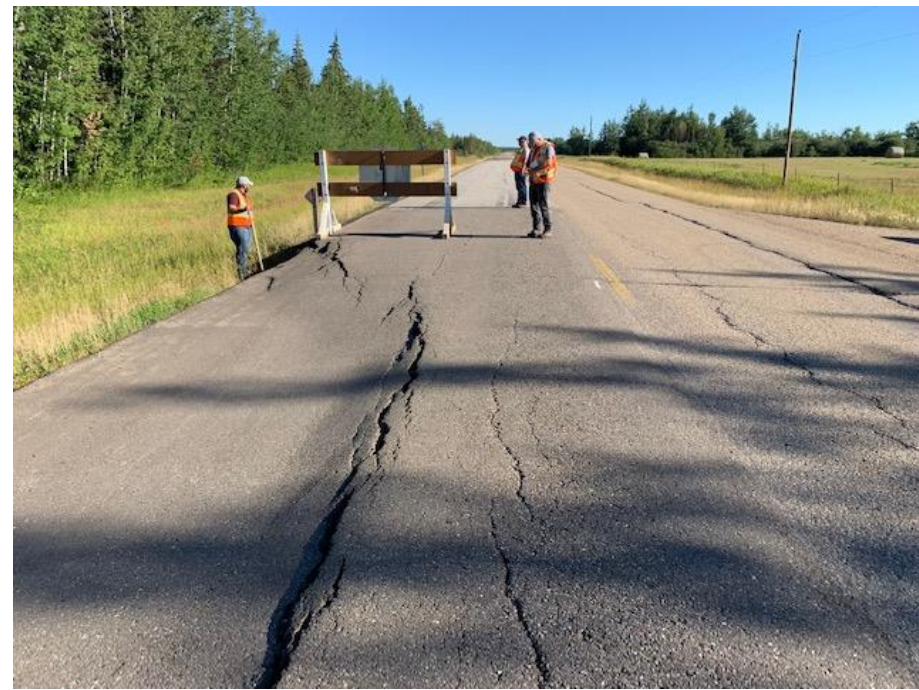
Photo 2. Looking north standing near middle of scarp crack.
