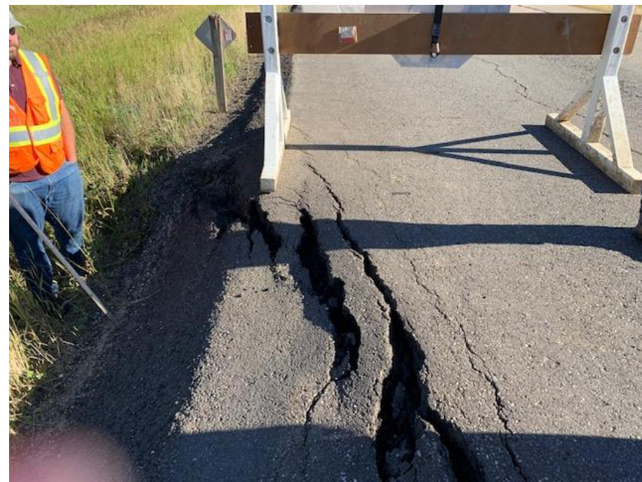
Photo 5. Looking at cracks on shoulder of highway open up to 100 mm wide.
