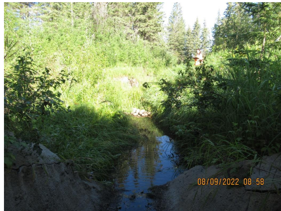
Photo 9. Looking west from culvert outlet at creek and creek erosion.
