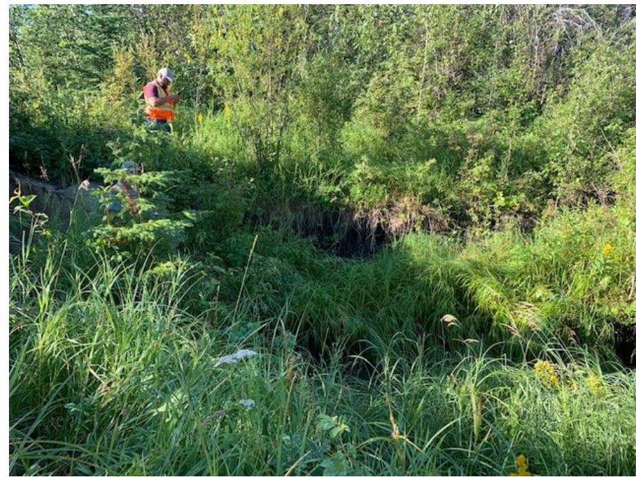
Photo 8. Looking south at where bank erosion has taken place.
