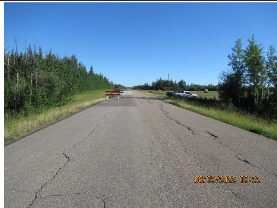
Photo 4. Looking north at lane patching and barricades on either side of scarp.
