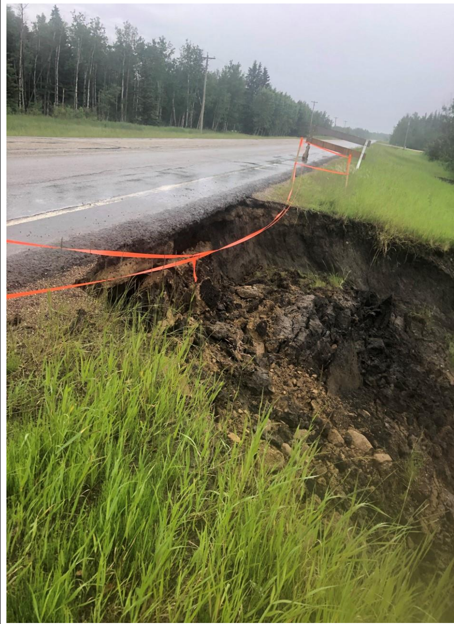
Photo 11. Looking south at landslide scarp that has retrogressed further cutting into pavement taken after call out inspection on July 2, 2020.
