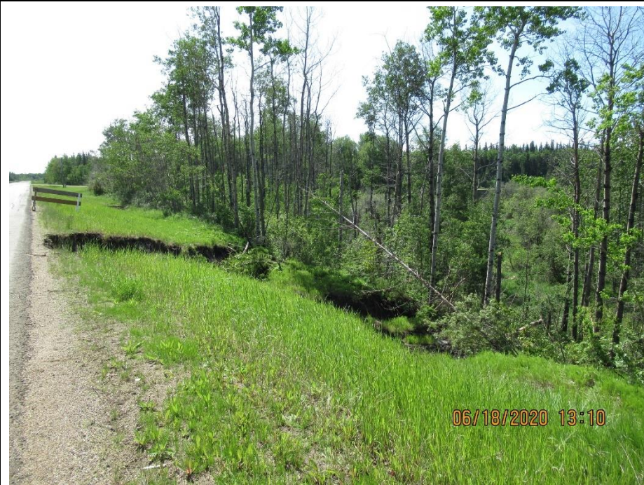
Photo 9. Looking south at landslide scarp retrogressing close to the highway pavement.
