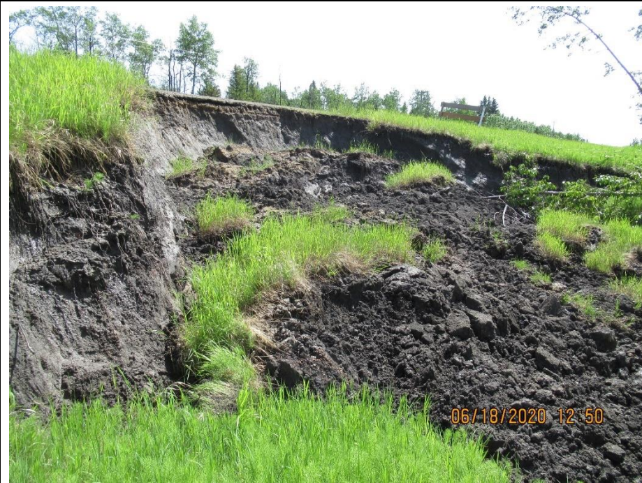
Photo 5. Looking southeast towards backscarp and slabs of soil.
