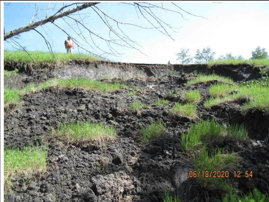
Photo 6. Looking east towards highway and landslide backscarp.
