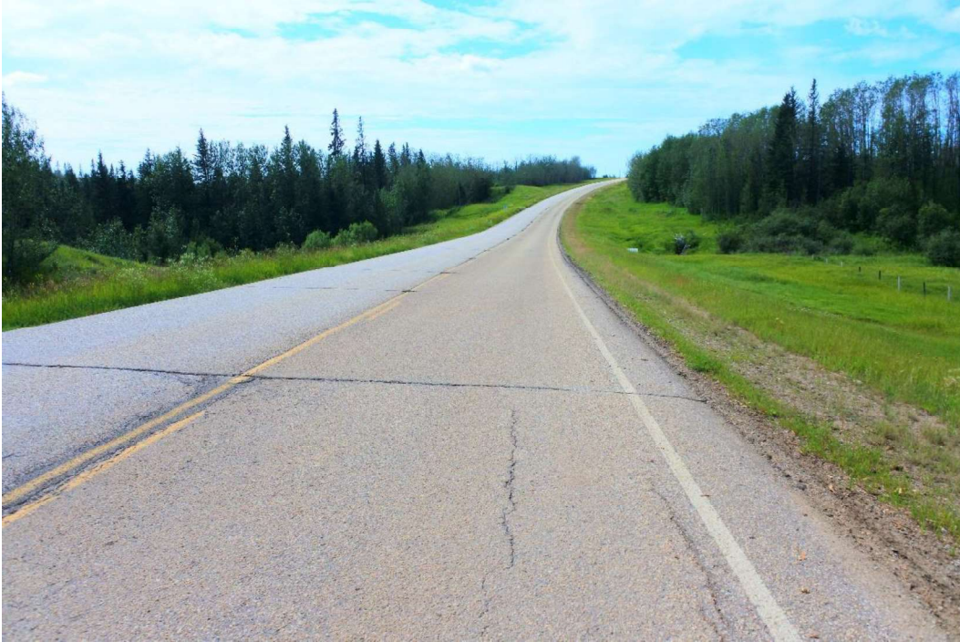
Photo 5 – Looking south at potential extension of slide-related cracks.
