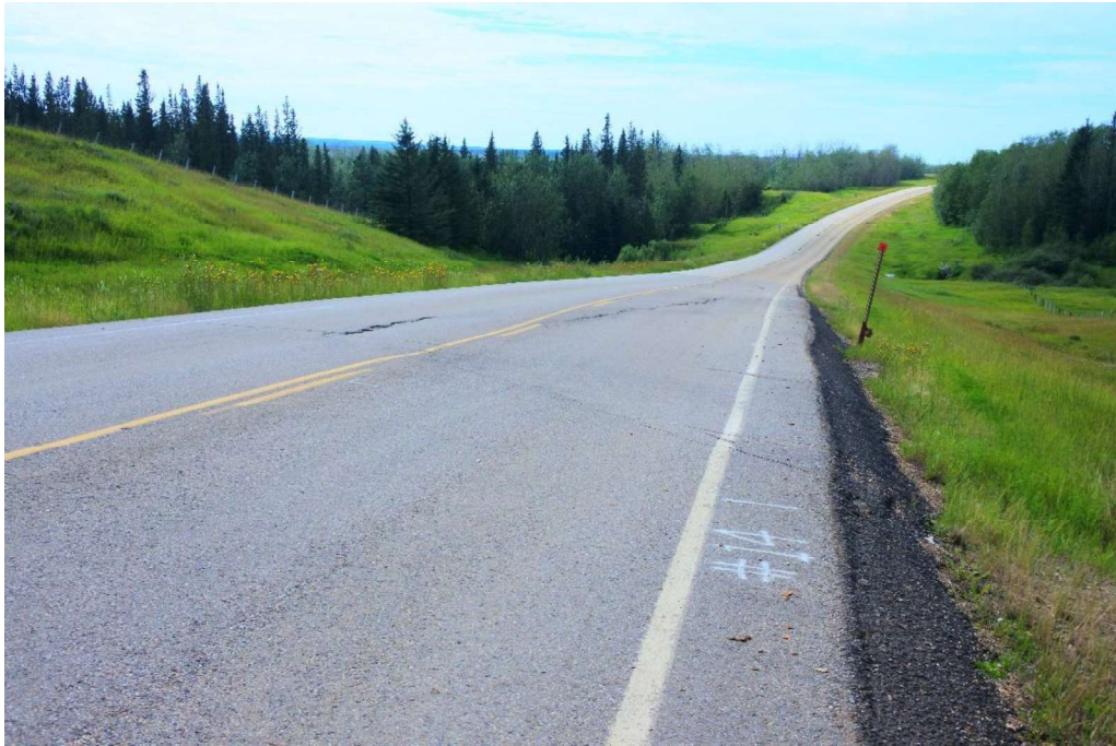
Photo 1 – Looking south at main crack and dip in highway surface. Significant thickness of asphalt visible at the edge of the pavement.
