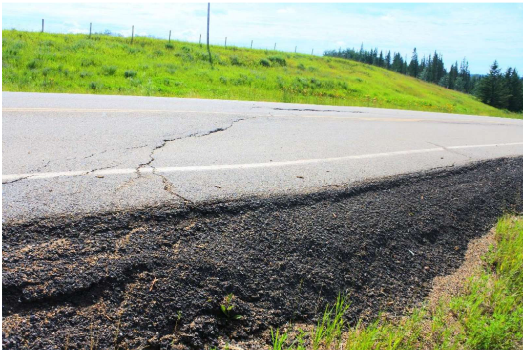
Photo 4 – Looking southeast at north end of crack pattern and several layers of ACP patches.
