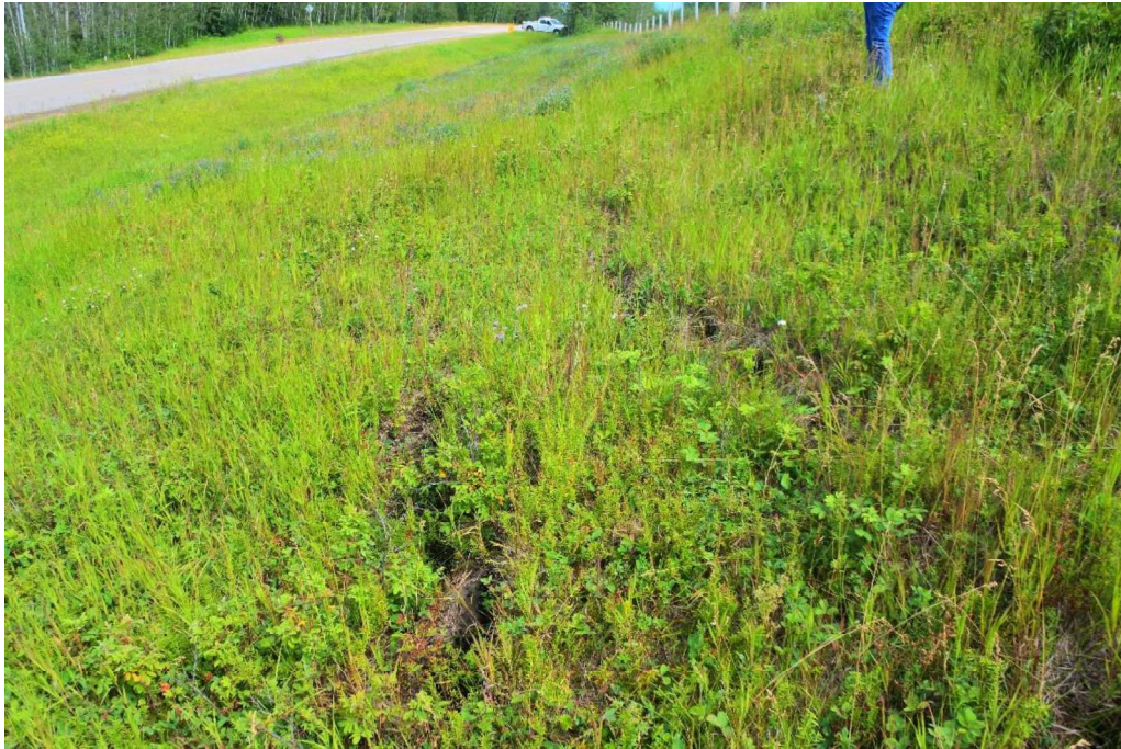
Photo 11 – Looking north at slumping backslope below power pole with open tension cracks.
