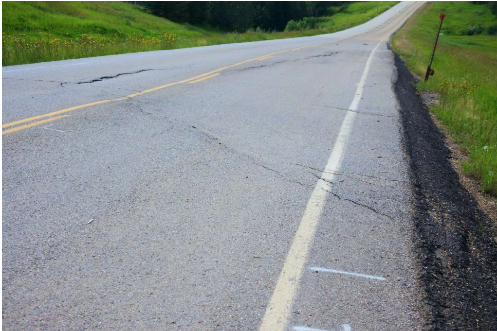
Photo 3 – Looking south at differential across crack.
