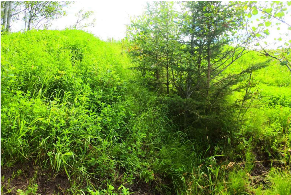
Photo 6 – Looking east at erosion gully forming on north side of toe berm (west of the highway).
