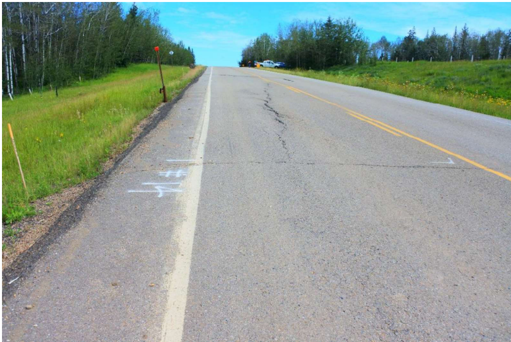
Photo 2 – Looking north at main crack and dip in highway surface.
