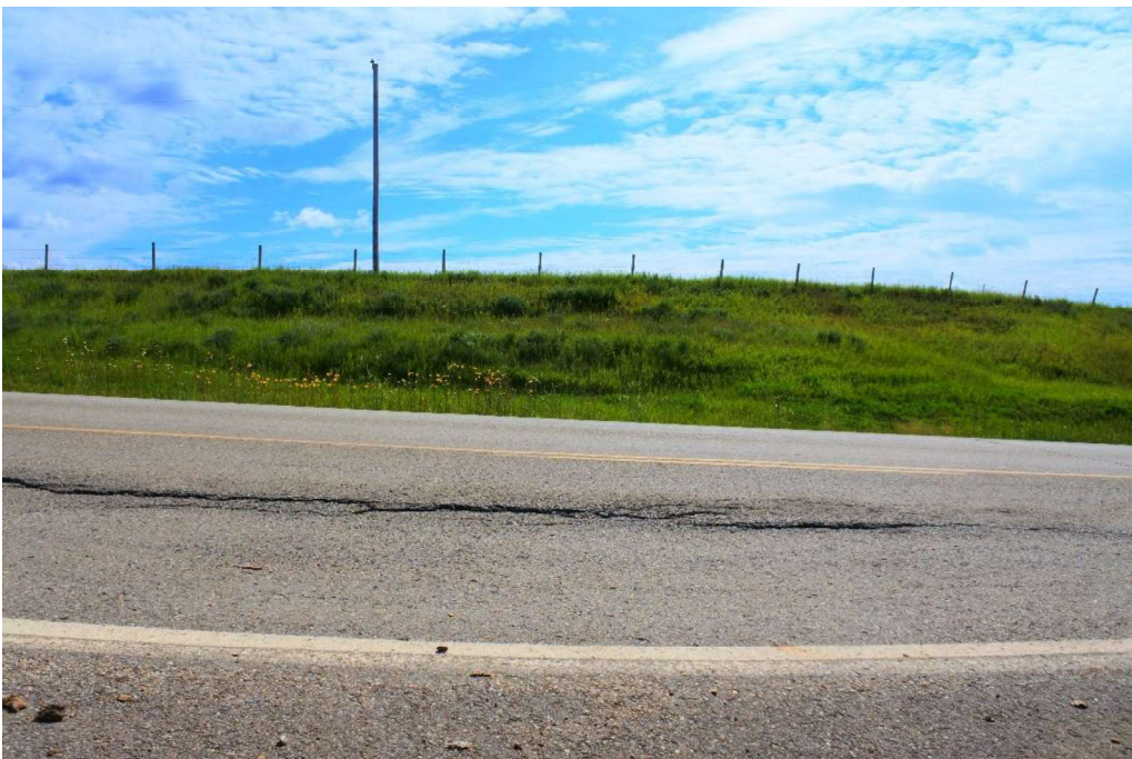
Photo 10 – Looking northeast at backslope slumps just south of the power pole.
