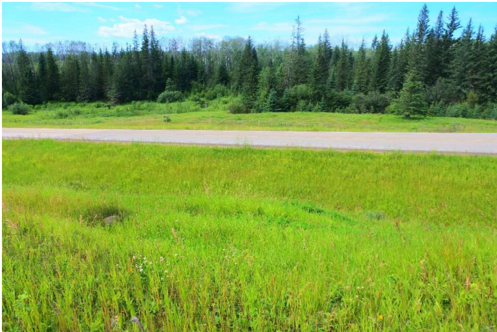
Photo 12 – Looking west from the backslope at the subsiding area in the pavement.
