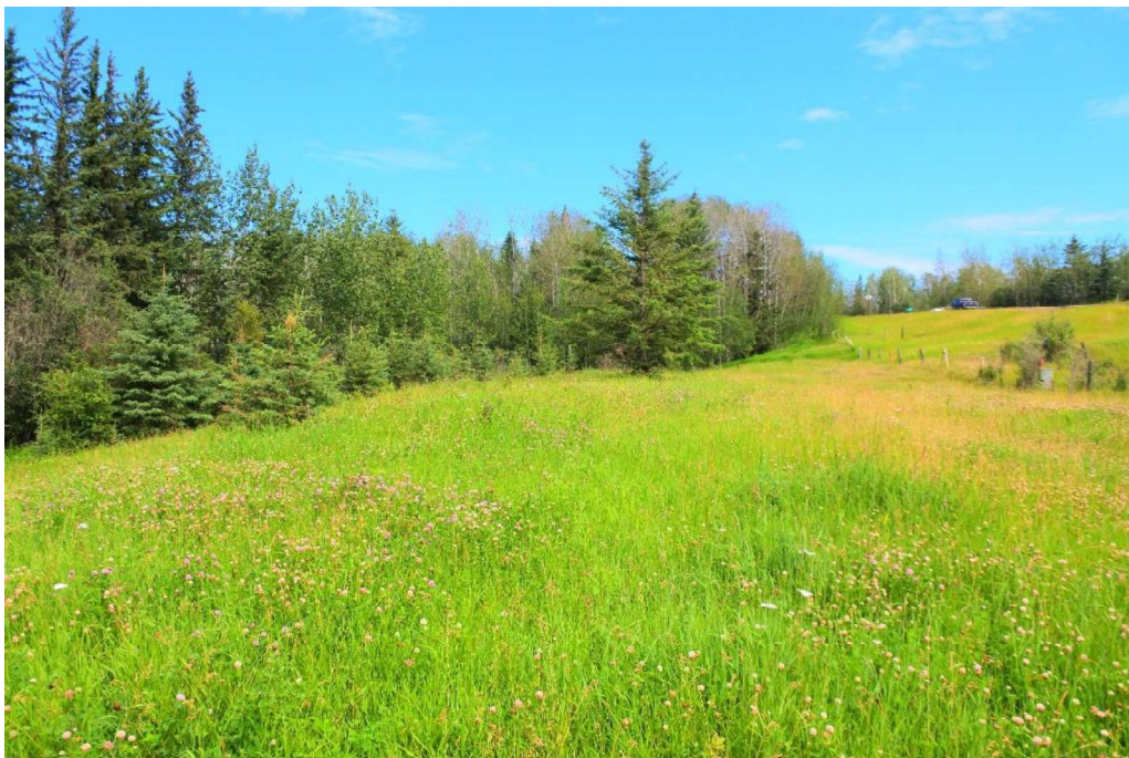
Photo 8 – Looking northeast along the top of the back-tilted toe berm and leaning fence
